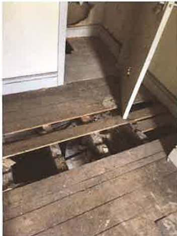
Fig 5 Missing Floorboards to Unit 2 Replace
