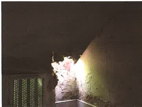
Fig 23 Damaged roof to Unit 6 Reroof lean to at rear
