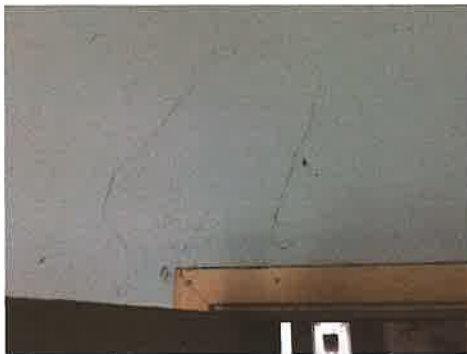
Fig 10 Cracking over GFL door to Unit 2 Replace lintels in concrete
