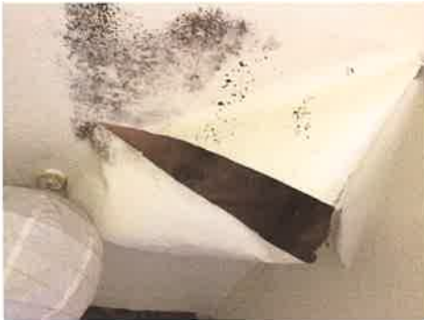
Fig 14 Roof leak to Unit 3 Repair roofing
