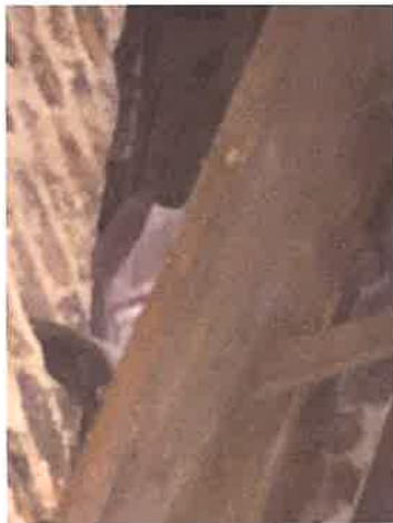
Fig 9 Damaged felt to Unit 2 Repair
