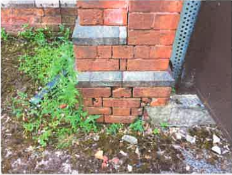
Fig 13 Damaged pointing to Unit3 Repoint
