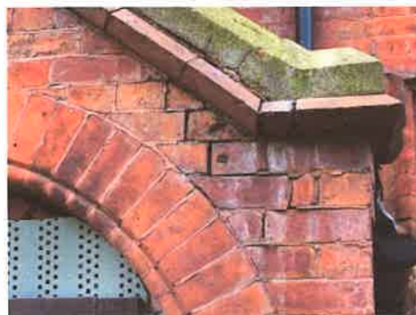
Fig 12 Damaged brickwork to Unit 4 Rebuild
