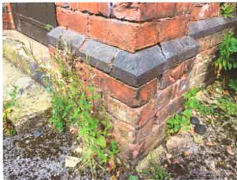
Fig 30 Poor quality pointing to Unit 1 Repoint
