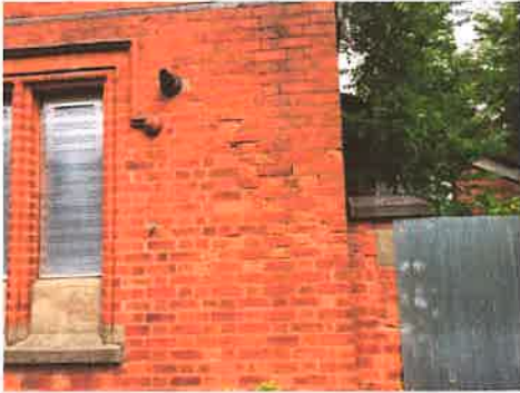
Fig 28 Perished bricks to Unit 1 Replace and repoint
