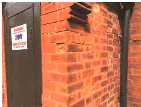
Fig 31 Perished bricks to Unit 1 Replace
