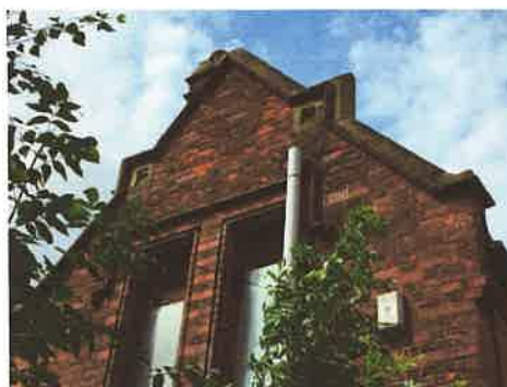
Fig 24 Perished brickwork to rear pediment of Unit 6 Replace perished bricks
