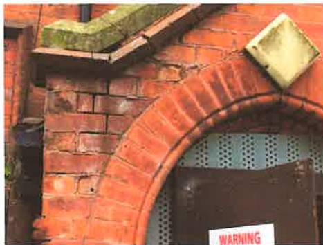
Fig 11 Damaged brickwork to Unit 3 Rebuild
