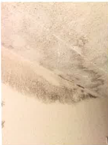
Fig 7 Damp To Unit 2 ceiling Check roof flashings etc
