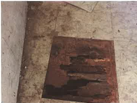
Fig 22 Rotten floor boards to Unit 6 Replace boards and check joists
