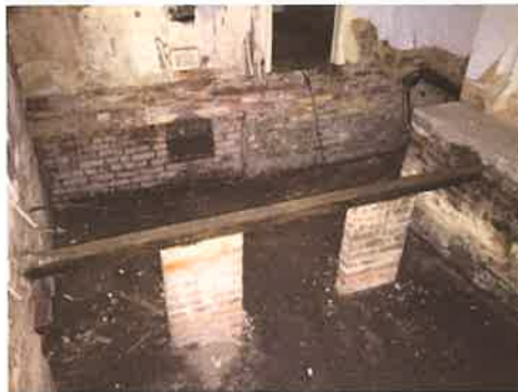
Fig 16 Missing floor joists to Unit 4 Replace joists
