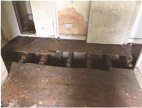
Fig 21 Missing floorboards to Unit 6 Replace
