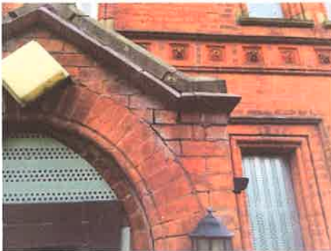
Fig 26 Damaged brickwork and copings to Unit 6 Rebuild
