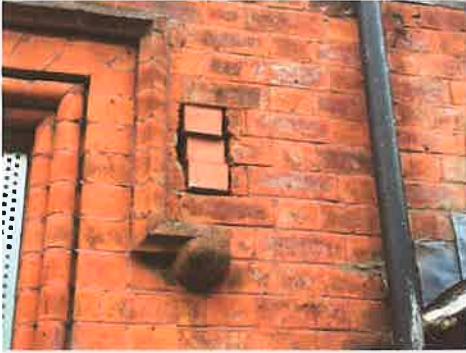
Fig 25 Missing bricks to Unit 6 Replace
