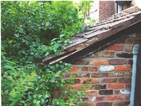
Fig 27 Tiles missing to lean to roof of Unit 6 Replace lean to roof
