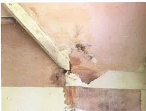
Fig 8 Damp To Unit 2 ceiling Check flashings
