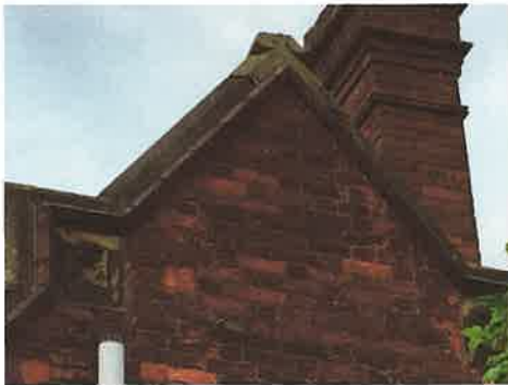
Fig 29 Copings slipped to Unit 1 Refix generally with stainless steel fixings
