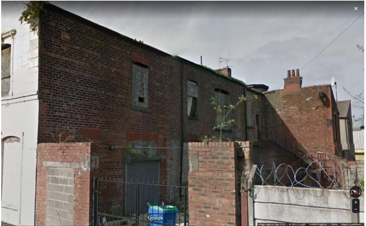
Figure 1.7: Google Street View, as at April 2016, showing the derelict state of the rear elevation of the application premises.
