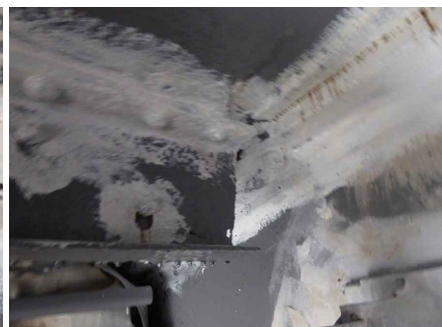
IMAGE 4 - PFC SUPPORTING DECK PLATES CORRODED AWAY, PFC TORN IN LOCATION OF THE FIXINGS TO BACKING PFC LARGE CRACK IN DECK PLATE.
