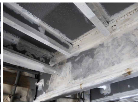
IMAGE 2 - PFC SUPPORTING DECK PLATES CORRODED AWAY MINOR CRACK IN DECK PLATE.
