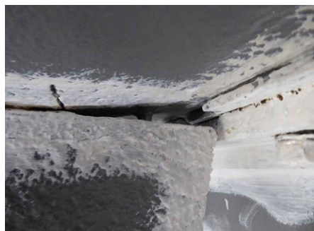
IMAGE 3 - LARGE CRACK IN DECK PLATE.
