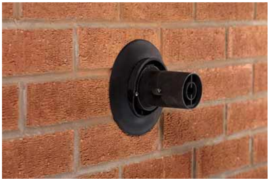
Boiler Flue Wall Penetration
