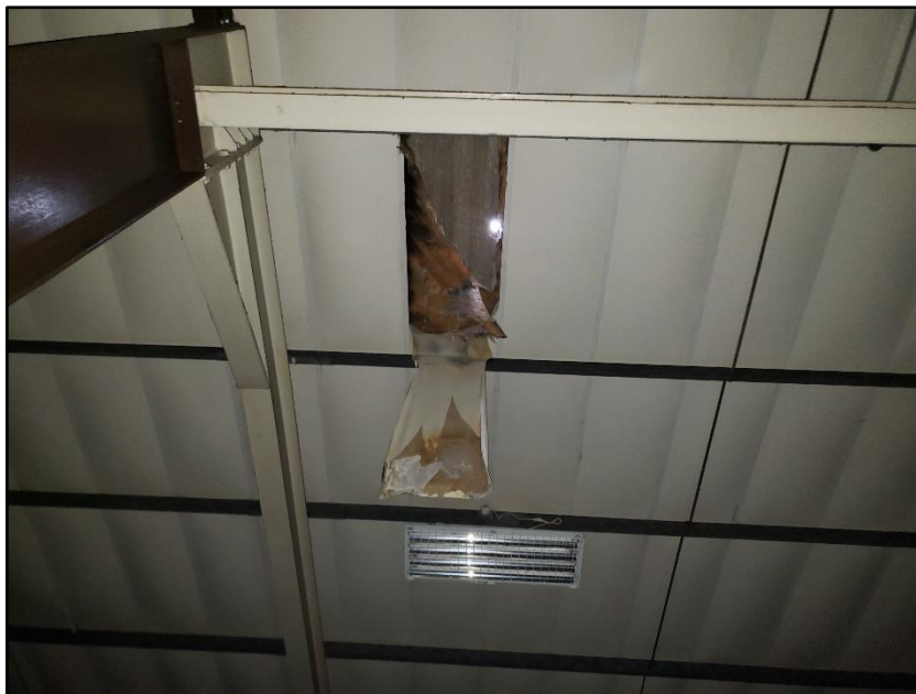
Photograph 7 showing a damaged roof panel
