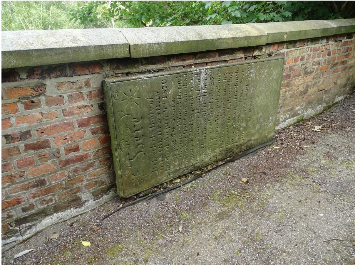
Photo 5: Existing Headstone positioned against parapet wall section that requires rebuilding.
