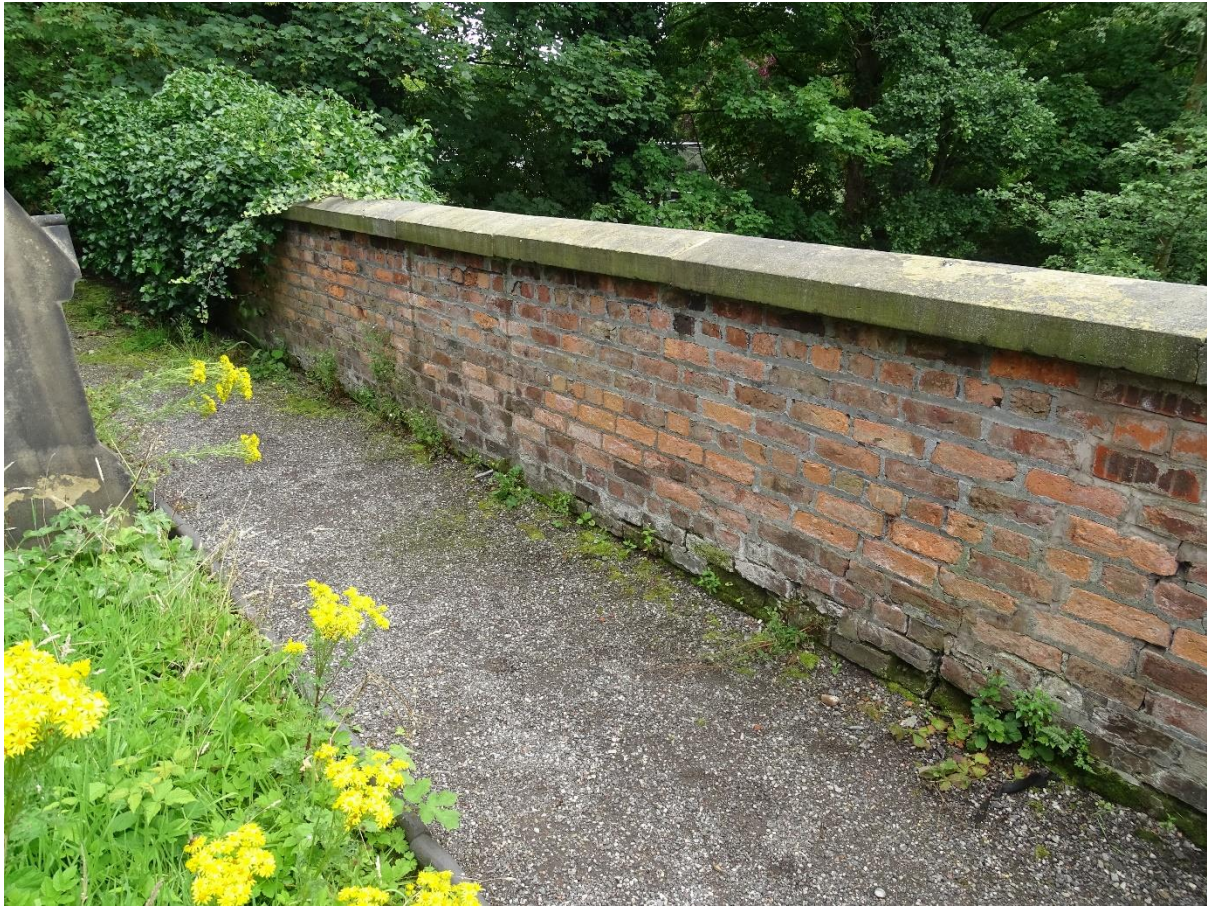
Photo 11: Section of parapet wall to be repaired and repointed.
