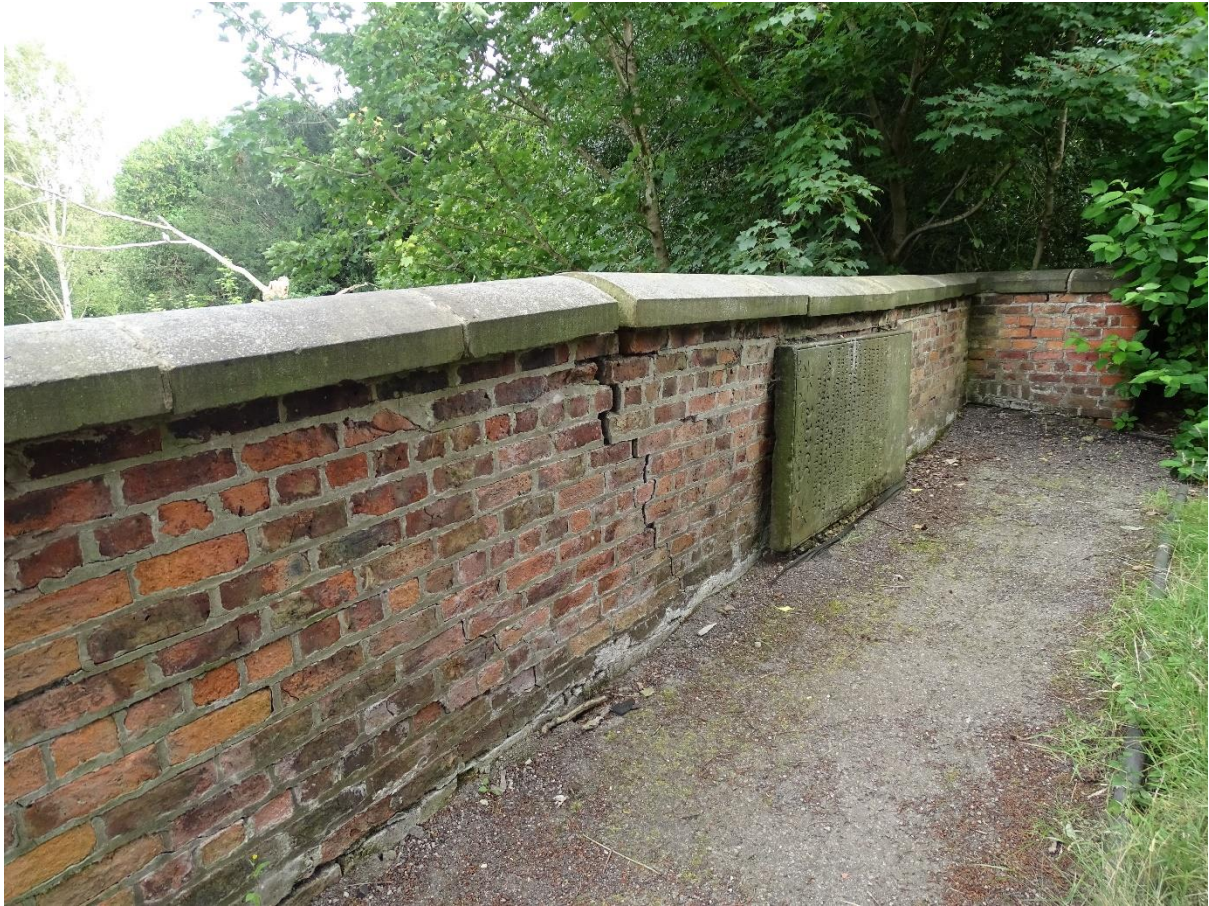
Photo 2: Parapet wall section to be rebuilt to best match existing.
