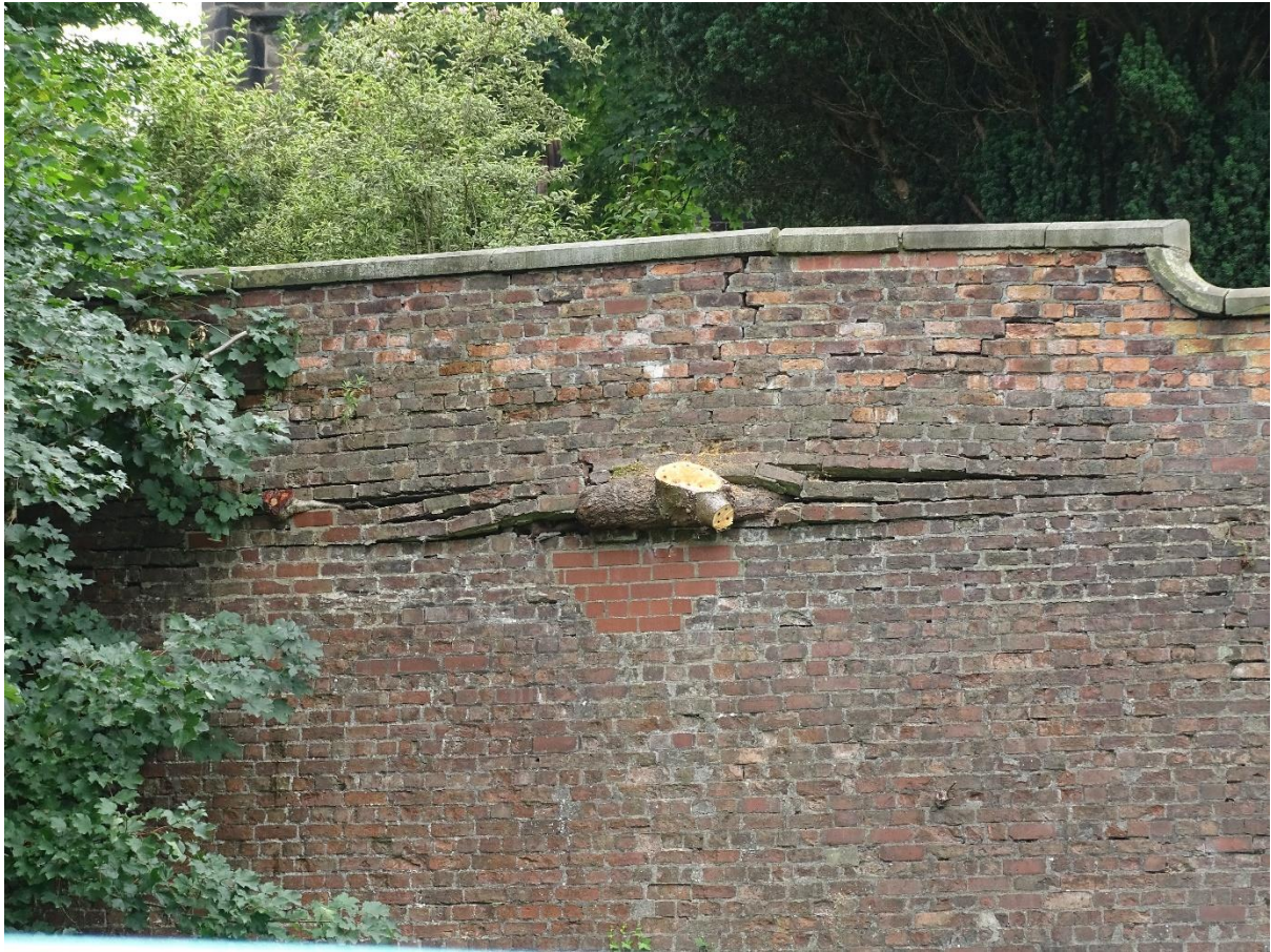
Photo 3: Remains of the Goat Willow stump to the joint of the parapet / retaining wall.
