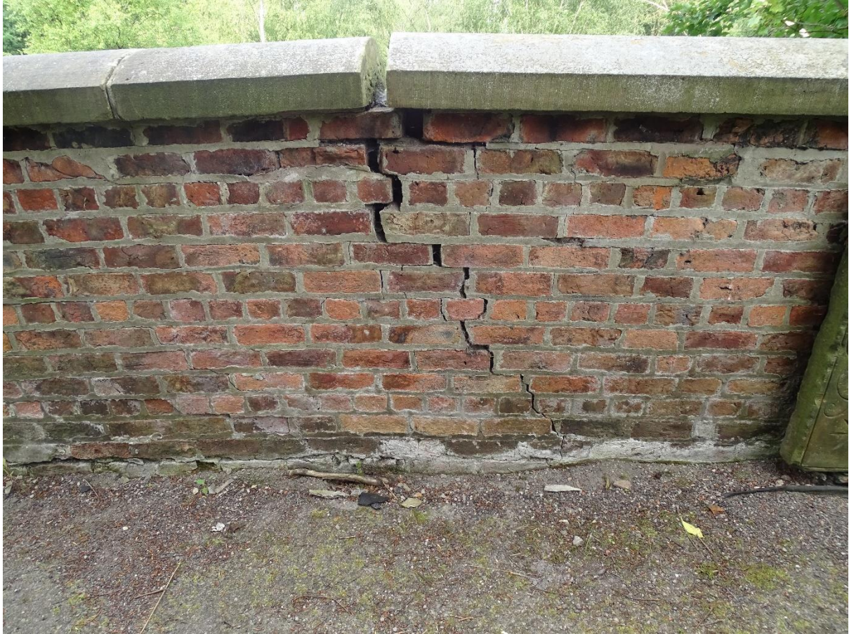
Photo 1: St James Church cracking to Parapet Wall damaged by growth of Goat Willow.
