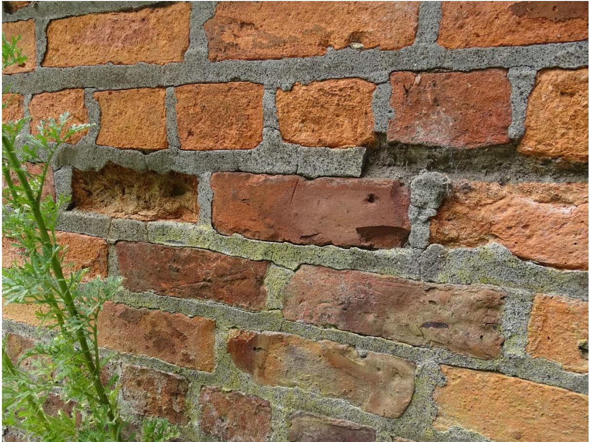
Photo 13: Existing parapet wall condition, showing spalling brickwork and loose pointing
