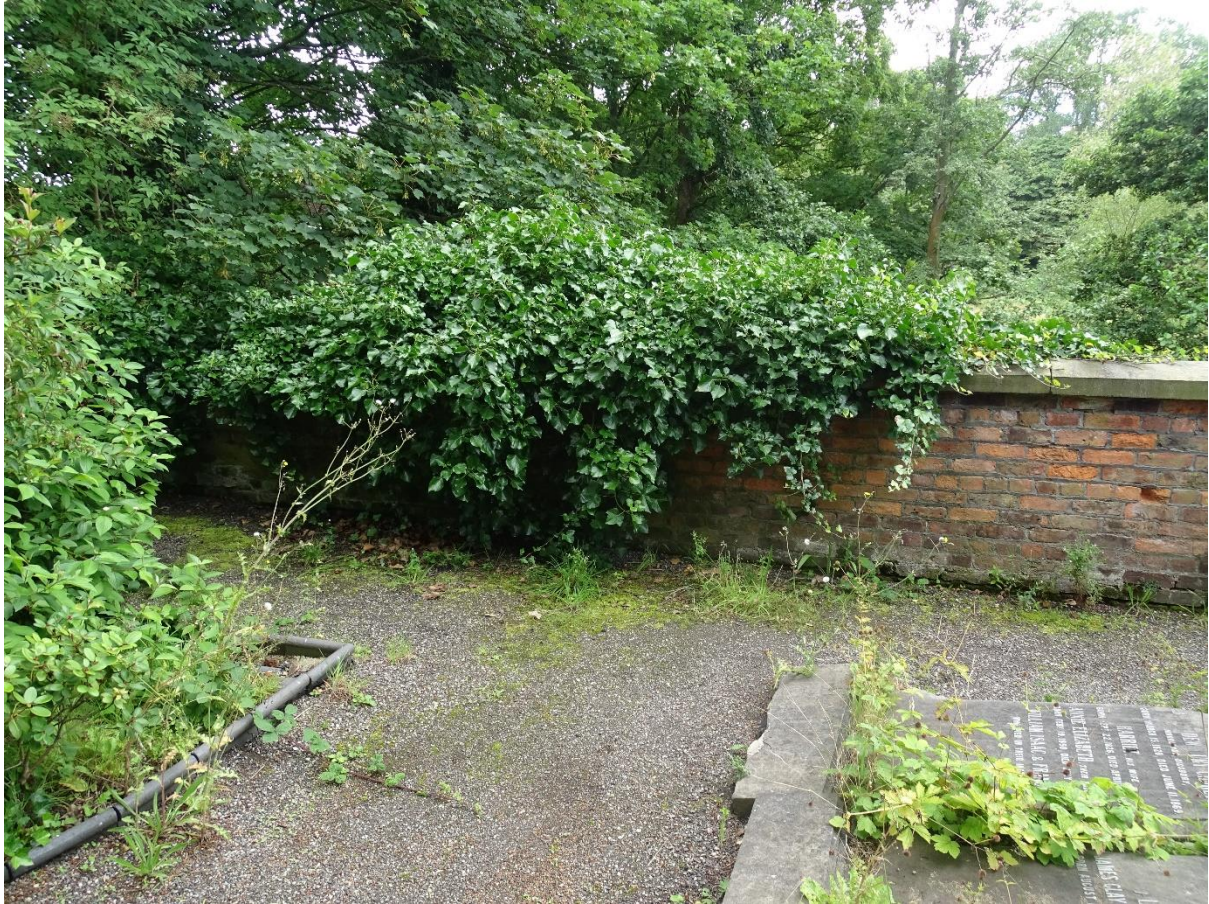
Photo 10: Vegetation overgrowth that requires removal from both sides of wall.
