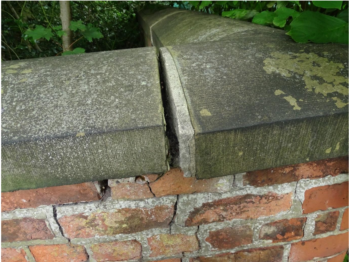
Photo 14: Existing coping stone joint.
