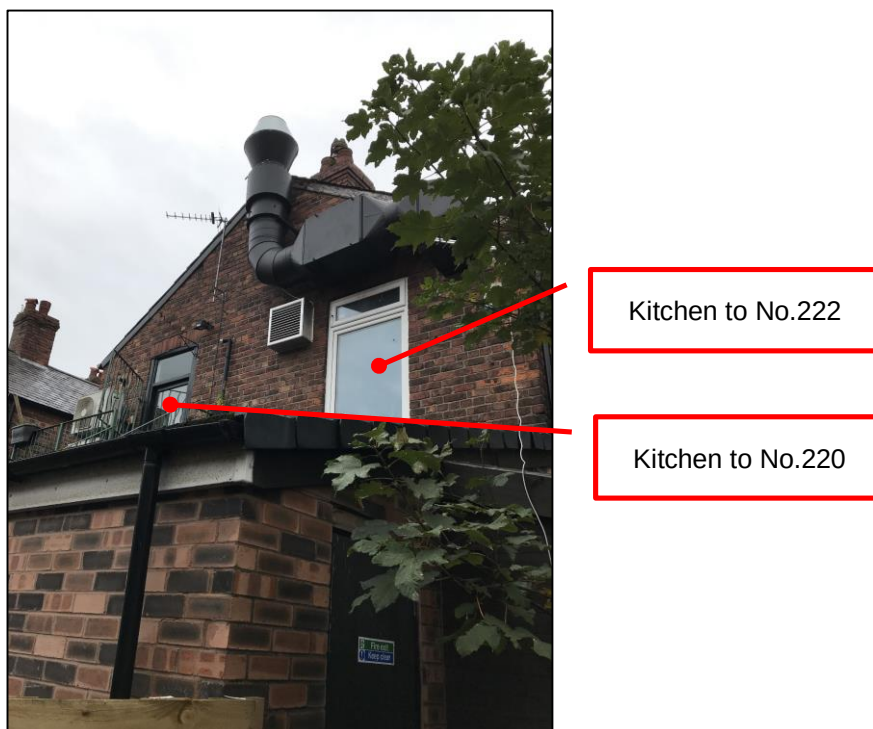
Figure 4.1 – Photograph showing kitchen extract ductwork and flue
