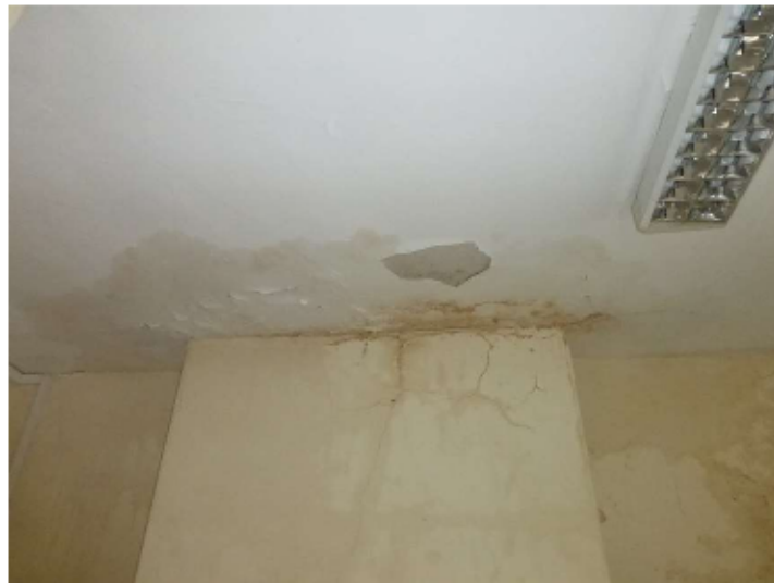
Dampness on 1 st floor ceiling at chimney breast
