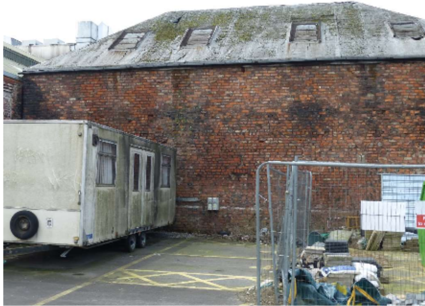
Rear roof to production building. Note loss of pointing to brickwork.
