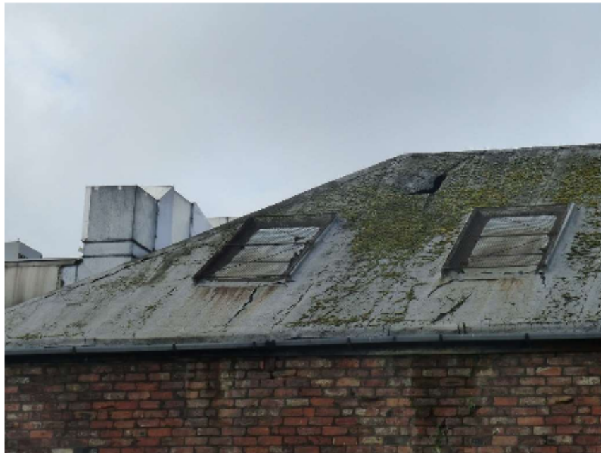
Enlarged view on some holes in the roof and roof coverings
