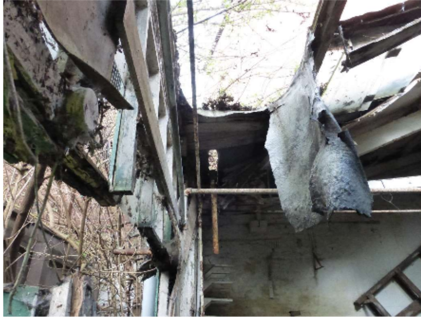
Partially collapsed roof and wall to the lean-to building
