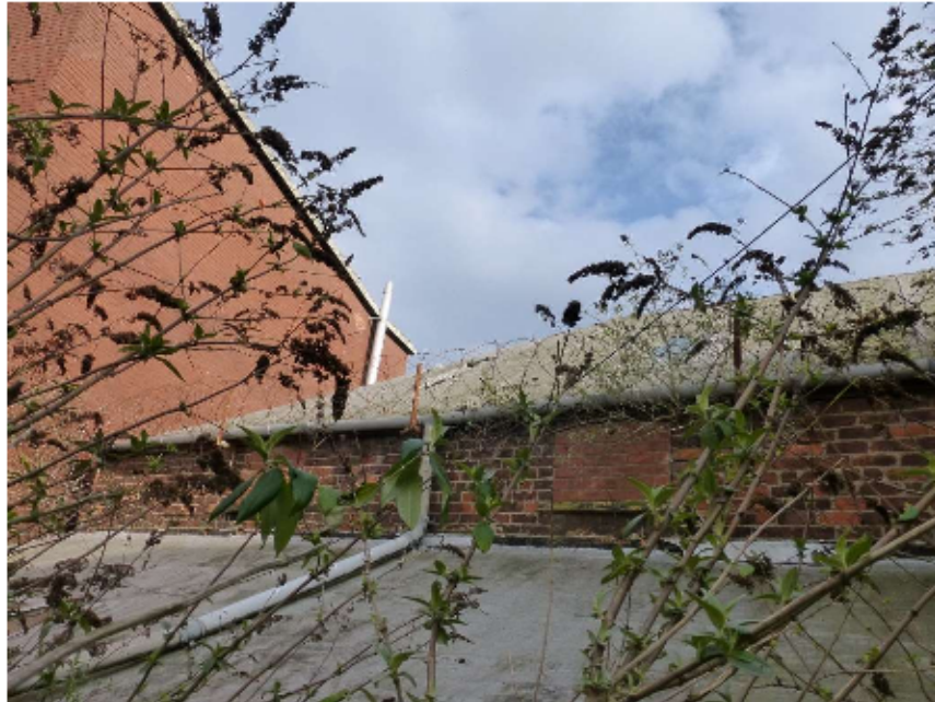
Main production building roof viewed from behind lean-to building. Note sagging of lean-to roof where it joins main building wall
