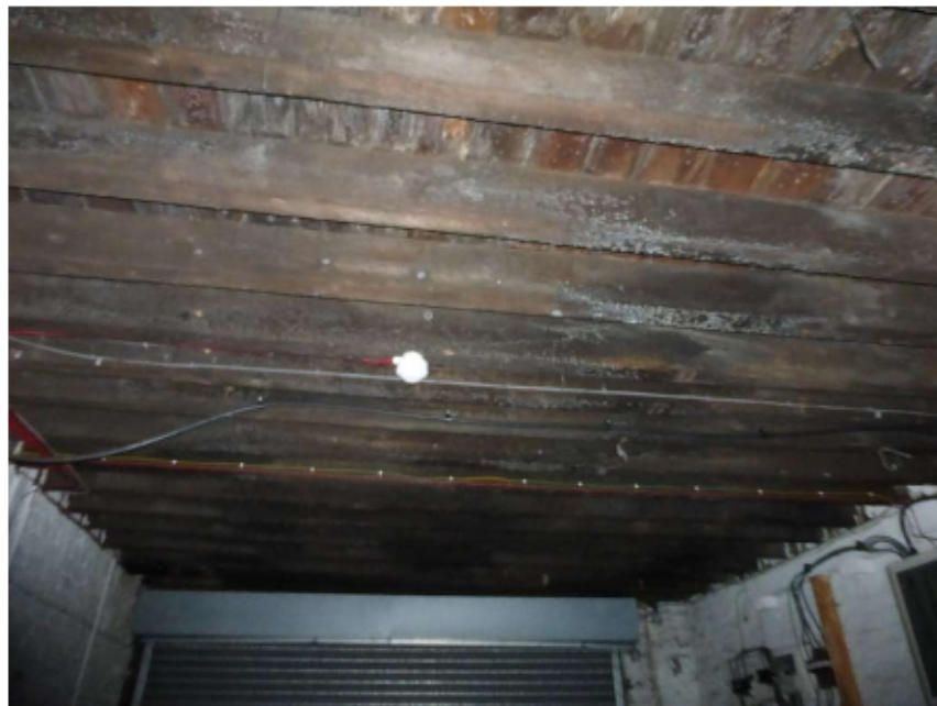
Dampness and mould spores on underside of 1 st floor over access
