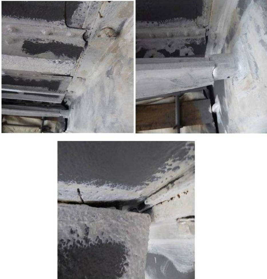
Image of broken deck plates (network rail photographs)
