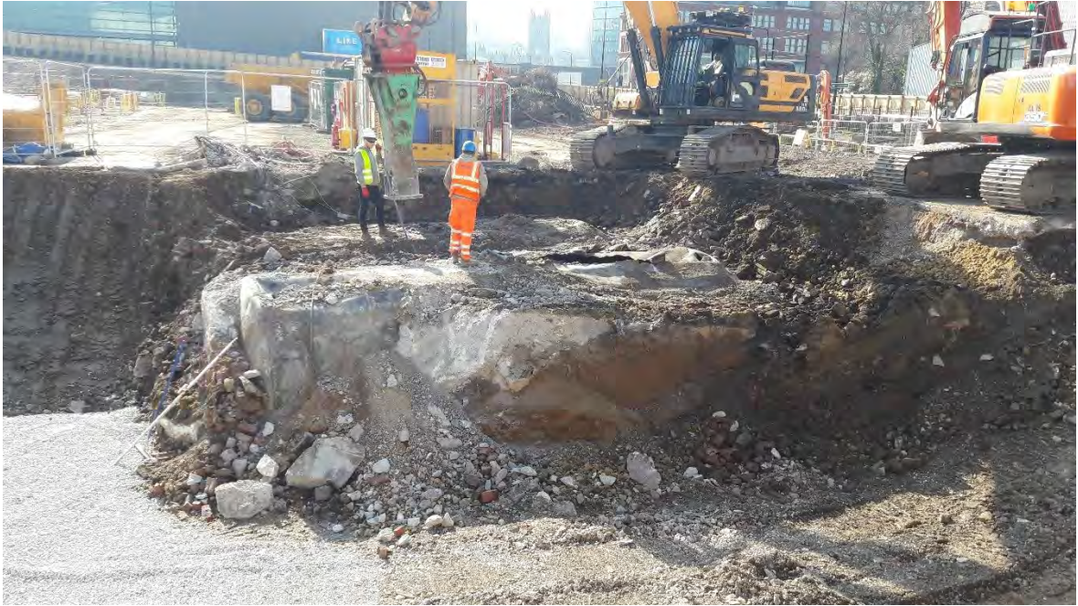
Underground storage tanks with concrete surround.
