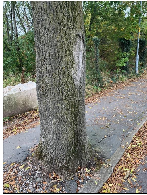
Plate 2: T1 close-up of occluded wound and pavement heave.
