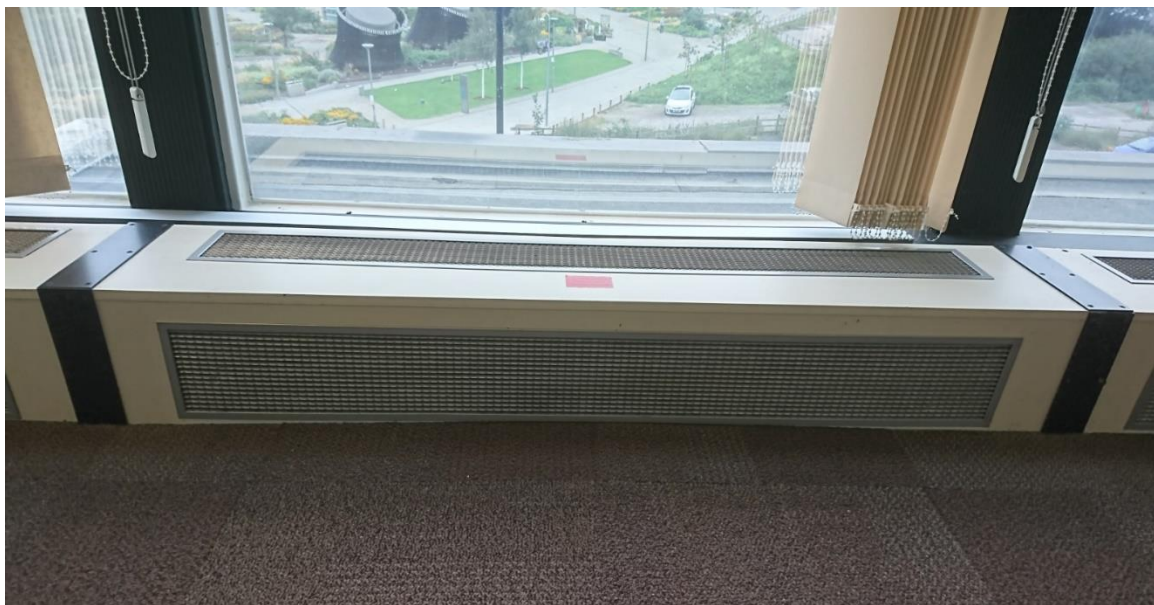
02.07 Example of the redundant Weathermaster, perimeter air-conditioning unit.
