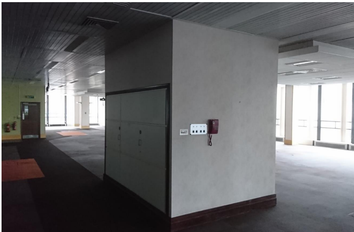
02-21 Detail of the inserted IT plant rooms in the podium office.
