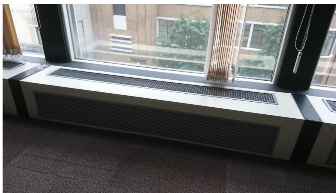
02-18 Example of the Weathermaster air-conditioning system in the podium.
