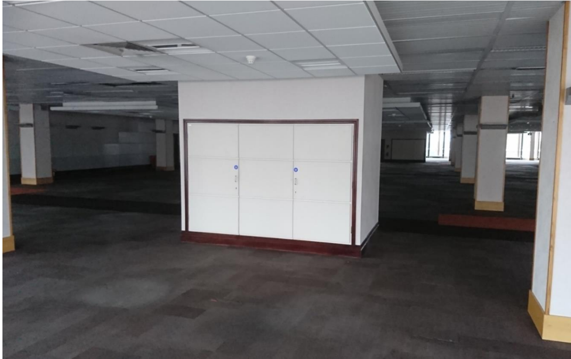
02-20 Example of one of the inserted IT plant rooms in the podium office.
