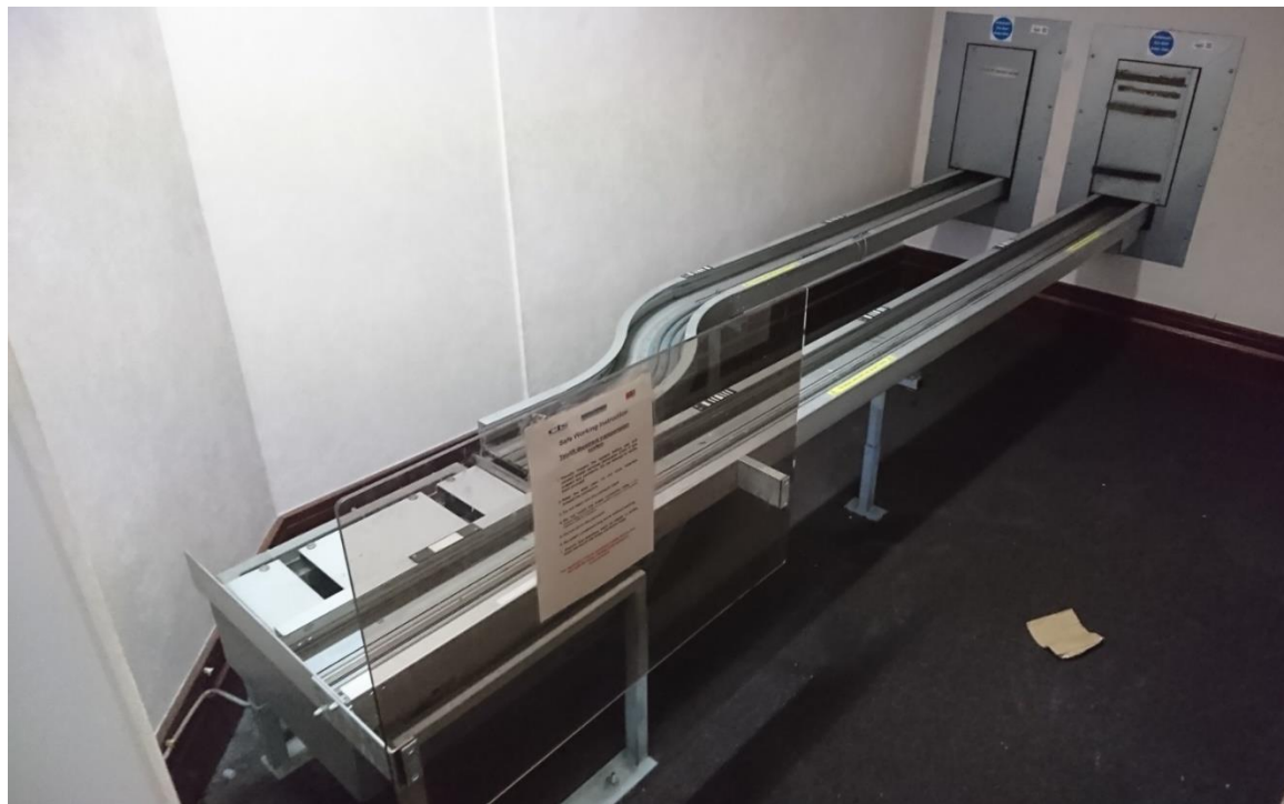
02-11 Details of the double-track Telelift document distribution system (see also section 4.4 above)
