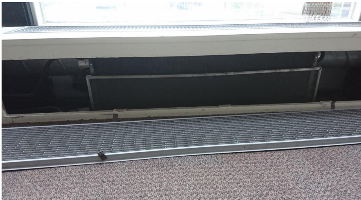
02-25 Example of the Weathermaster ductwork and system (see also Section 4.3)
