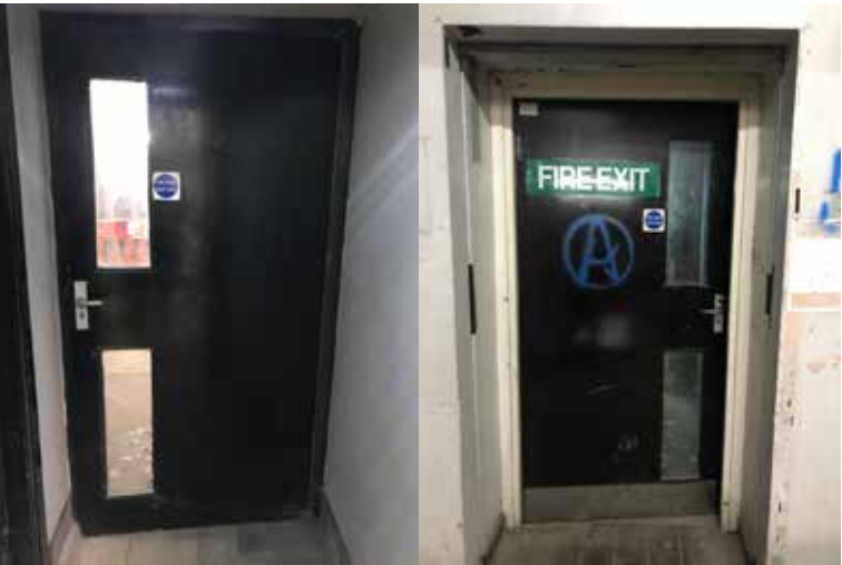
Fire door from lobby to B2 corridor space
