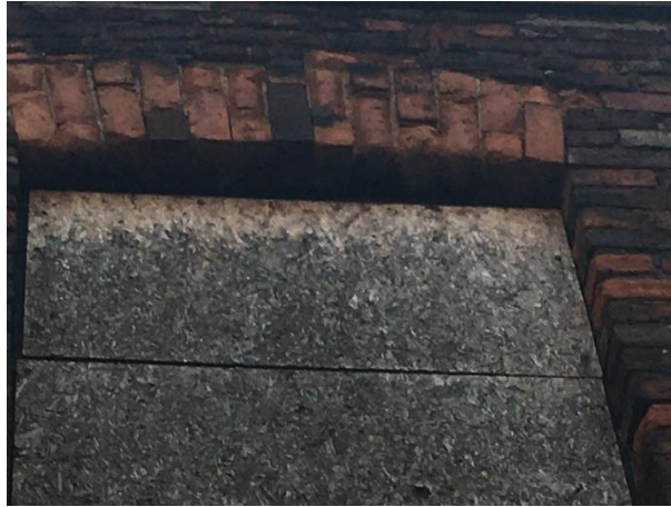
PLATE 5 SHOWING CREVICES LOCATED WITHIN BOARDED WINDOWS
