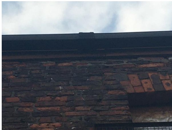
PLATE 6 SHOWING WOODEN FACIA BOARDS
