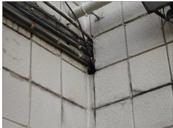
Plate 30. Showcase Cinema (gap in the external wall)
