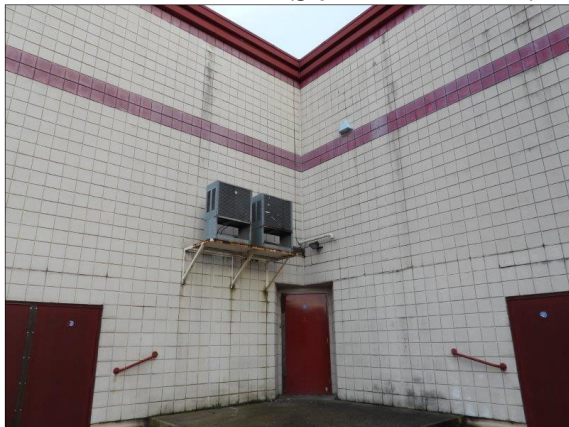
Plate 29. Showcase Cinema (gap in the external wall)
