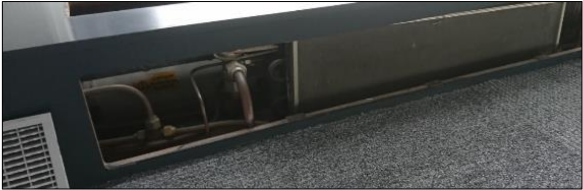
Figure 28. Example detail of the interior ductwork.
