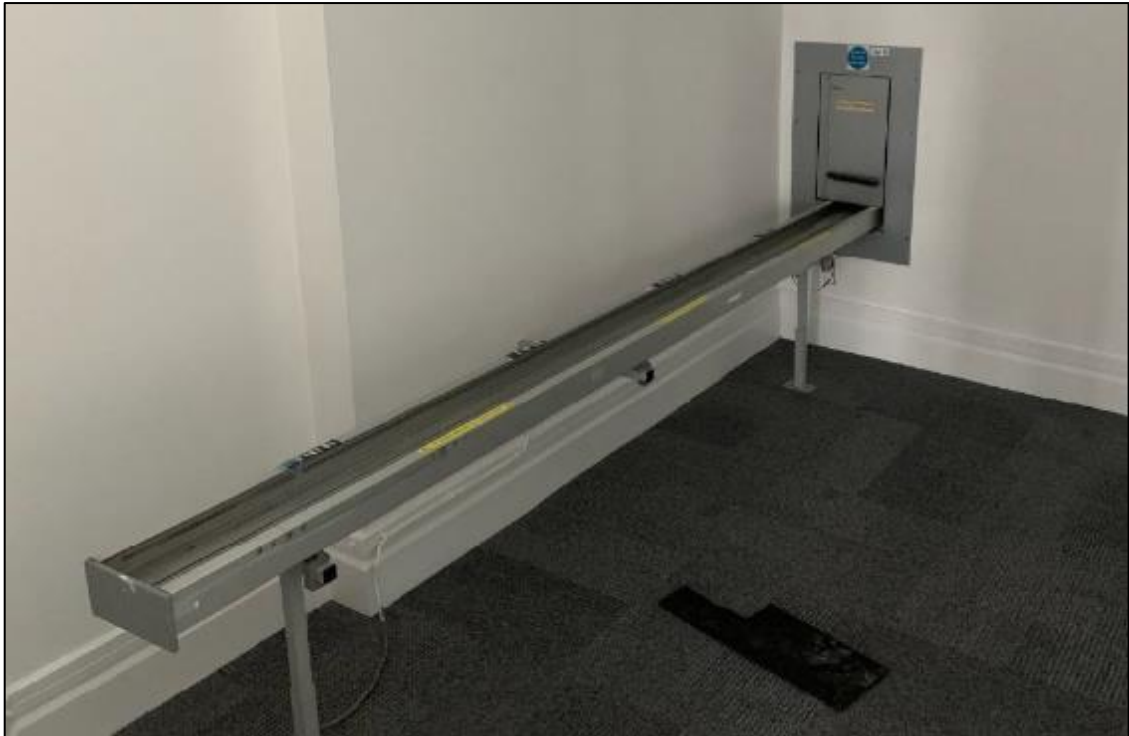
Figure 36. An example of the office-side single track system on the 15 th tower floor, showing the entrance to the riser and vertical distribution.
