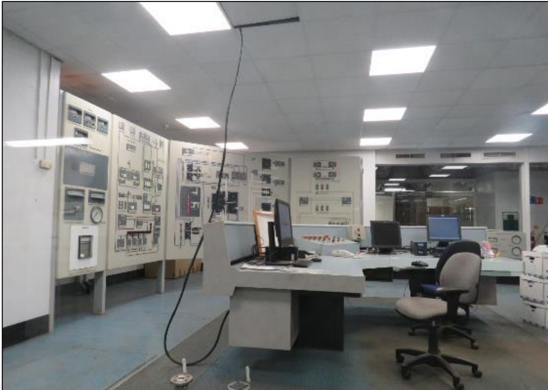
Figure 31 View of the basement control room (level B2). Note the original control equipment has been removed and replaced.
