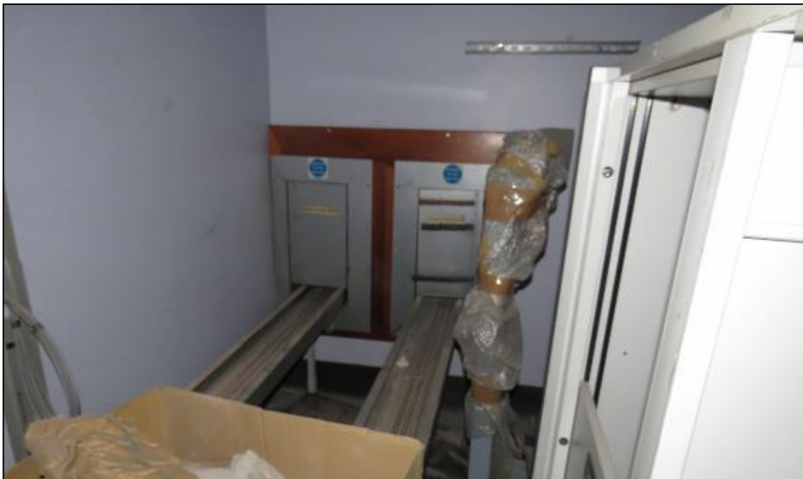
Figure 35. The connection to the former post-room showing the connection to the riser which runs through the tower. The system has been redundant for some years.
