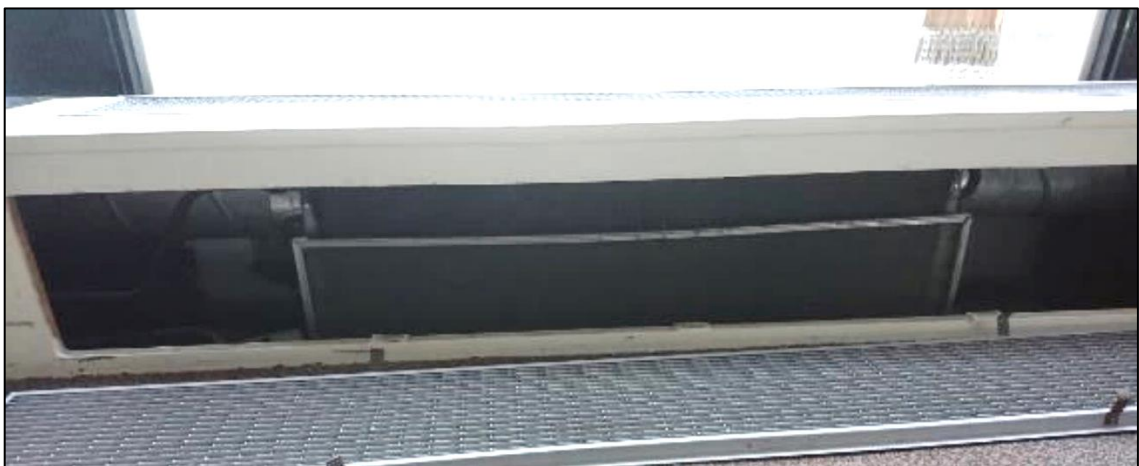
Figure 27. Example view of the interior of the system showing the ducting.
