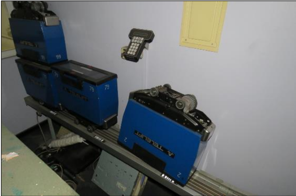
Figure 34. The document transportation units (Ground-floor post-room) showing the drive mechanism.
