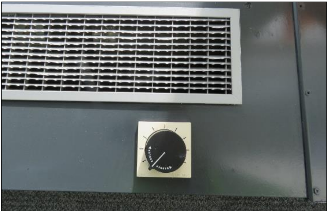
Figure 30 Detail of the simple adjustment control for each floor level. The main system controls were in the basement.
