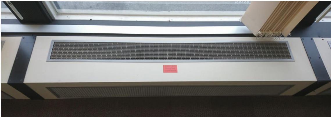
Figure 29 Details of the top of the perimeter air-conditioning system.
