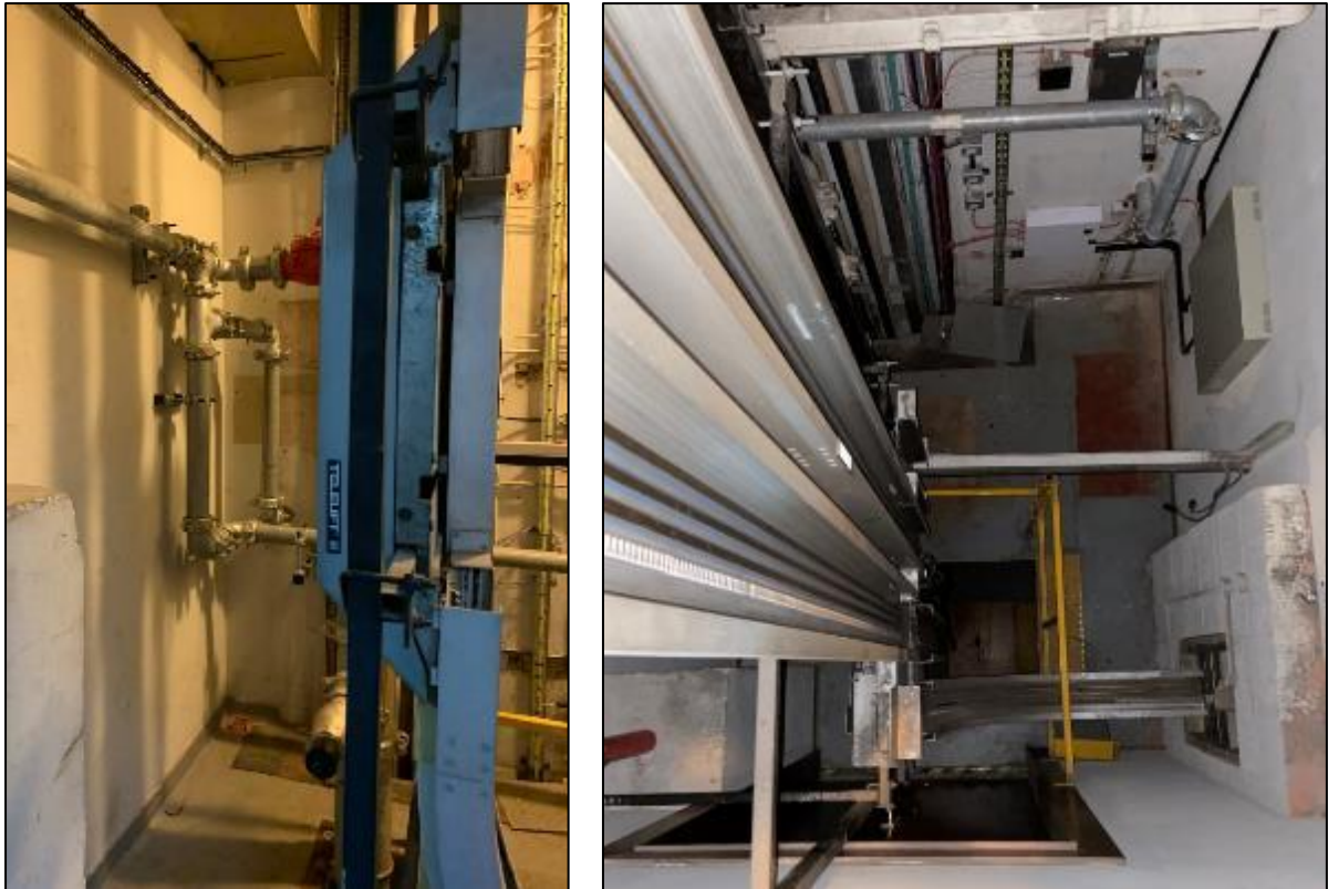
Figure 40. Views within the vertical riser showing the Telelift mechanism (left side) and the route of the document movement system which connected each office floor in the tower offices (right hand side).
