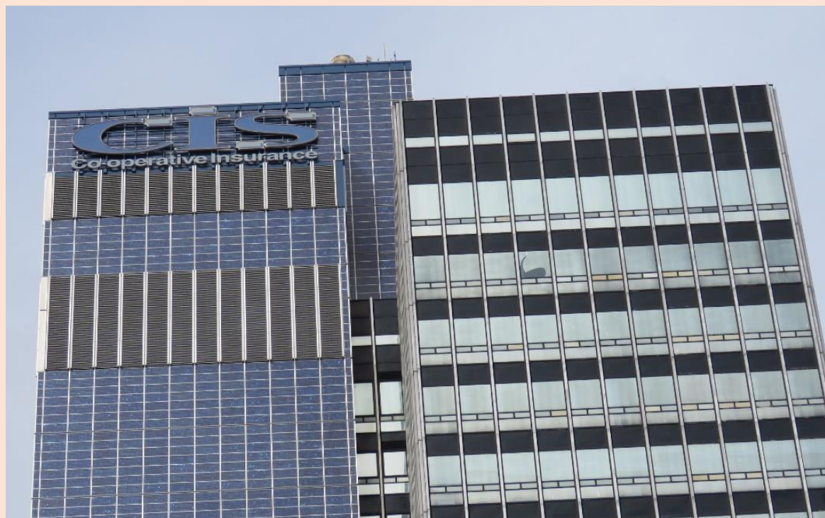
RS-10 Details of the top of the service and office towers from the Riga Street car-park, showing the non-original signage, photovoltaic panels and failing film applied to the glazing.
