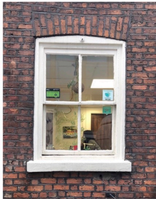
WINDOW W.01 EXISTING SLIDING SASH WINDOW BEYOND SERVICABLE CONDITION
