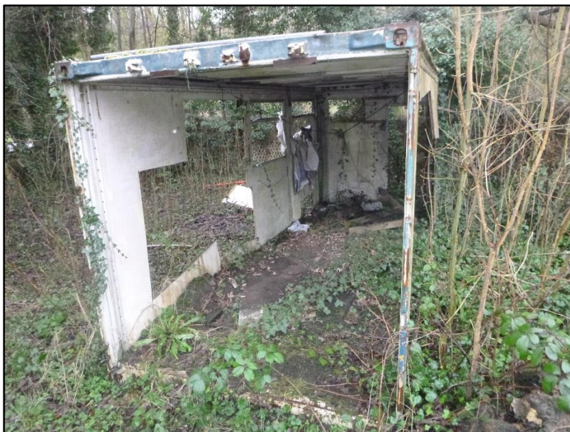
Photograph 5 showing the damaged container on site
