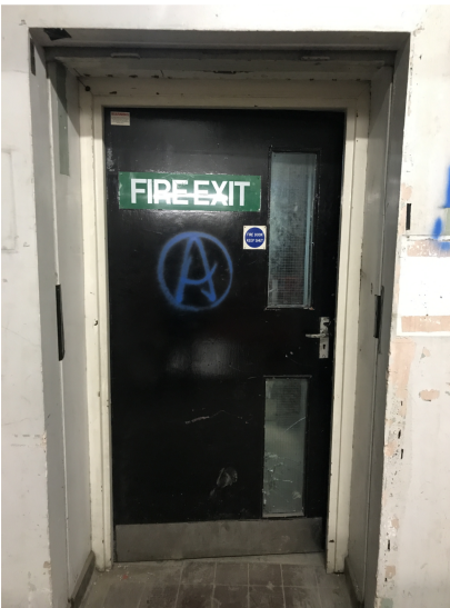
Existing non-compliant fire door to be replaced
