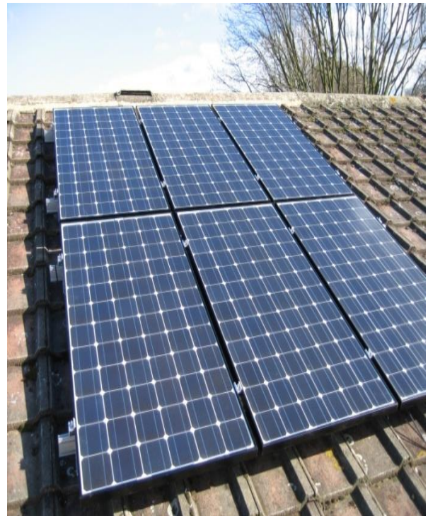
Figure 4 - Photovoltaic array on a pitched roof
