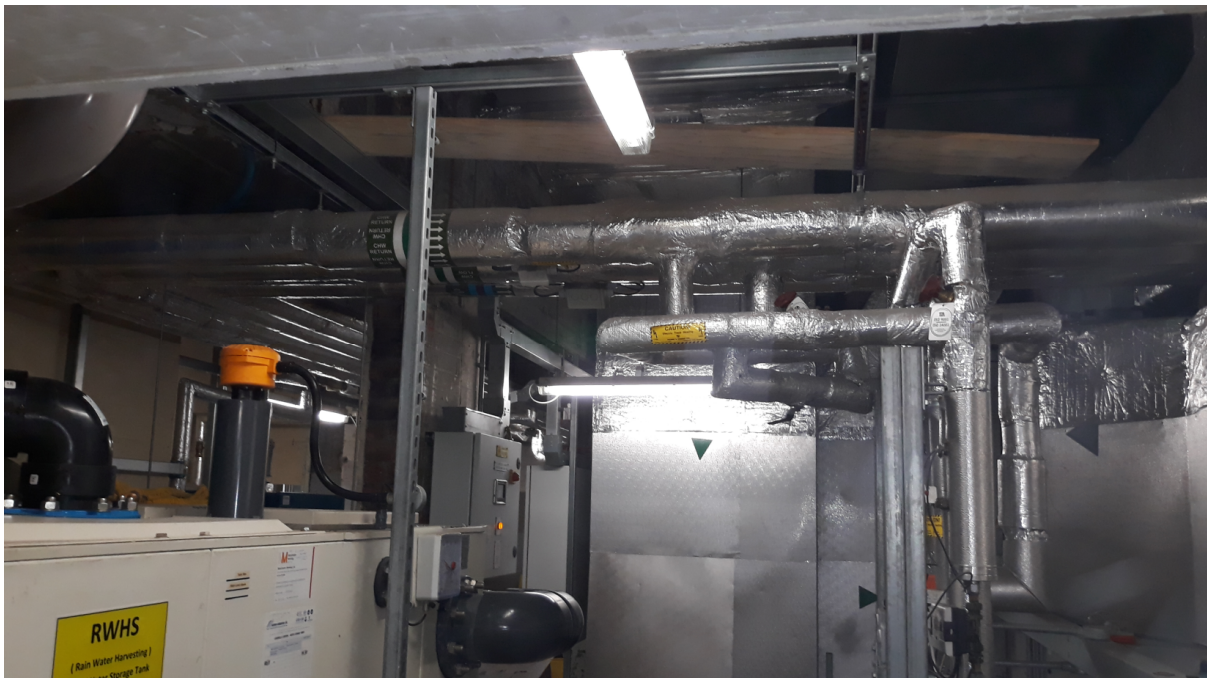
Basement plantroom HV cable ladder route adjacent existing services
