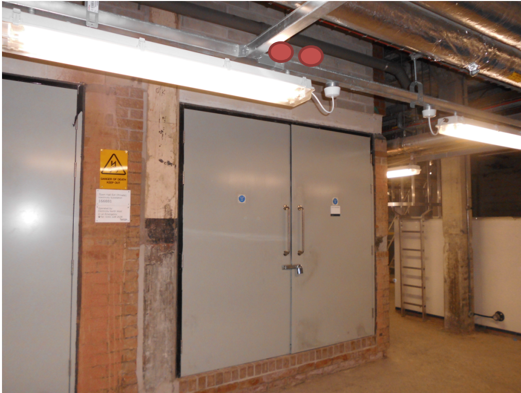
Existing RMU transformer room switchroom cable ladder entry position above double door through existing blockwork wall
