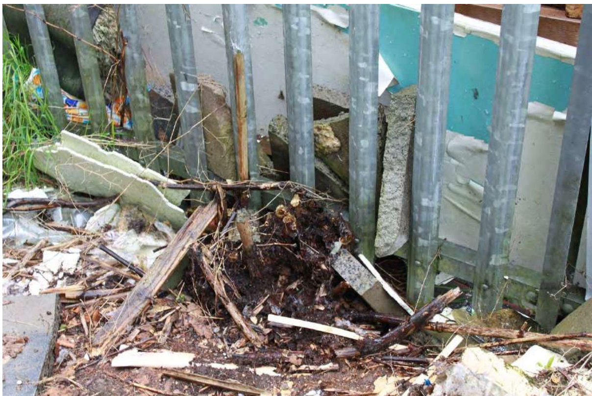
Photo 8 - Crown visible at boundary with 18 Ellen Wilkinson Crescent
