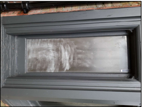
P83 - View of opening to bay window of Room A0/37. Polycarbonate to be removed and replaced with hand drawn glass.
