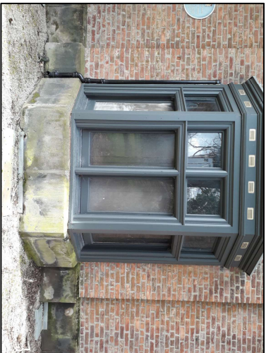
P82 - View of bay window to Room A0/37. No. 4No. larger openings have been fitted with polycarbonate glazing.
