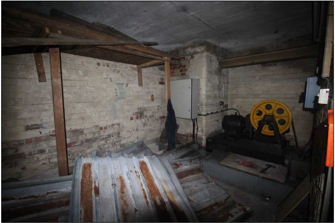
Plate 62: The lift winding gear room
