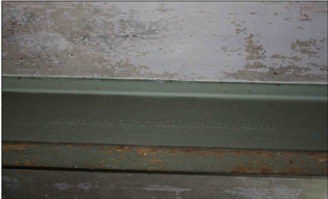
Plate 31: The rolling stamp of Dorman Long on the steel beams and columns used in the construction of the warehouse and attached office/warehouse block
