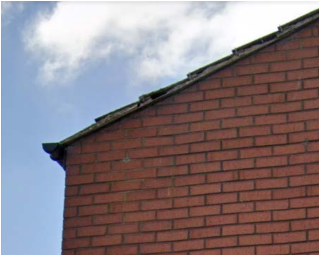
Figure 13: Gaps in mortar on edge of roof on Building 2
