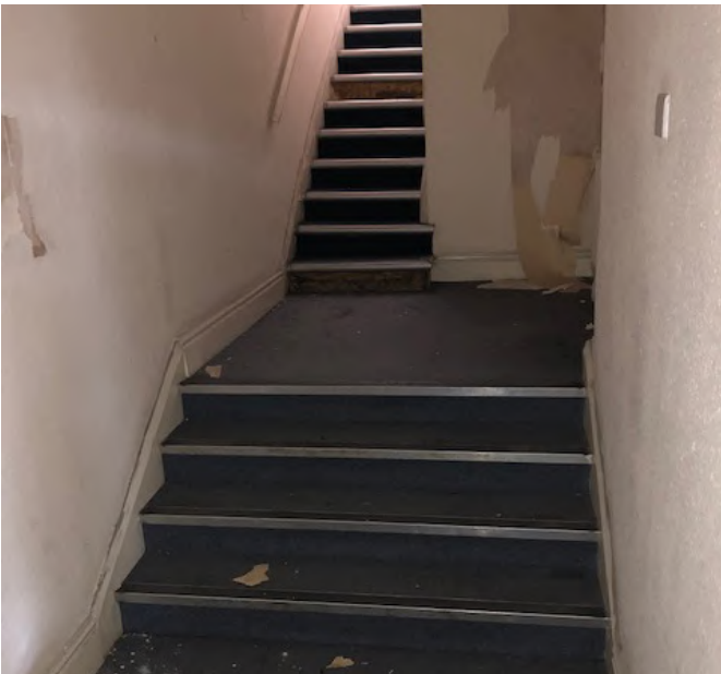
5: All staircases not original
