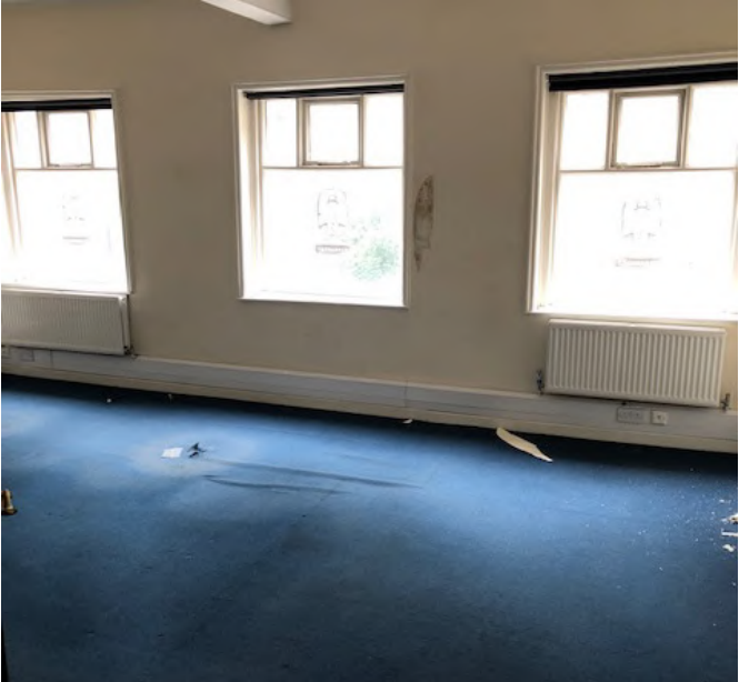
2: Radiators not original, no secondary glazing
