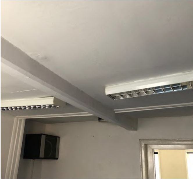
3: Plastered ceiling, no coving
