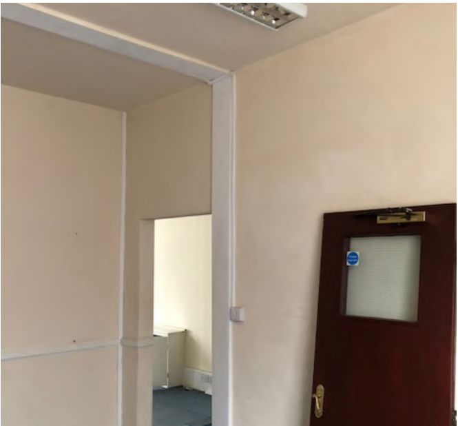
12: No coving on this floor
