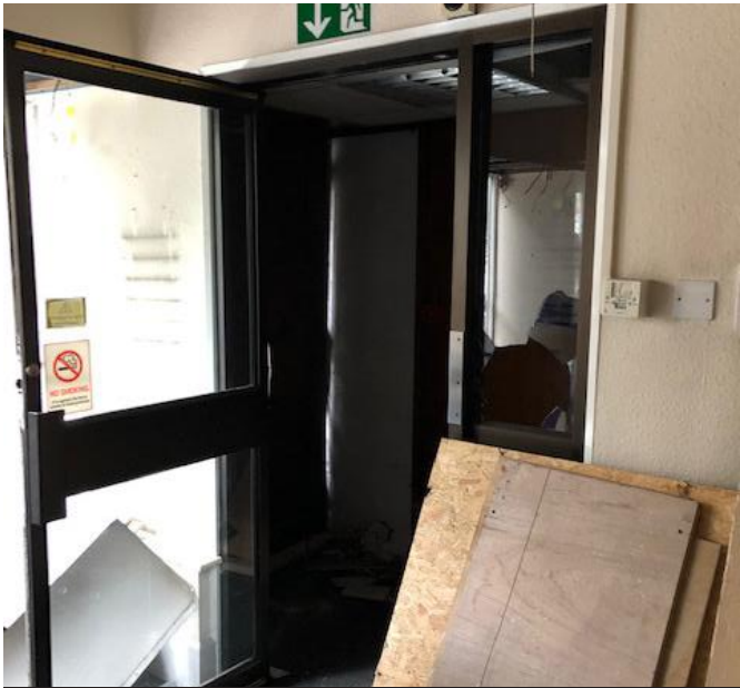
1: Facade and entrance doors not original
