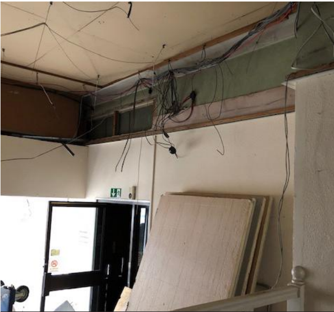
3: False ceiling with non-original coving above
