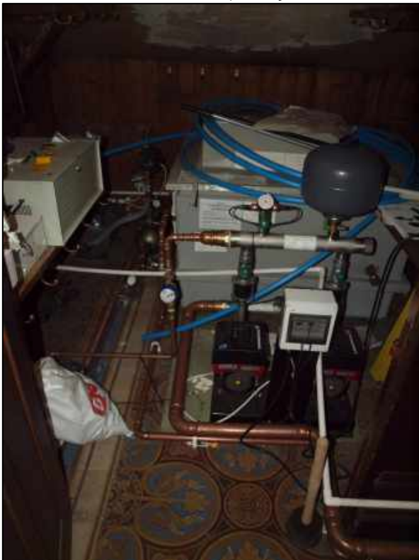
Plate 14: Detail of pipework in below stairs cupboard
