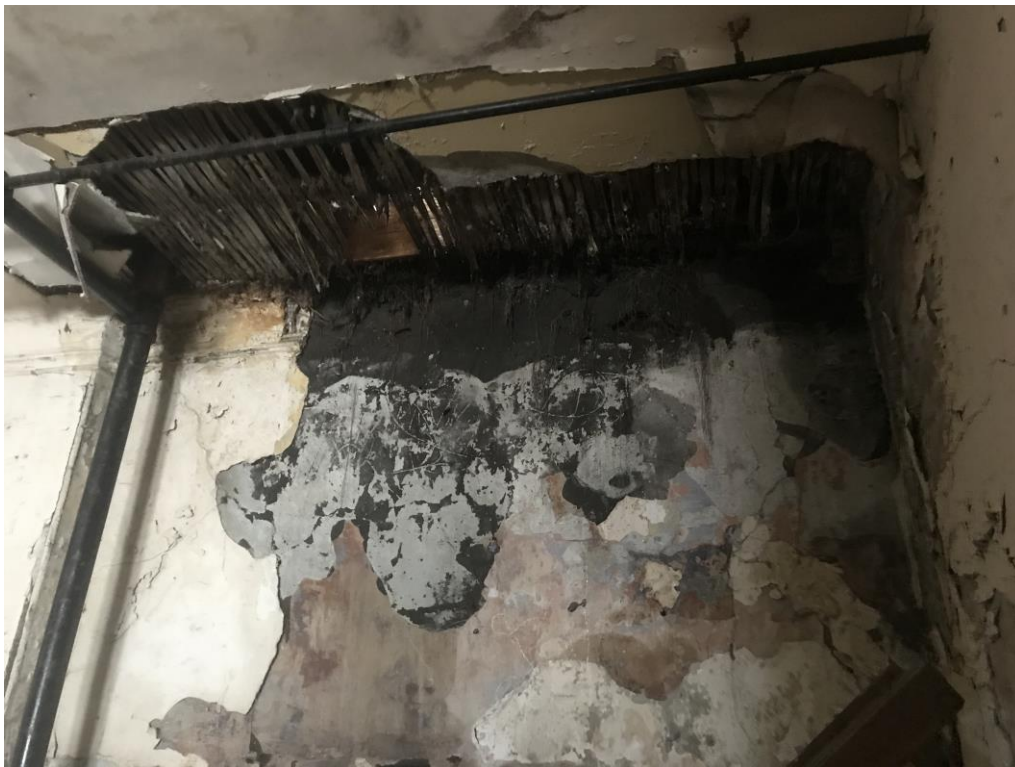
Photo 23 – Collapsed Ceiling Above First Floor to Mezzanine
