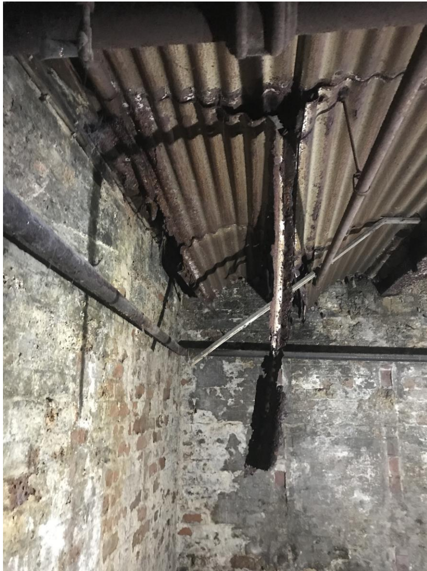
Photo 30 – Partial Collapse of Corrugated Sheet Metal in Basement
