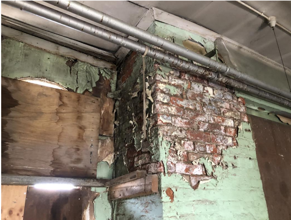
Photo 17 – Evidence of Water Ingress at Second Floor Level
