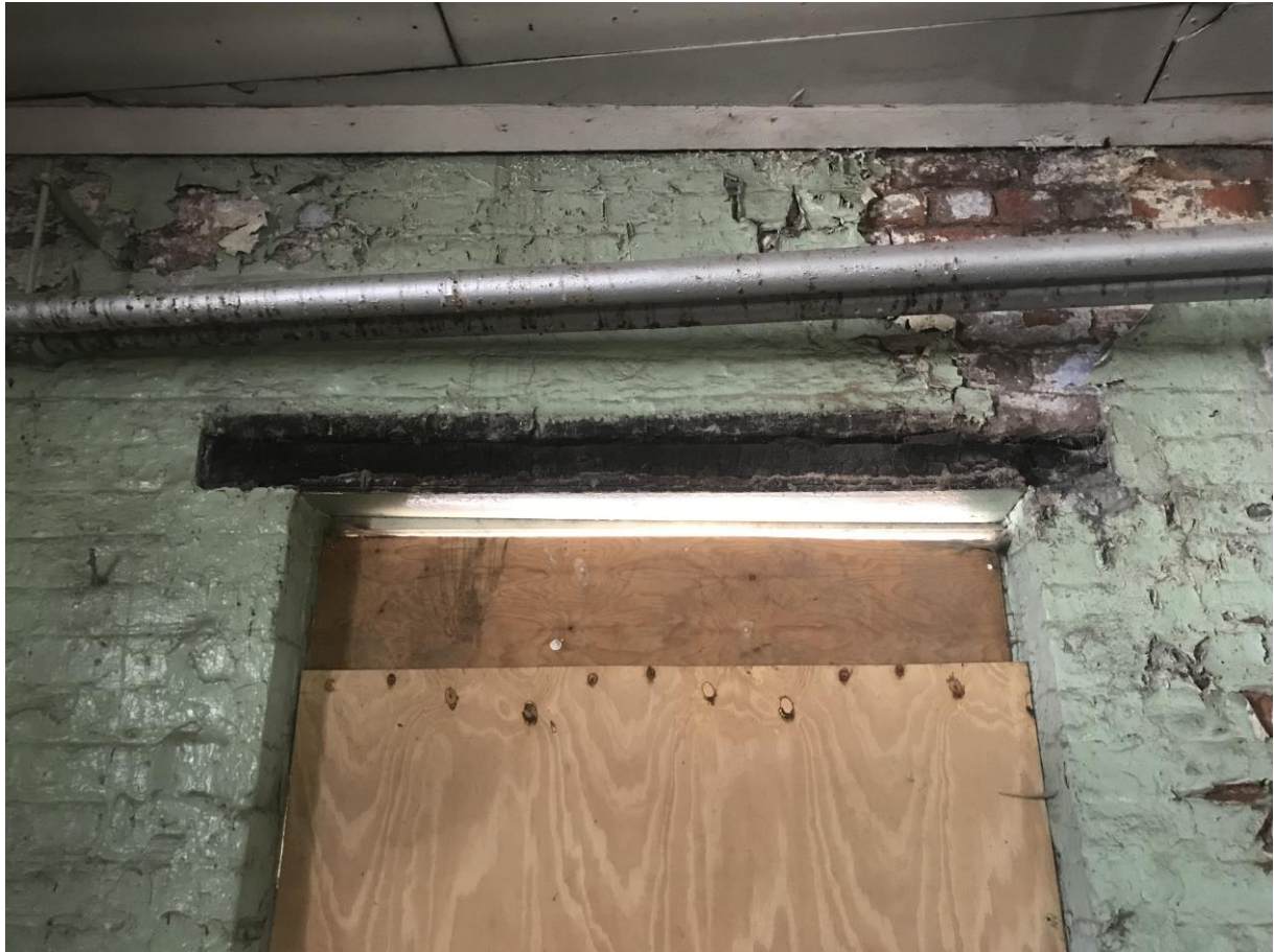
Photo 15 – Existing Fire-Damaged Timber Beam to Northeast Elevation
