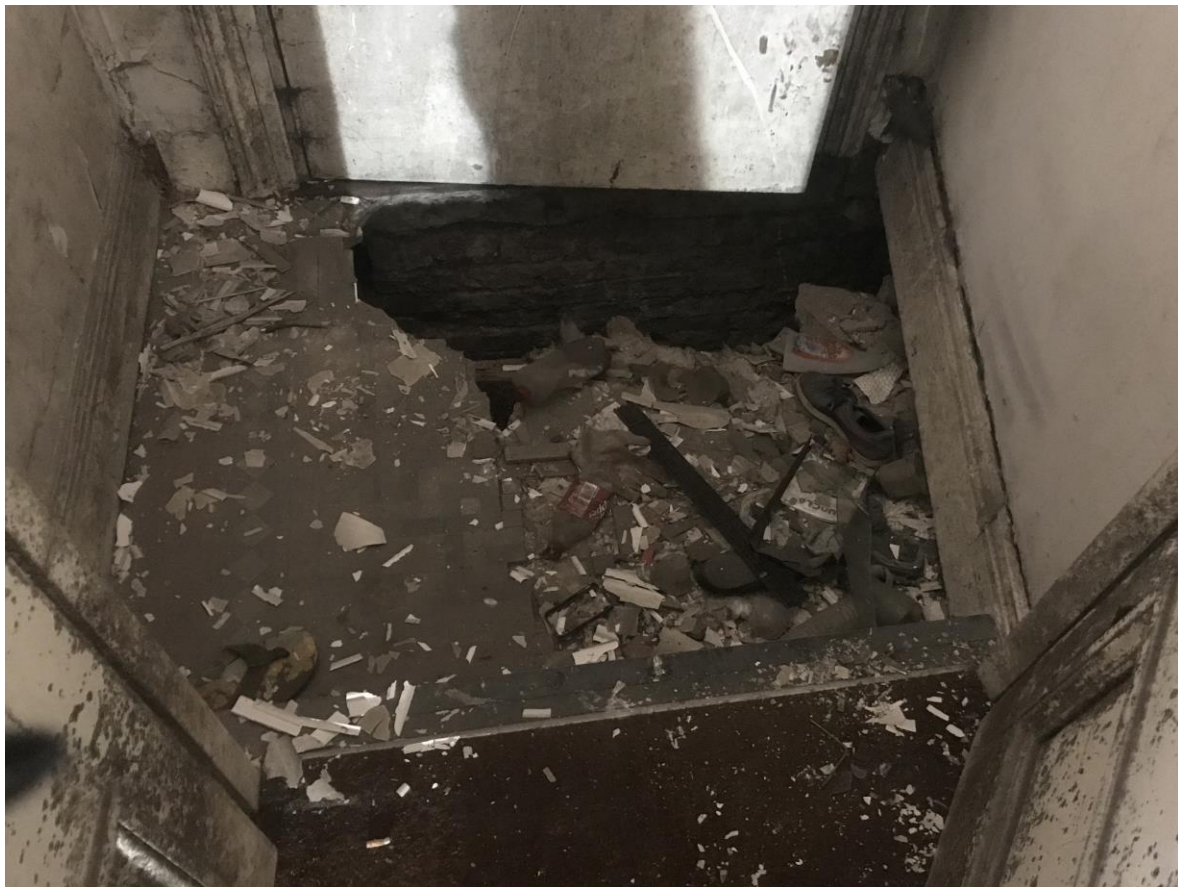
Photo 27 – Ground Floor Partial Collapse at Laystall Street Entrance Door
