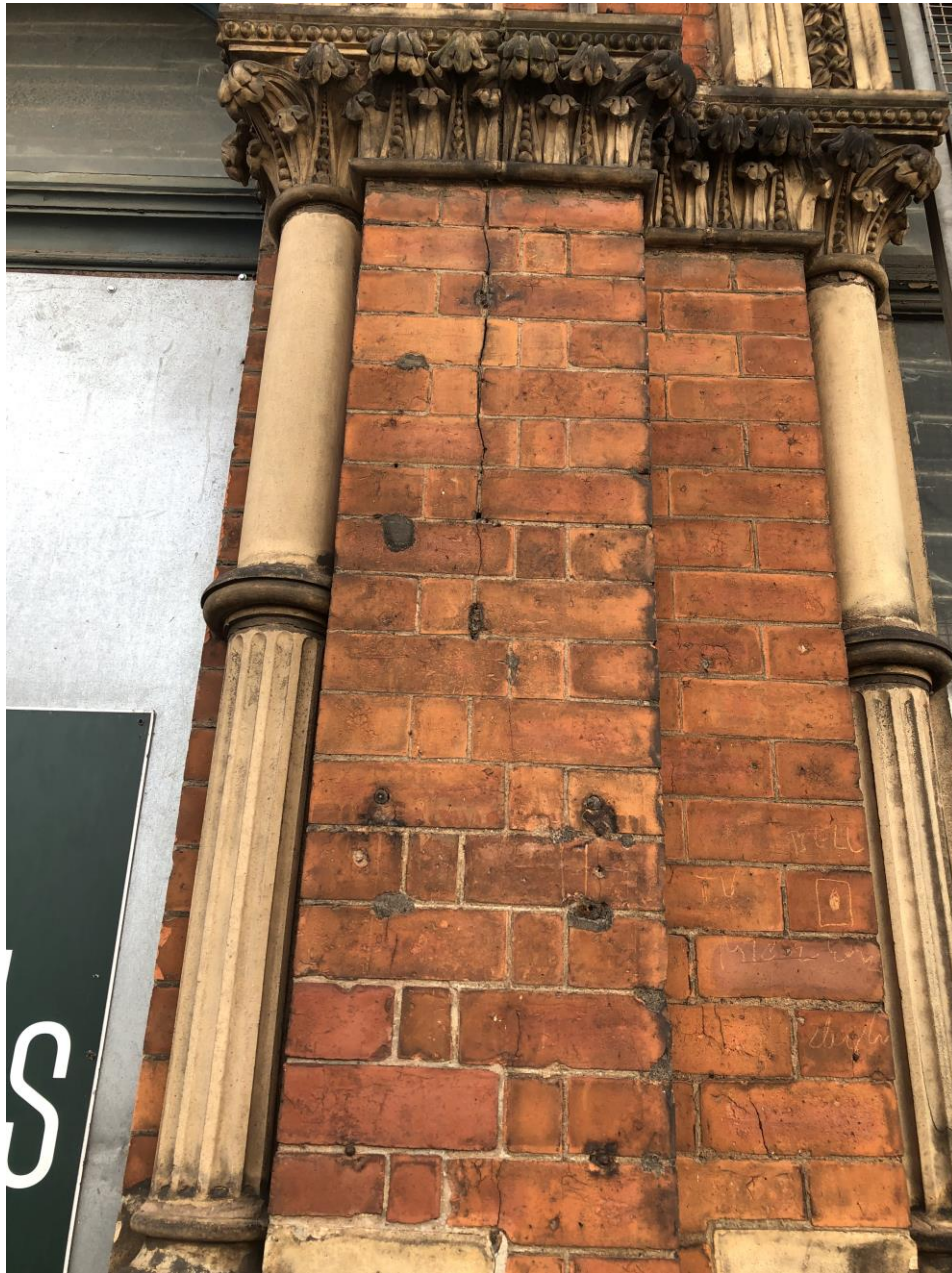
Photo 8 – Vertical Masonry Cracking Due to Corrosion of Ferrous Fixing
