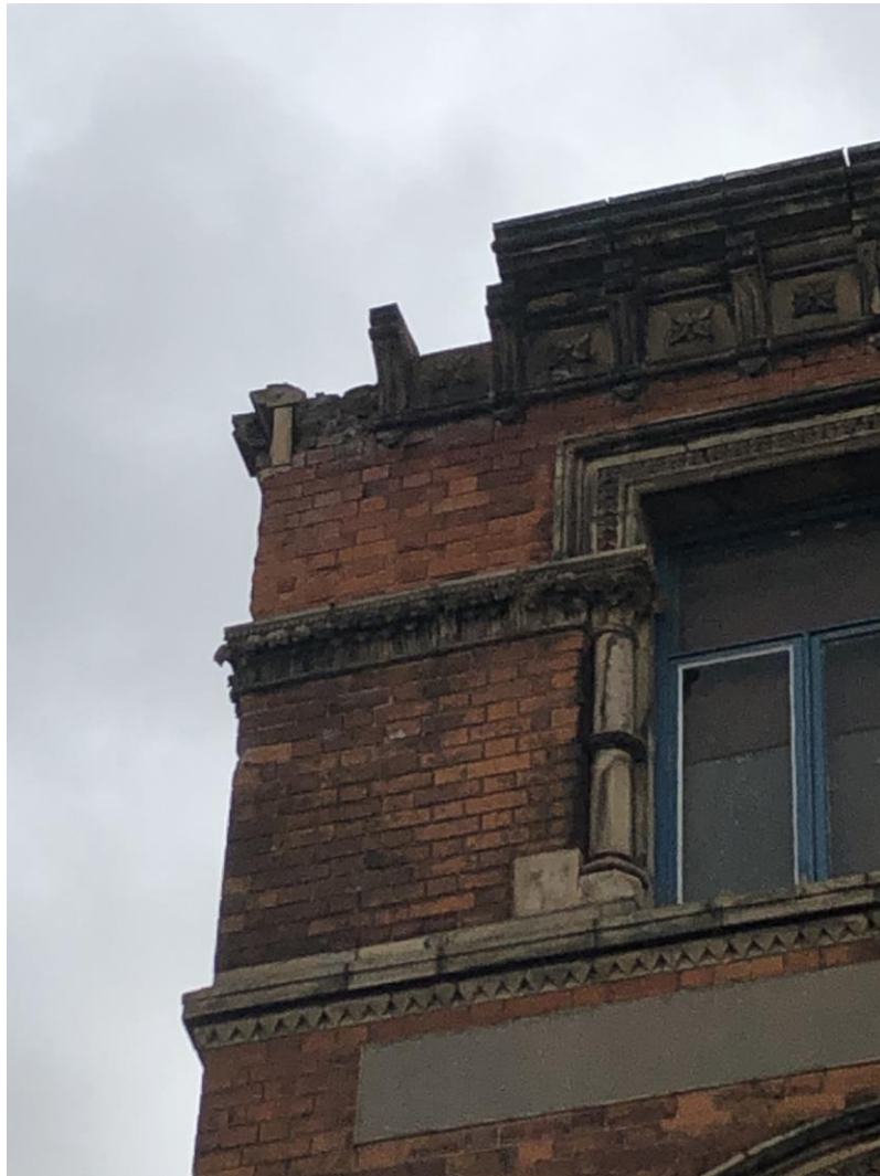
Photo 3 – Missing Terracotta Parapet Moulding
