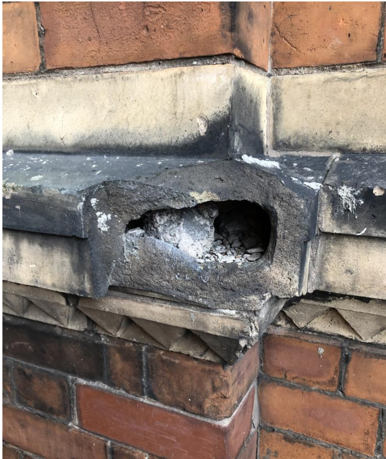
Photo 11 – Vehicle Strike Damage to Terracotta on Northeast Elevation
