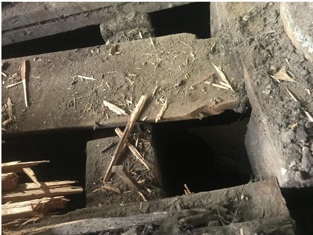
Photo 1 – Possible Brittle Fracture to Top Flange of Second Floor Beam
