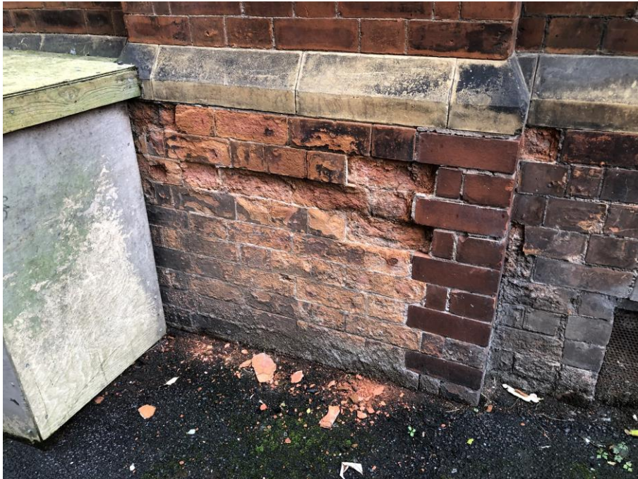
Photo 9 – Lower Level Freeze / Thaw Spawling of Brickwork
