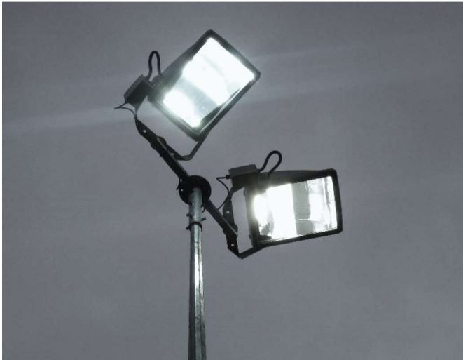
Artificial (Flood) Light Mast c/w Two Luminaries
