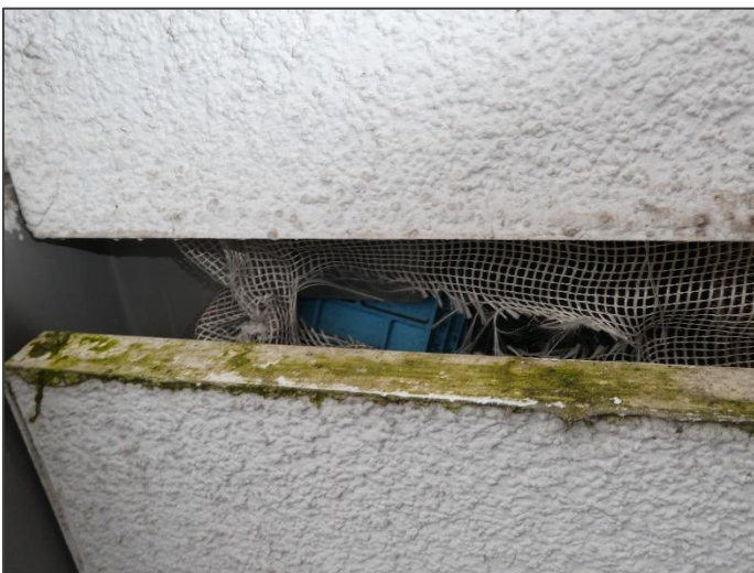
Photograph No. 3: Render system – Stains at open joint edges
