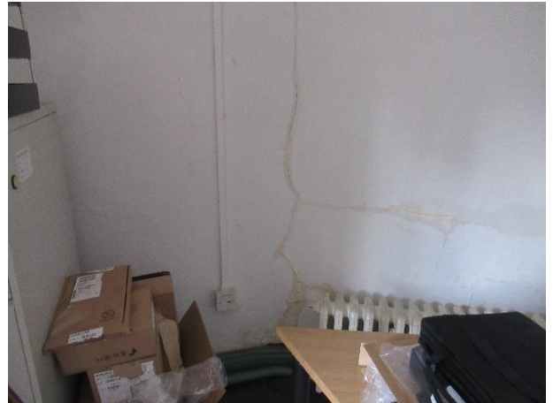
Water ingress at first floor of the Station Masters House
