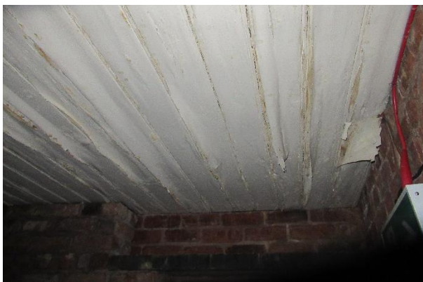
Loose paintwork to the ceiling in the basement
