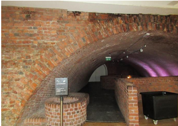
Water staining to masonry over viaduct arch
