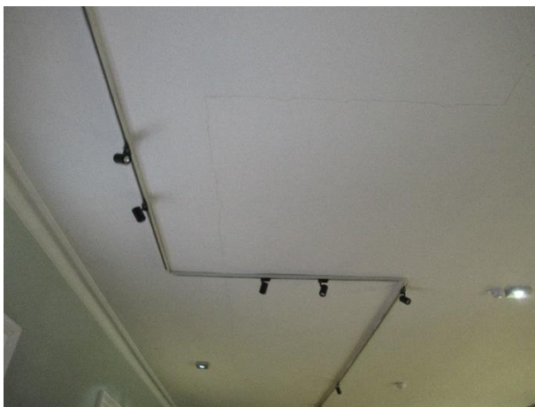
Cracking to the ceilings over the western Waiting Room
