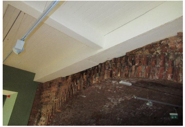
Water staining to masonry over viaduct arch
