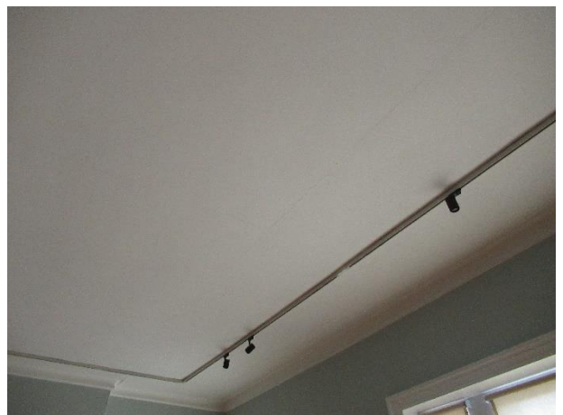
Cracking in the eastern Waiting Room
