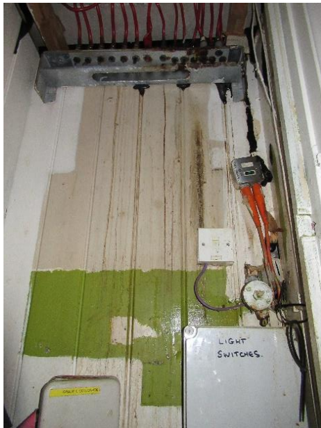
Electrical cupboard to south east corner
