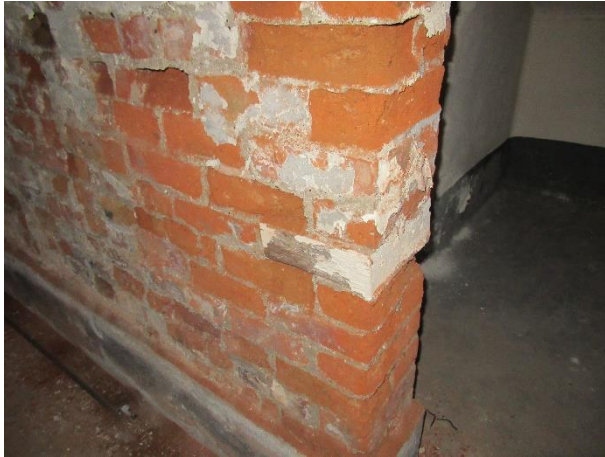
Erosion of masonry in the basement
