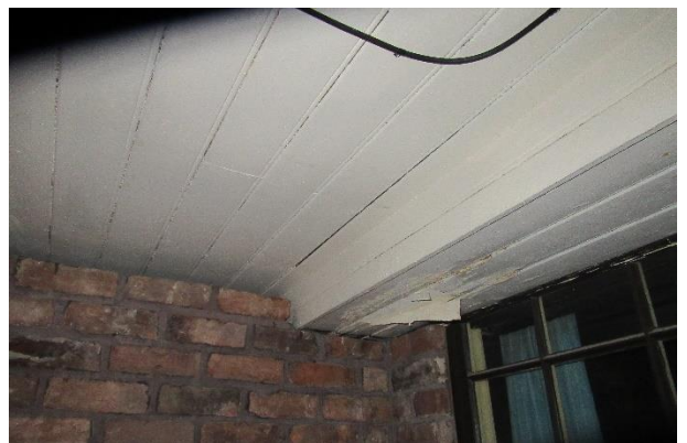
Loose paintwork to downstand beam
