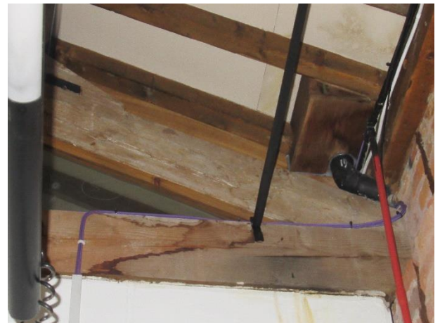
Timber hopper units to drainage outlets behind the parapet
