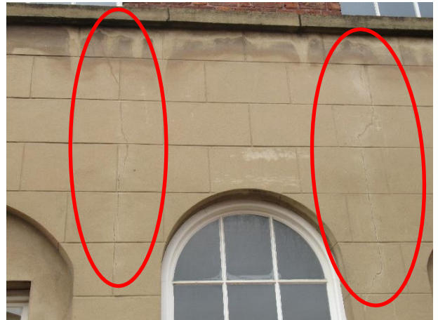
Cracking in render façade to south elevation
