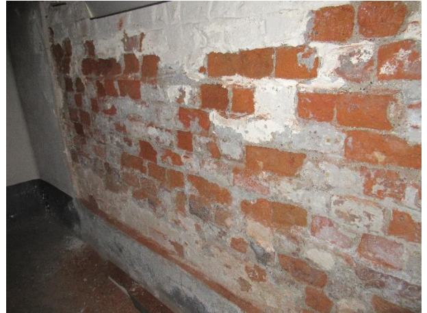
Erosion of masonry in the basement
