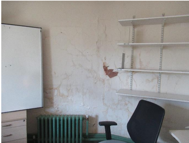
Water ingress at second floor of the Station Masters House
