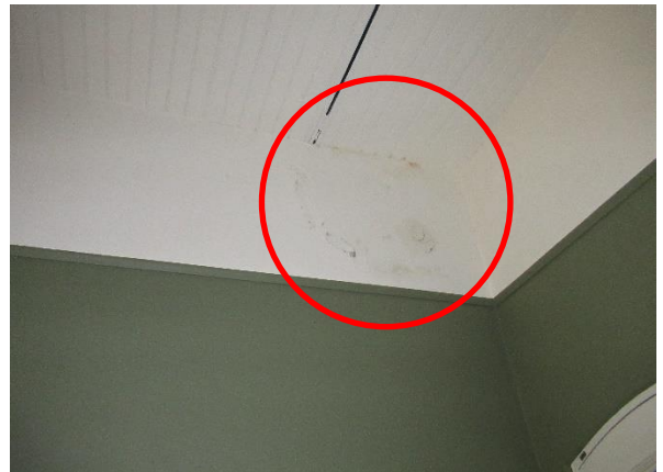
Water staining to wall finishes at ceiling level
