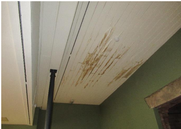
Water staining and loss of finishes to ceiling
