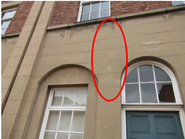
Cracking between window openings to south elevation
