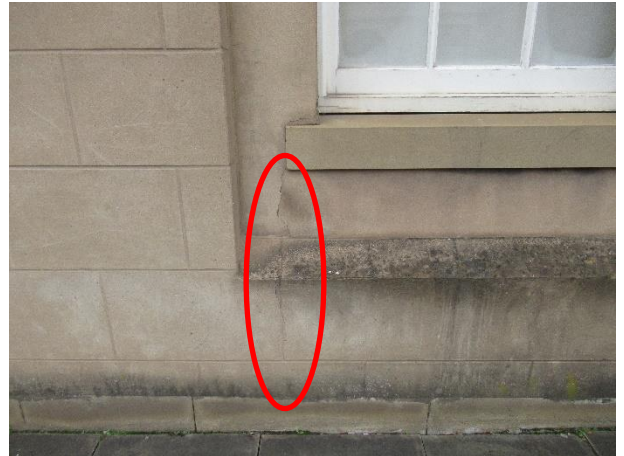
Cracking to window reveals at sill level.
