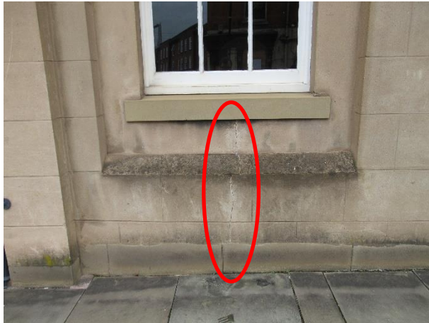
Cracking below ground floor windows
