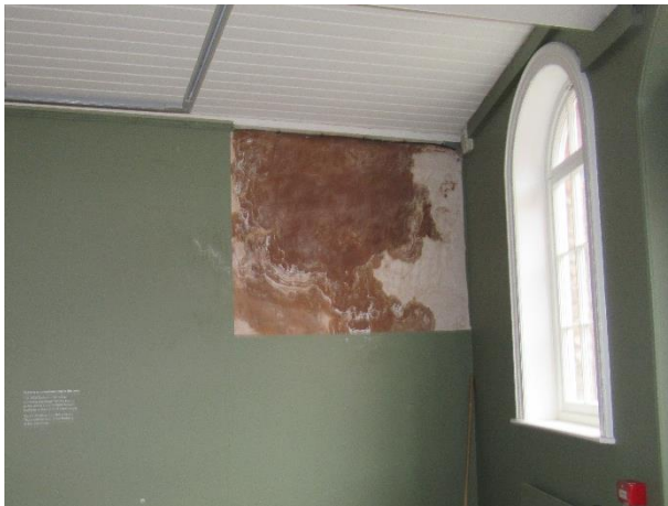
Water ingress into entrance hall
