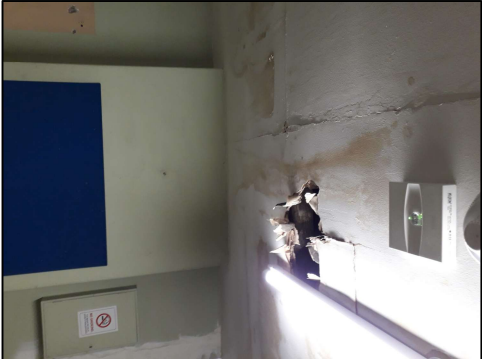
P20 - View of Break Out Area A1/18 hole in plasterboard ceiling to be made good.
