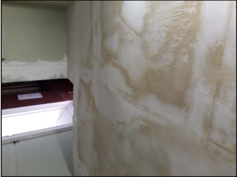
P21 - View of Break Out Area A1/18 water damaged plasterboard ceiling to be replaced.
