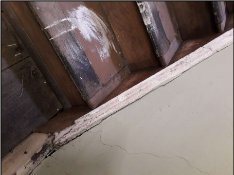
P24 - View of Break Out Area A1/18 To refix loose section of moulding above string to steps.
