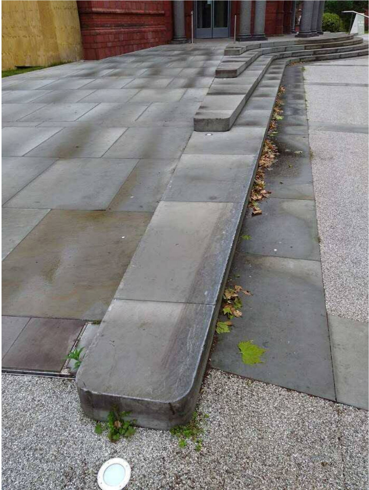
Photo 6. Close up damage to steps
