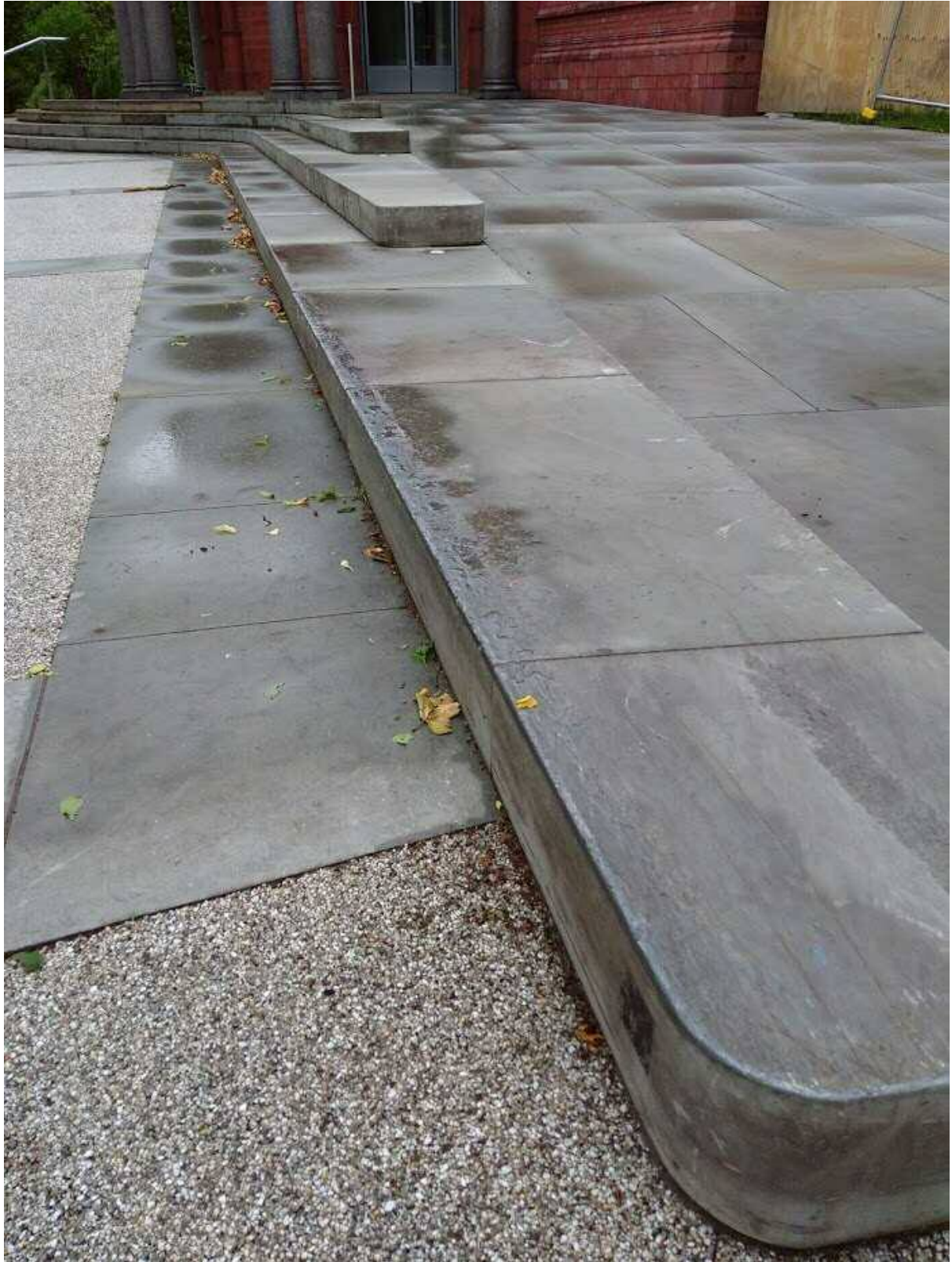
Photo 4. Close up damage to steps
