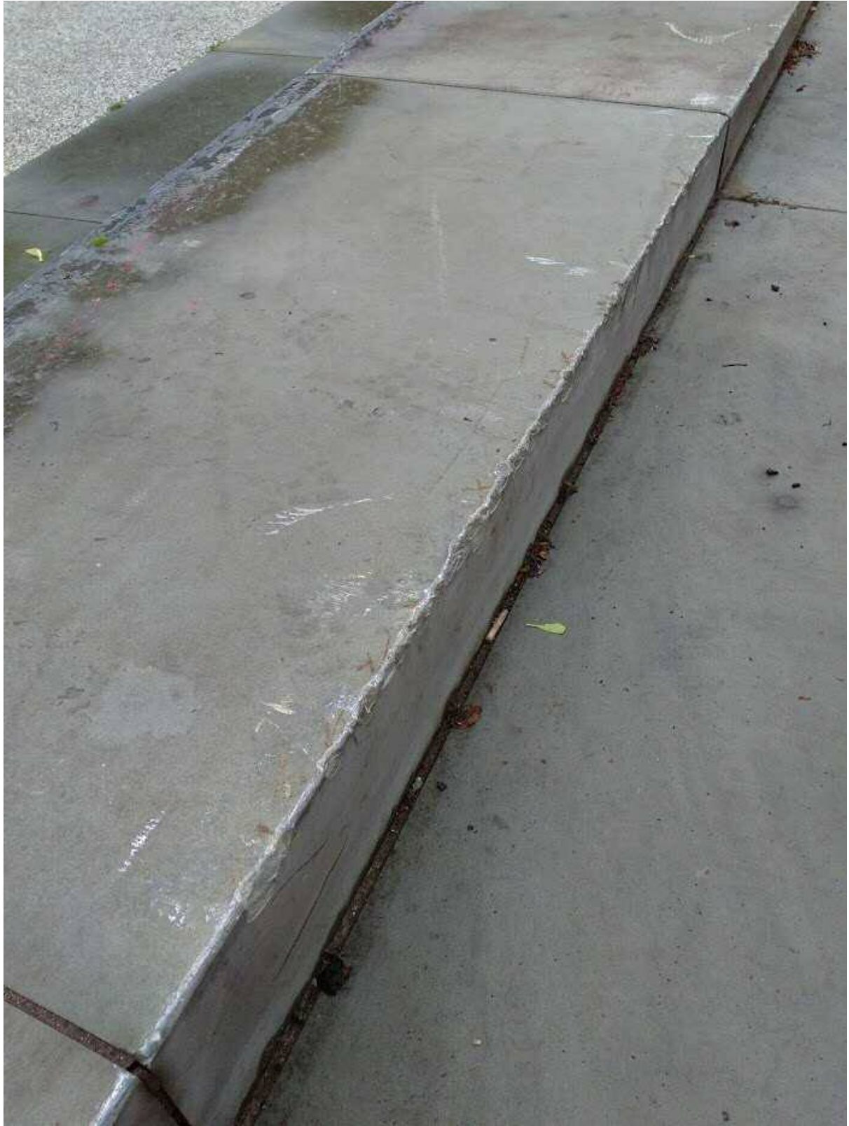
Photo 3. Close up damage to access ramp
