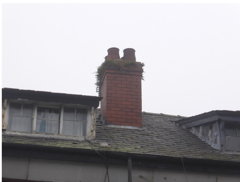
Photograph 2. Existing front dormer in very poor condition.
