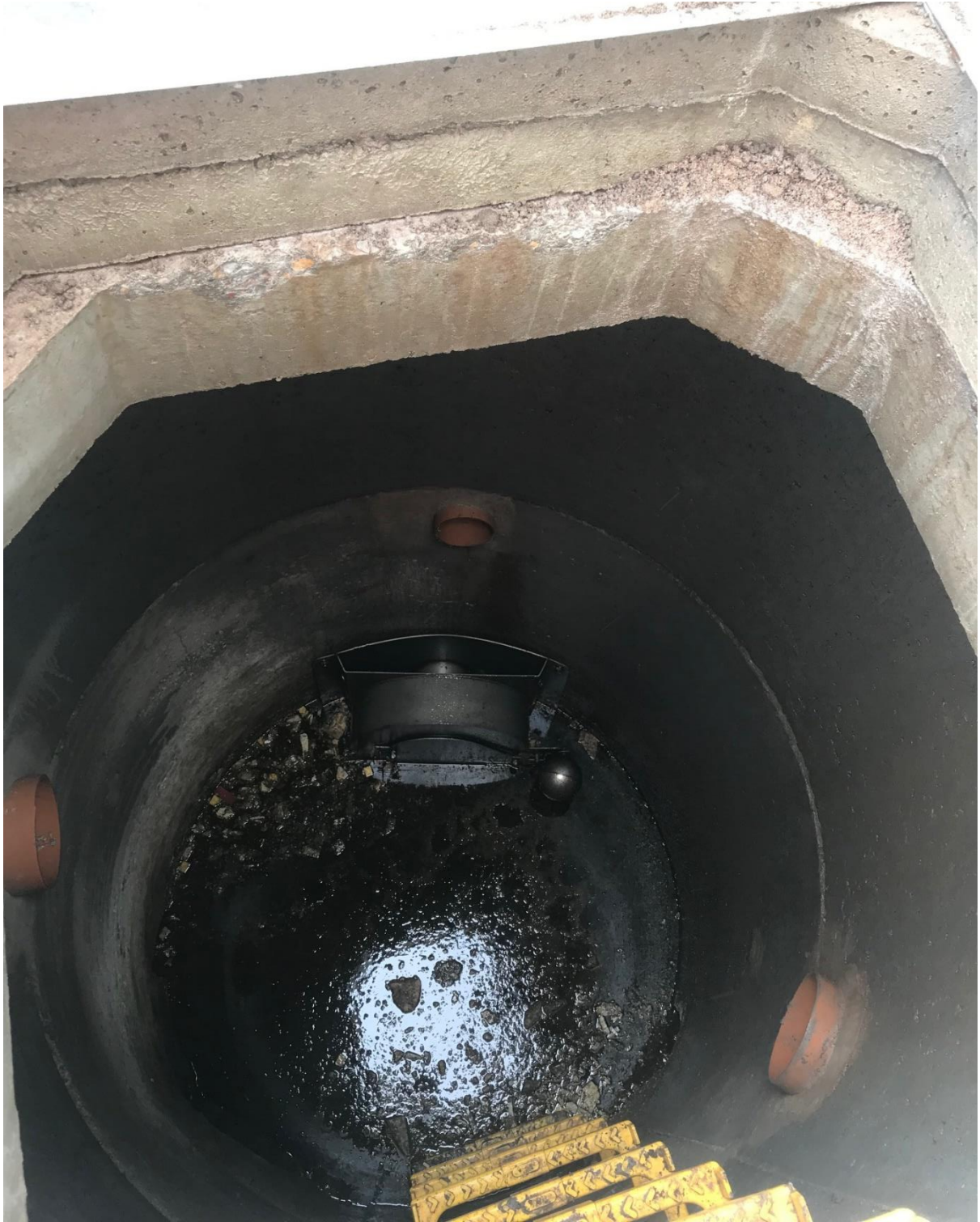
Figure 6 shows the hydrobrake flow controller fitted in the manhole
