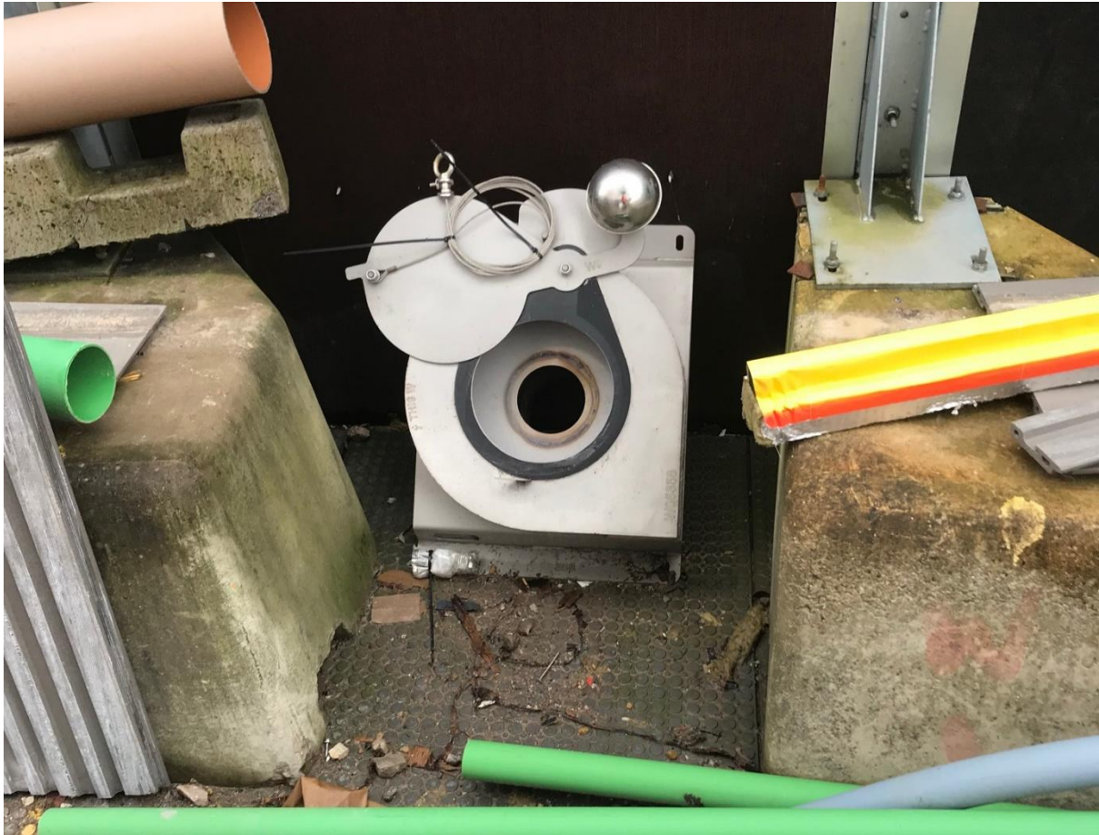
Figure 3 shows the Aco Q-Brake Vortex hydrobrake flow controller on site prior to fitting in SW MH S02.
