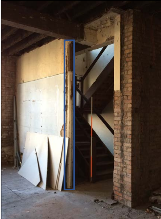
Detail 39: Fragmentary survival of part of timber doorcase to first floor level of staircase enclosure (outlined in blue). Fragment of “clay pot” construction in the wall adjacent to the doorcase suggests mid-20 th century reconstruction of the enclosure following bomb damage.
