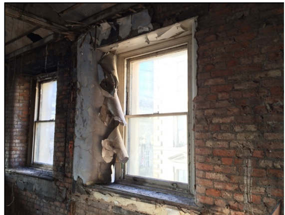
Detail 14: Fragmentary survival of internal lime plaster to bullnosed return to window reveal at third floor level.
