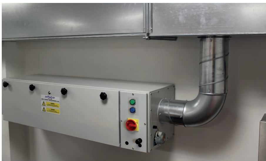
Figure 6 - UV-O 1000 Unit Installed
