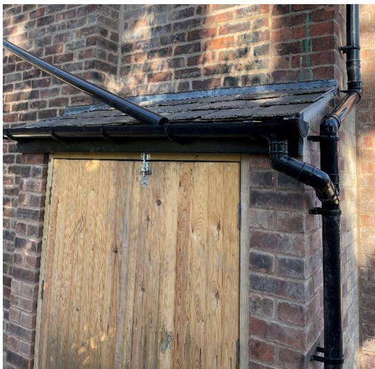
front of meter housing
