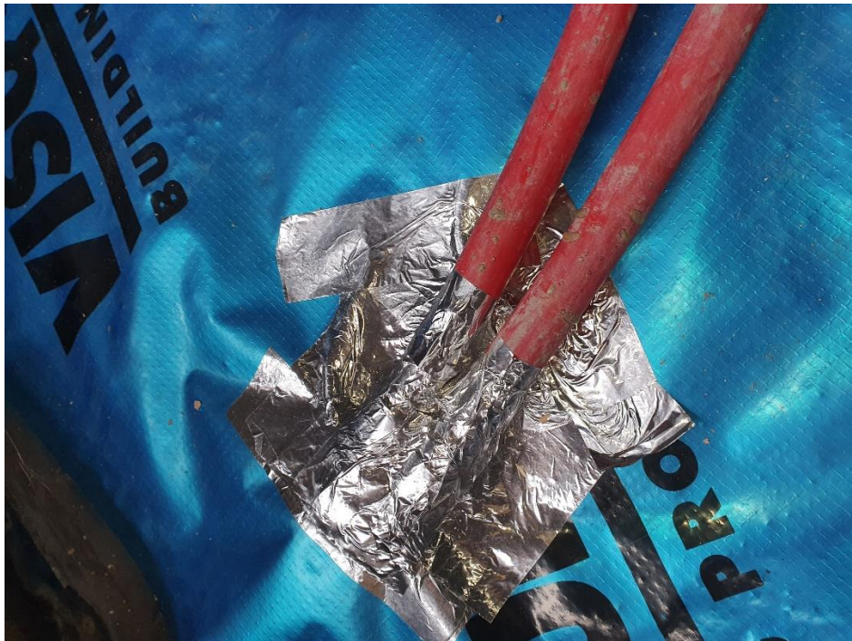
Photograph 8: Extra taping applied to Plot 2 car port cable. Untidy but seal formed (October 2020).
