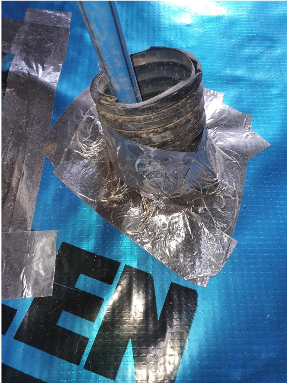
Photograph 5: Poor/untidy taping of service entry with gaps between plastic pipe and tape in Plot 3 (October 2020).
