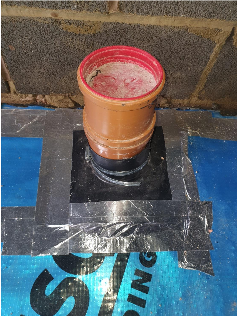
Photograph 4: Top hat and service entry in Plot 1 (Oct 2020).
