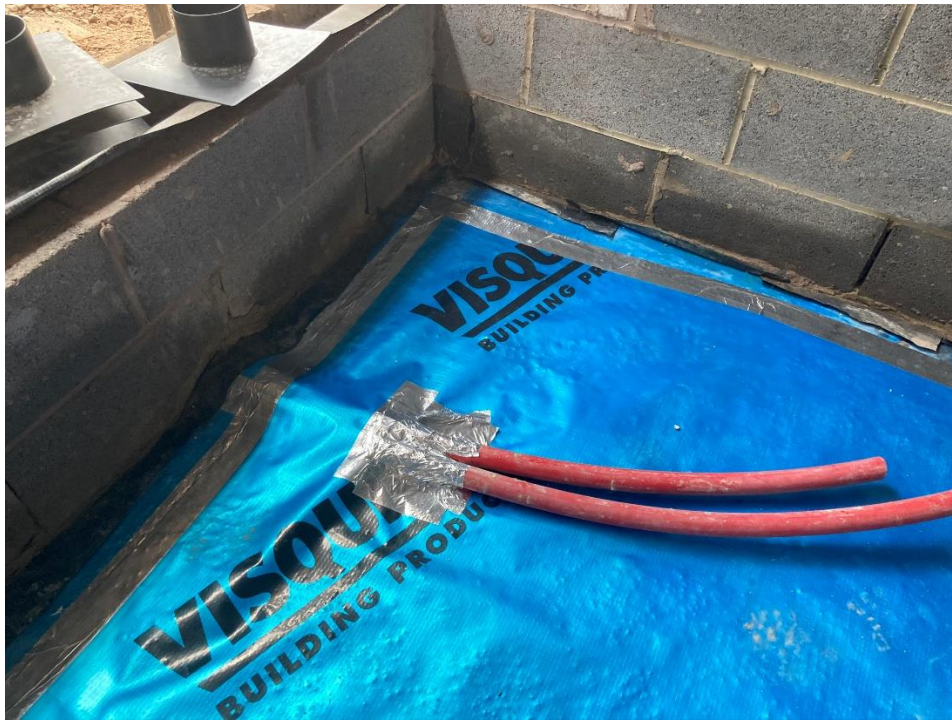
Photograph 7: Plot 2 car port cable with gap between and beneath 2 pipes (October 2020).
