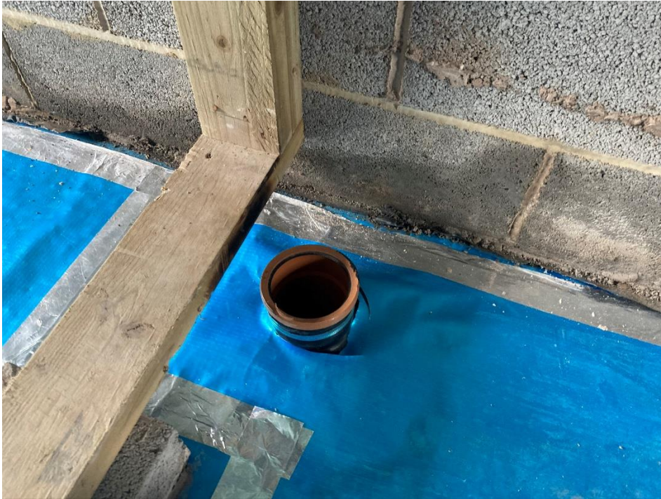
Photograph 9: Gap around service entry in Plot 2 with no tape at base (October 2020).
