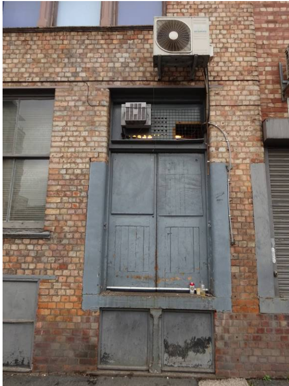
Figure 17: An example of a loading door.
