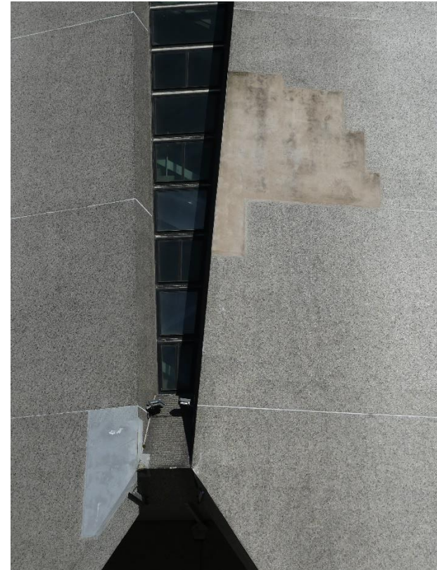
Figure 5.2: Current areas of missing tiles and remedial repairs to the southern elevation
