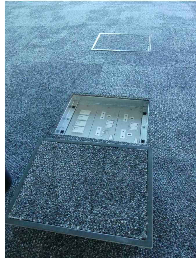
Figure 4.28: Modern services to Floor 4
