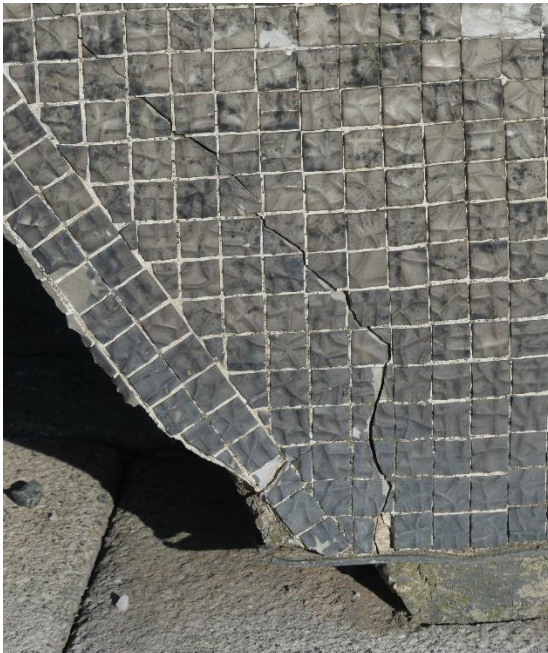
Figure 5.1: A current example of cracked mosaic adjoining the entrance to the southern elevation
