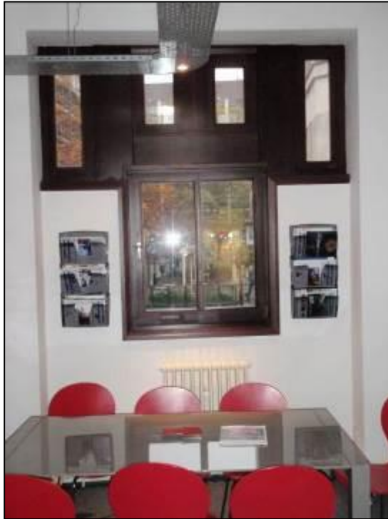
Altered window opening ground-floor - No significance
