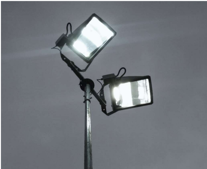
Artificial (Flood) Light Mast c/w Two Luminaries
