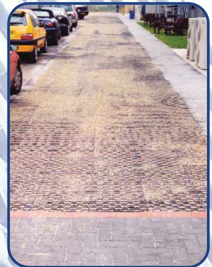
Car Park Infiltration Area.
