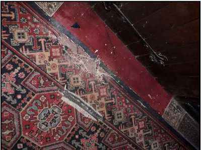
P51 - View of Tenant Hall / Suite A0/36. To carry out repairs to damaged section of carpet at threshold of doorway.
