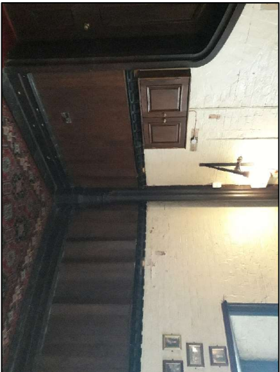
P54 - View of Tenant Hall / Suite A0/36. Timber T & G handling below dado rail has blown outwards due to damp penetration from historic defective external downspout. To refix 16No. loose vertical boards.
