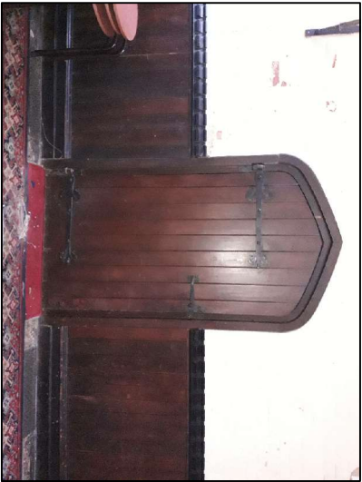
P50 - View of Tenant Hall / Suite A0/36. To plane the bottom of the door which is causing damage to the carpet area when opened and closed.
