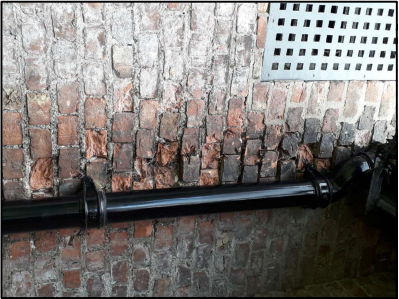
P54b - Rear Elevation gable end wall, defective brickwork joints to be repointed in a lime mortar.
