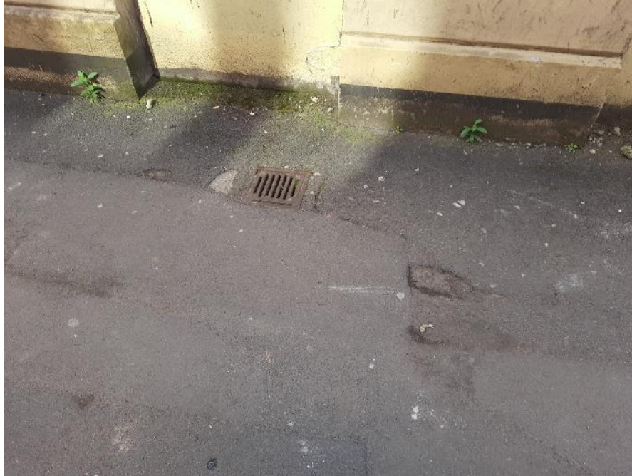
Figure 3.3 – Localised pitting in footway surface
