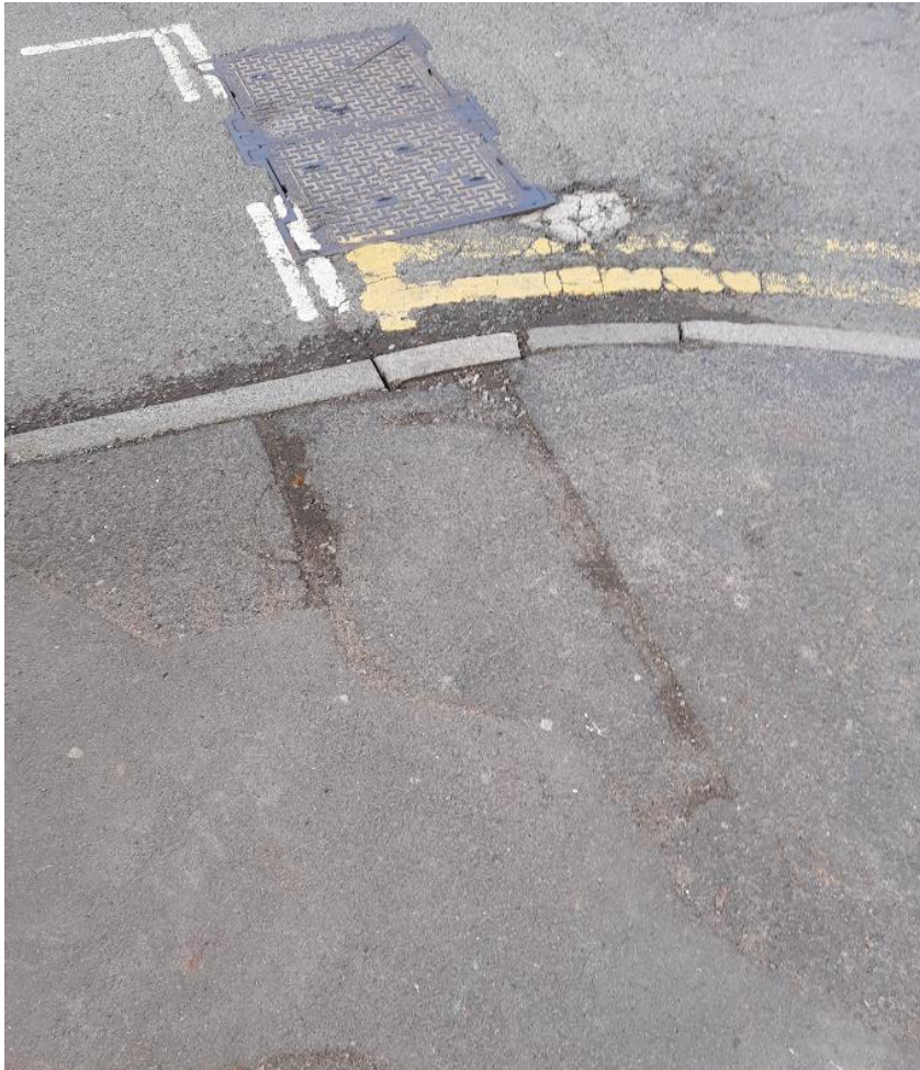
Figure 3.5 – Area of cracked asphalt adjacent to service chamber and loose kerbstones (Bloom St / Minshull St junction)
