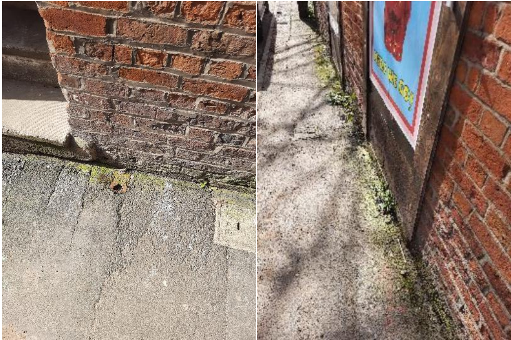
Figures 3.12 and 3.13 – Damaged cable outlet (left) and gas manhole cover (right)
