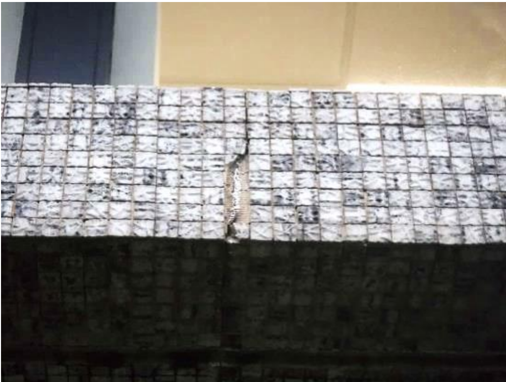
Photo B.58: A view showing a crack in the lower cantilever elevation (West machine hall south elevation)
