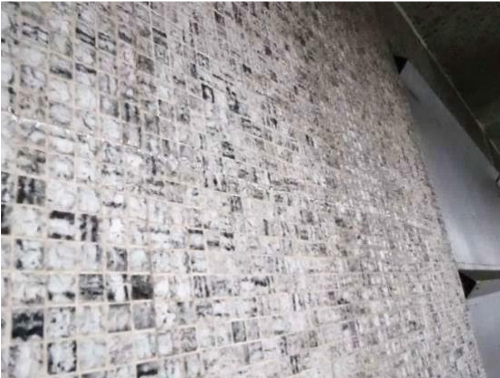
Photo B.45: A view showing a horizontal crack in the elevation (West machine hall north elevation)
