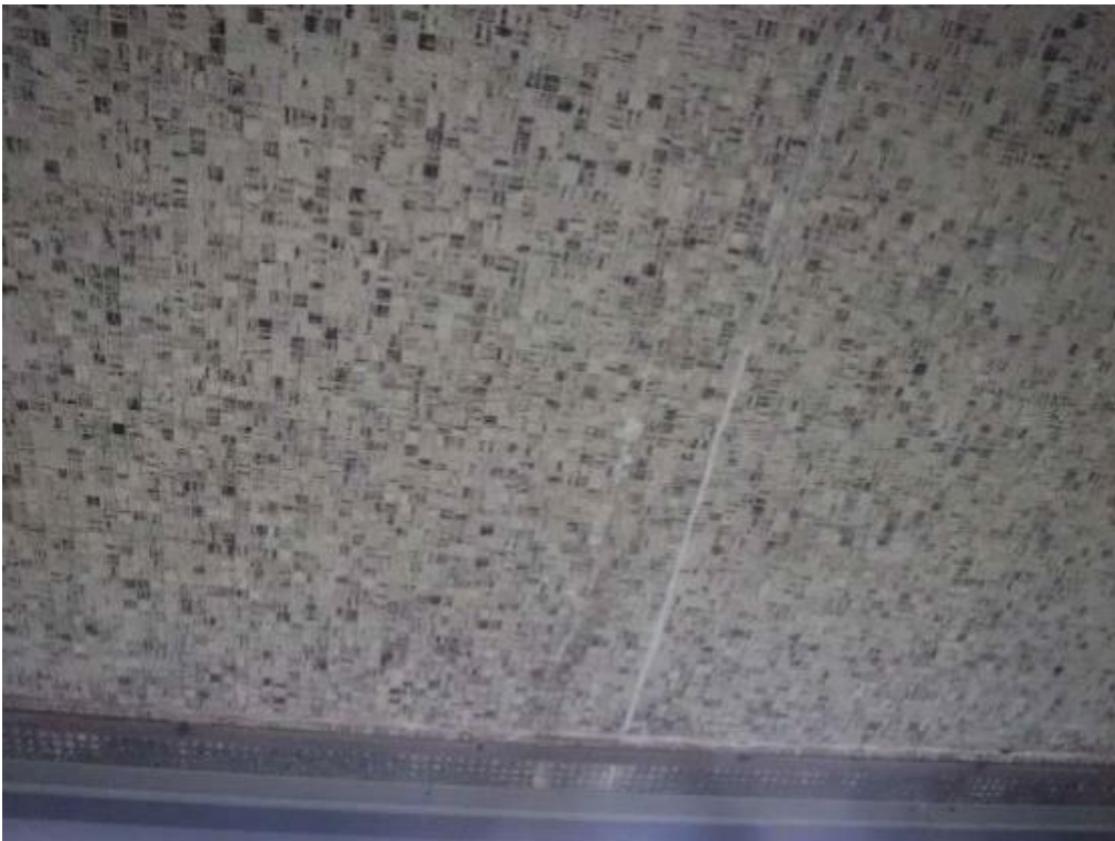
Photo B.60: A view showing a crack in the soffit of the upper cantilever (West machine hall, south elevation)
