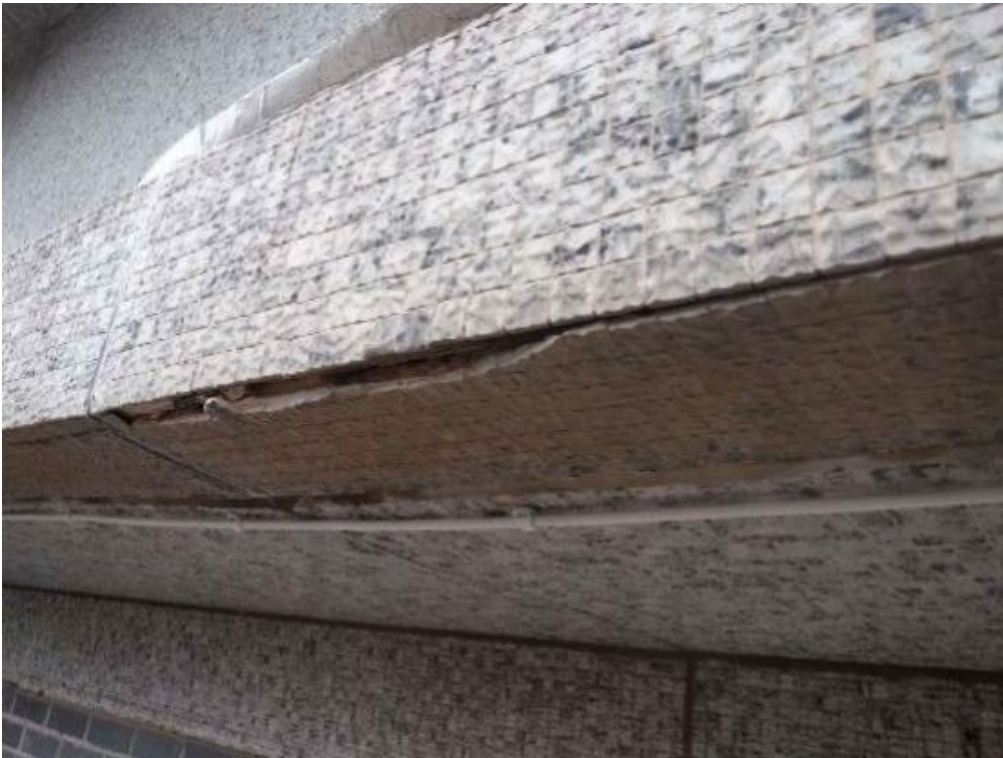
Photo B.91: A view showing spalling to the soffit of the lower cantilever (East Machine Hall)
