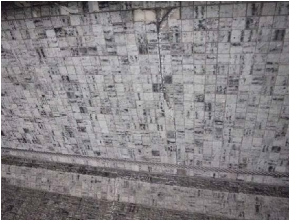
Photo B.63: A view showing a vertical crack in the south elevation of the West machine hall
