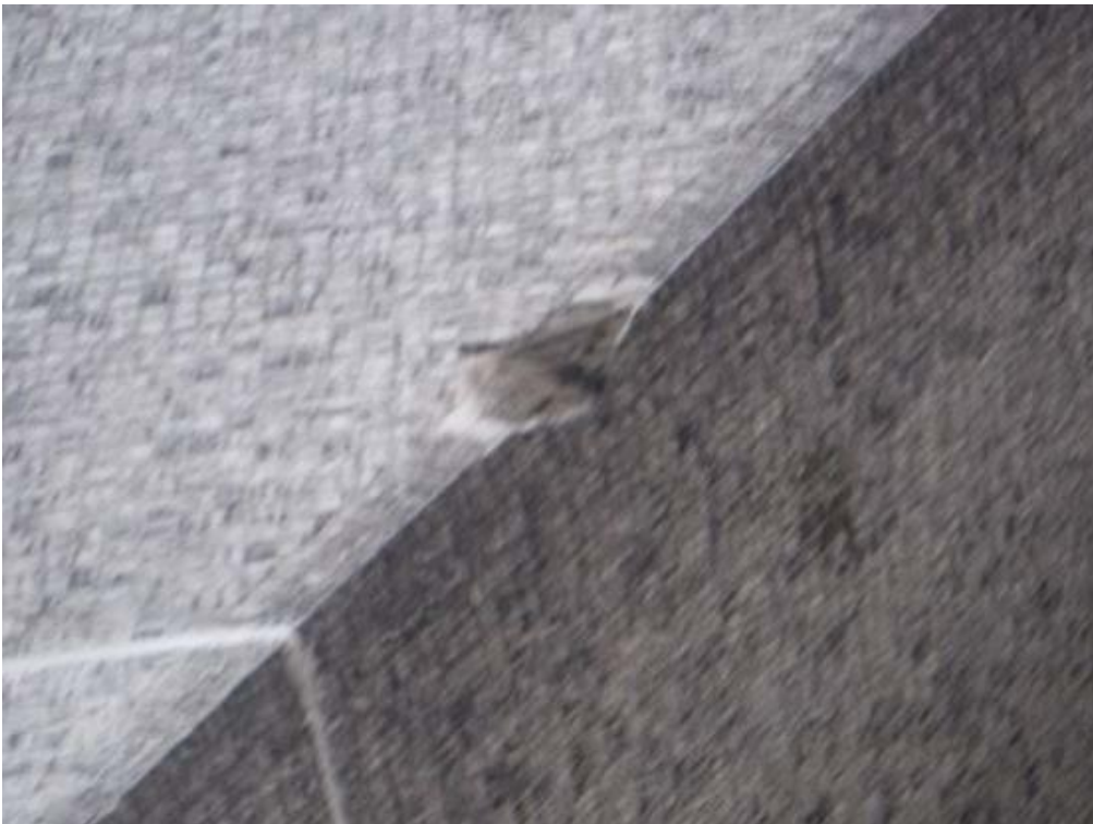
Photo B.8: A view showing a 'new' area of spalling to the 1st storey of the north elevation
