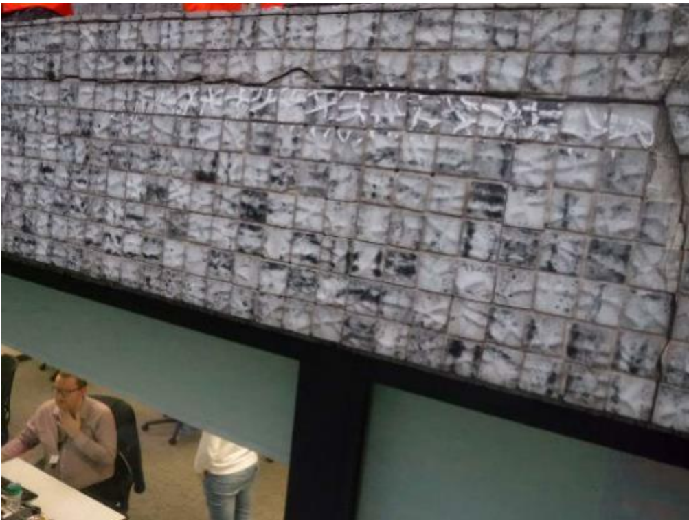
Photo B.62: A view showing a horizontal crack in the elevation of the lower cantilever (West machine hall, south elevation)
