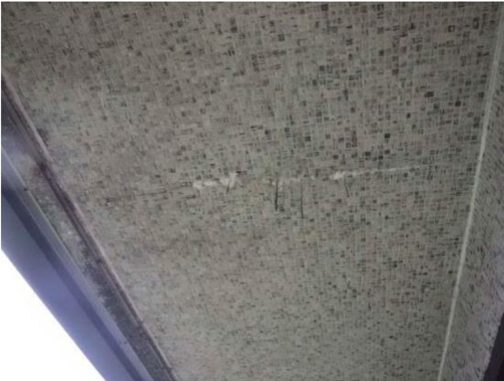
Photo B.67: A view showing a crack in the soffit of the upper cantilever (West Machine Hall, west elevation)
