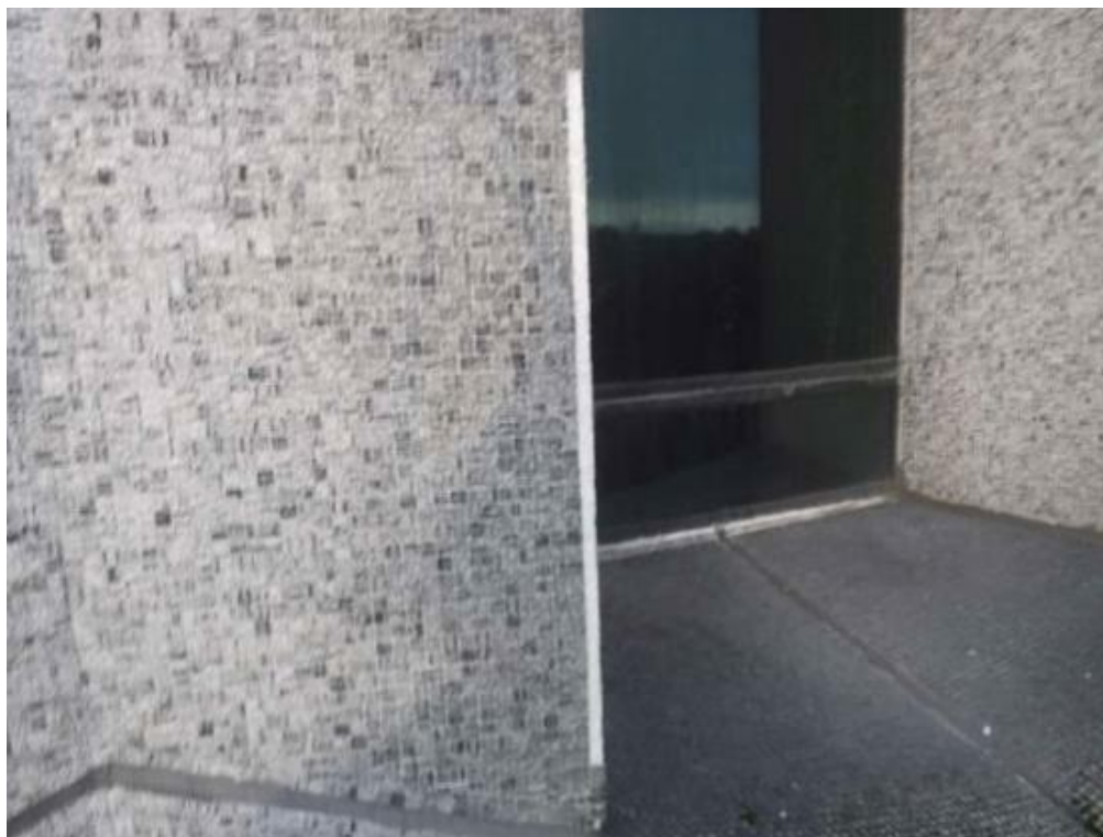
Photo B.29: A view showing missing tiles to the east elevation (row G storey 11)
