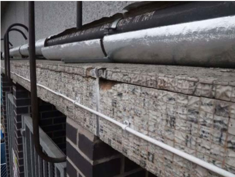
Photo B.90: A view showing an area of spalling and a horizontal crack in the east elevation of the lower cantilever (East Machine Hall)
