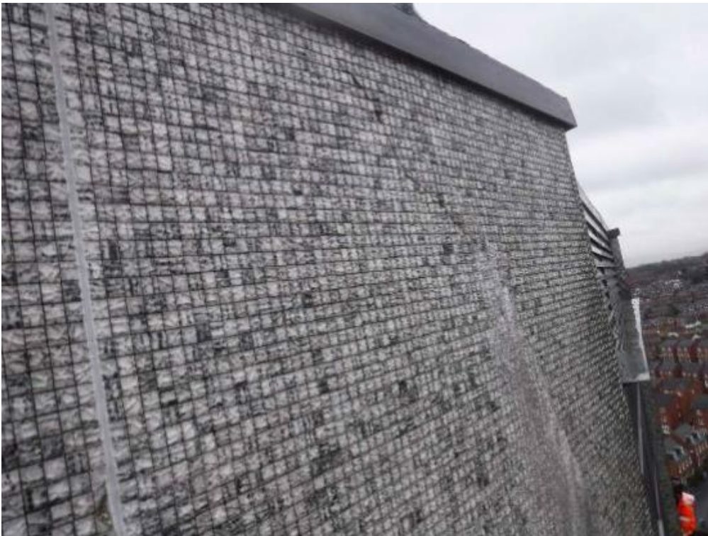
Photo B.12: A view showing a diagonal crack with leaching deposits to the 12th storey of the south elevation
