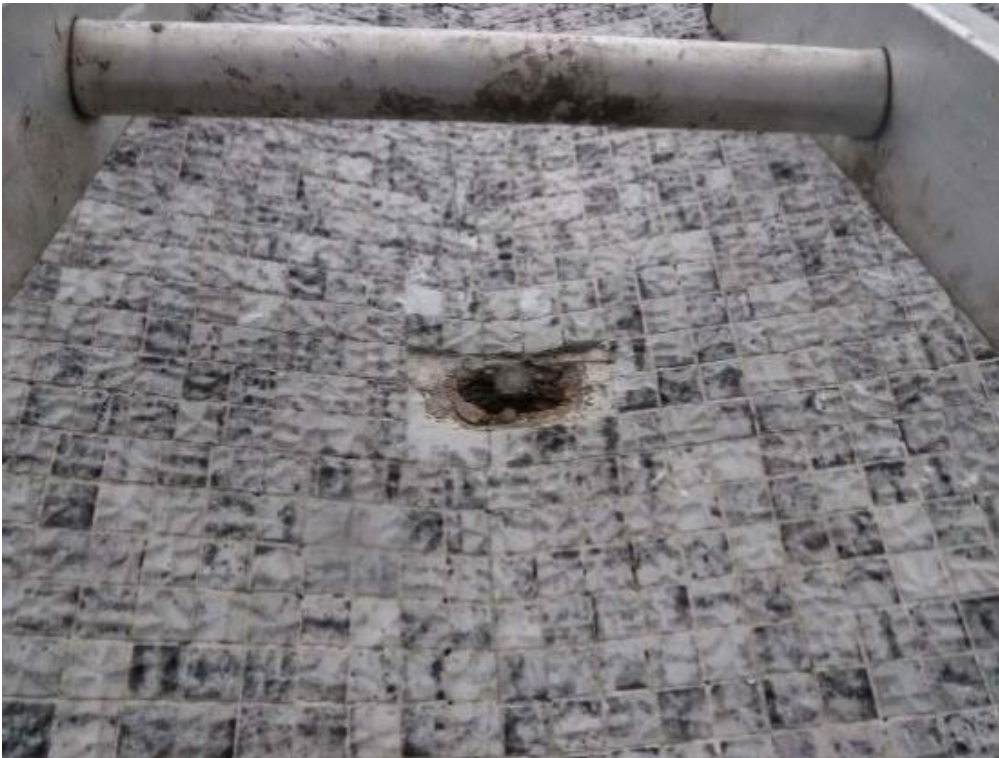
Photo B.27: A view showing spalling with exposed reinforcement to the east elevation (row R storey 2)
