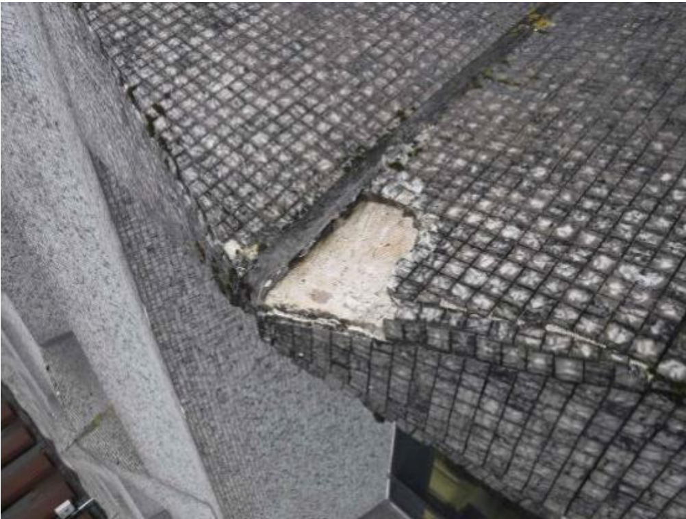
Photo B.38: A view showing missing tiles to the west elevation (row BD storey 11)
