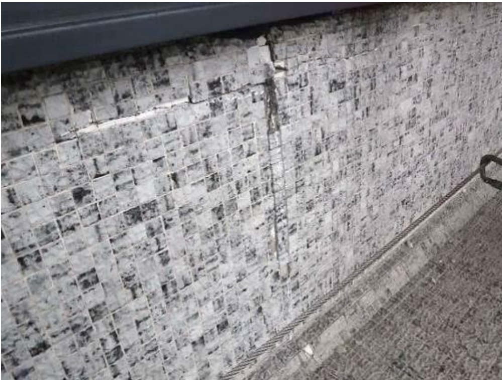
Photo B.80: A view showing vertical and horizontal cracks in the south elevation of the East Machine Hall
