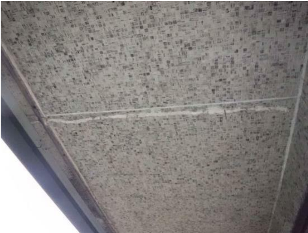
Photo B.54: A view showing a crack in soffit of the upper cantilever (West machine hall south elevation)
