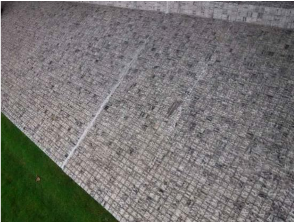
Photo B.57: A view showing a crack in the top face of the lower cantilever (West machine hall south elevation)
