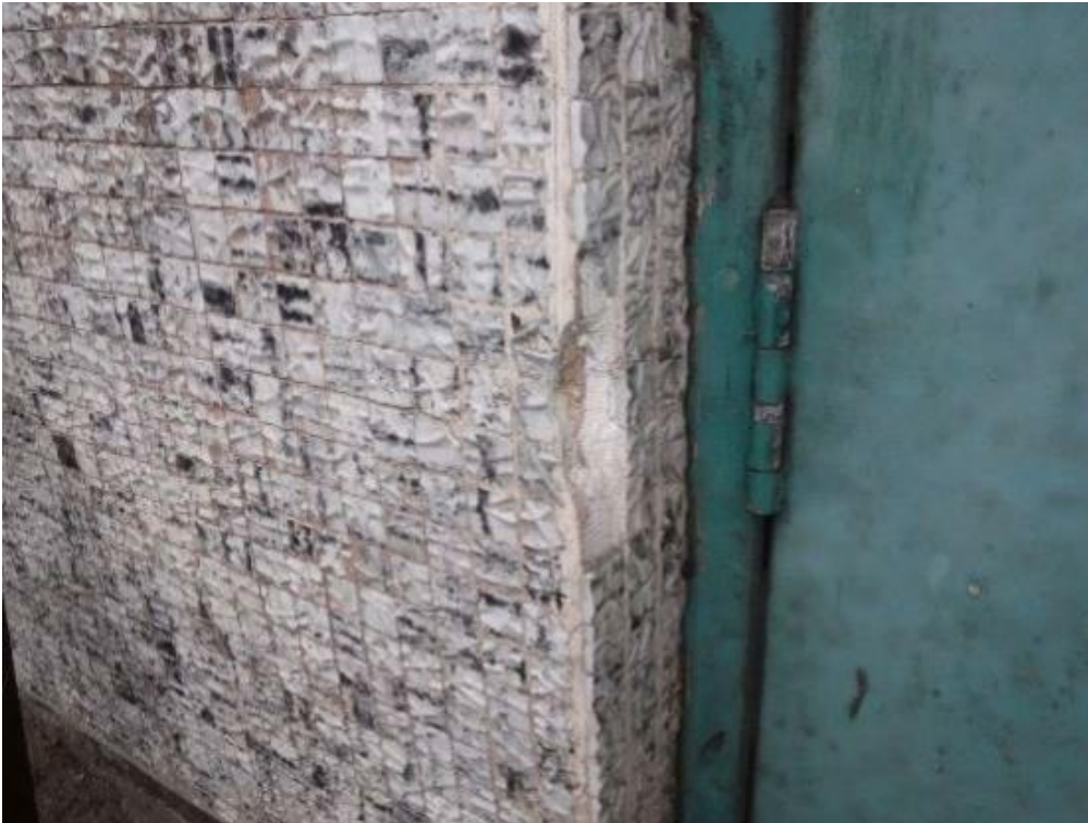
Photo B.49: A view showing spalling to the corner of the doorway (West machine hall north elevation)
