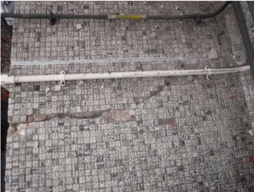
Photo B.51: A view showing a crack in the top face of the lower cantilever (West machine hall north elevation)
