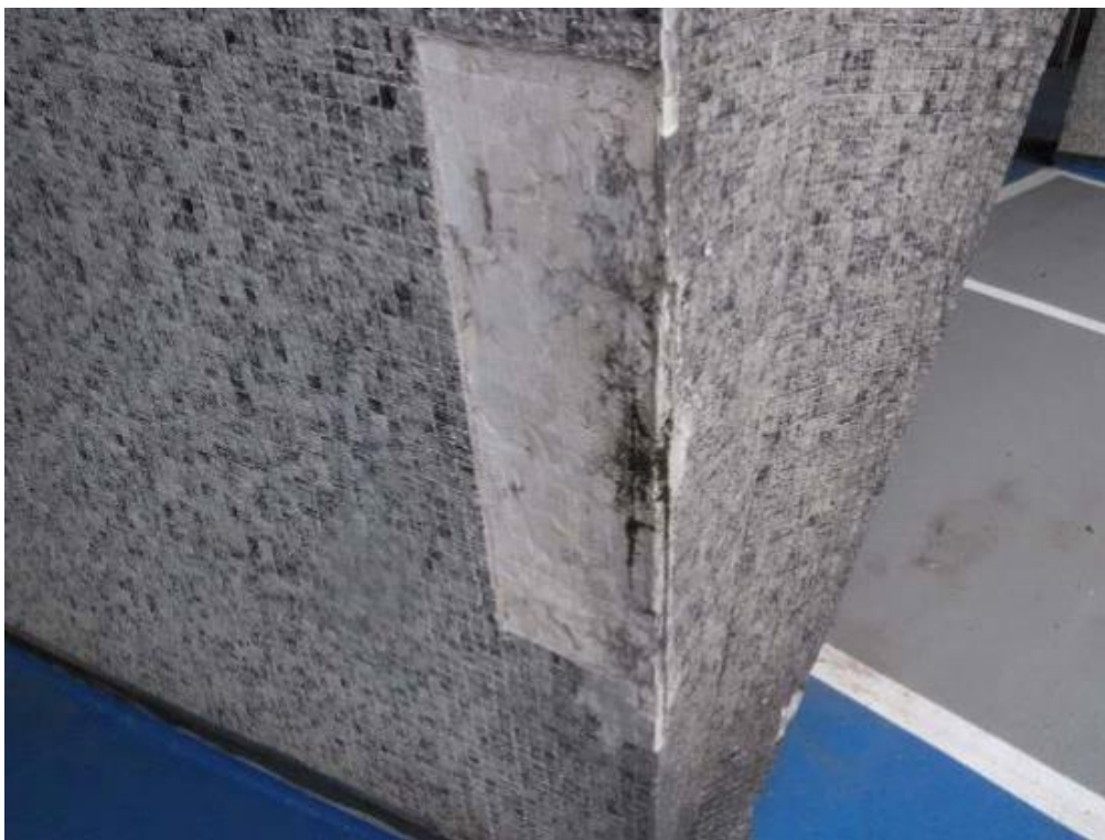
Photo B.33: A view showing missing tiles to the east elevation (row V storey 2)
