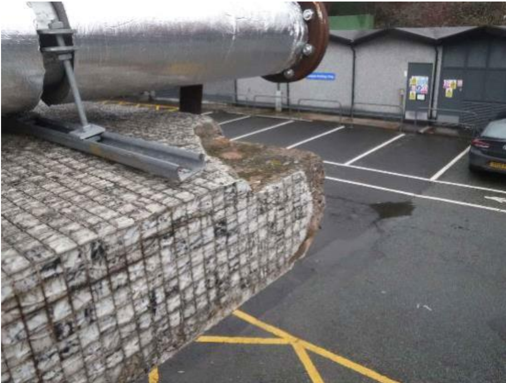
Photo B.73: A view showing spalling to the edge of the lower cantilever (East Machine Hall, north elevation)
