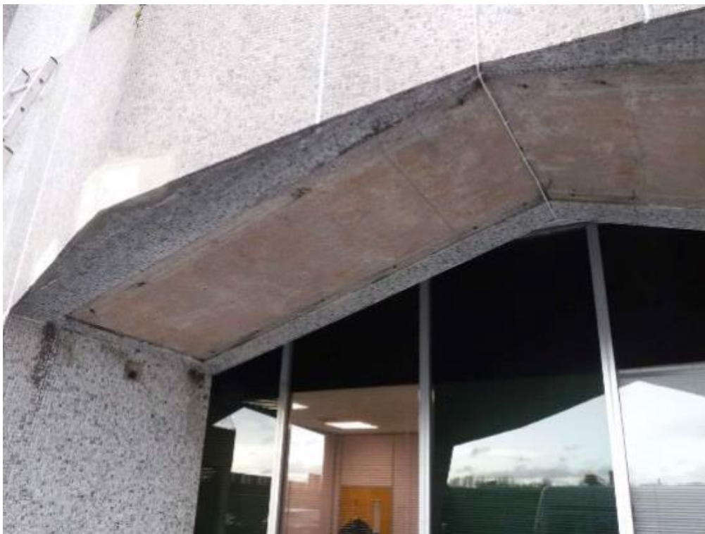
Photo B.26: A view showing missing cladding to the east elevation (row I storey 2)
