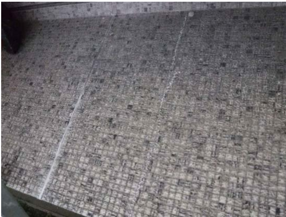
Photo B.56: A view showing a crack in the top face of the lower cantilever (West machine hall, south elevation)
