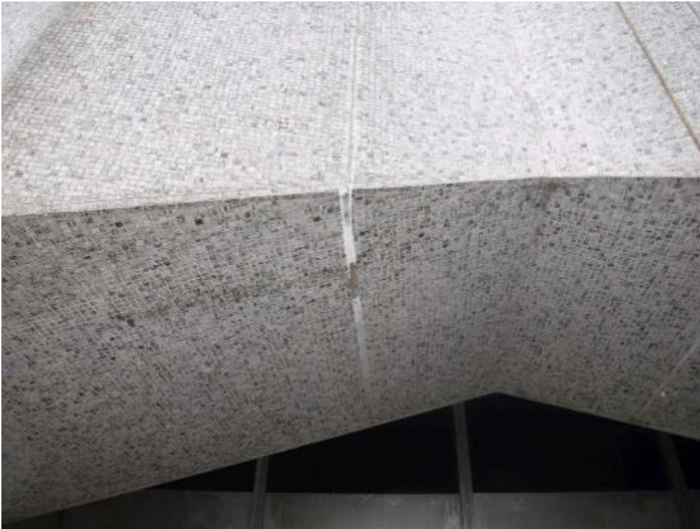
Photo B.35: A view showing de-bonded sealant (row BM storey 2)
