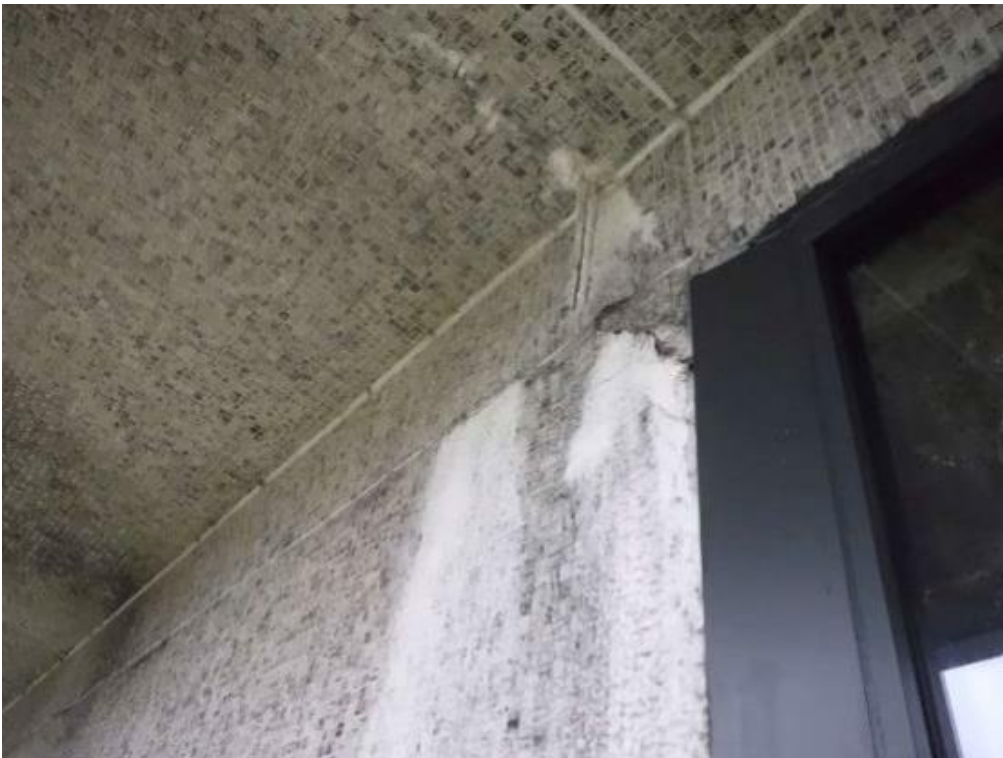
Photo B.66: A view showing a vertical crack in the west elevation of the West Machine Hall
