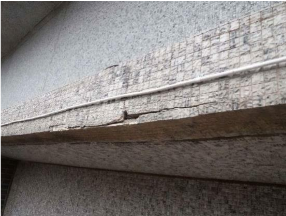
Photo B.88: A view showing a horizontal crack in the east elevation of the lower cantilever (East Machine Hall)
