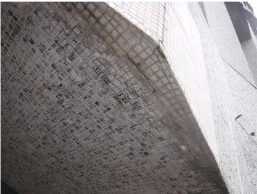
Photo B.36: A view showing a horizontal crack in the window reveal soffit of the east elevation (row BI storey 2)
