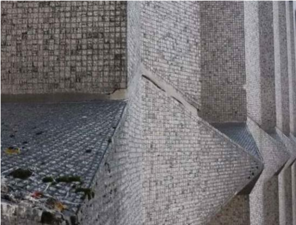
Photo B.23: A view showing de-bonded sealant to the east elevation (row O storey 12)
