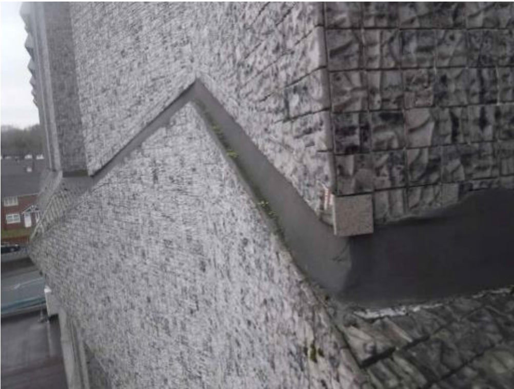
Photo B.41: A view showing a misaligned panel to the west elevation (row BM storey 4)
