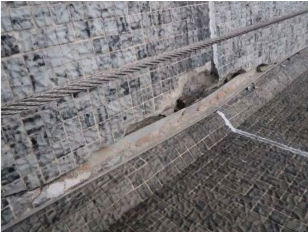
Photo B.83: A view showing an area of spalling to base of the mosaic panel (East Machine Hall, south elevation)
