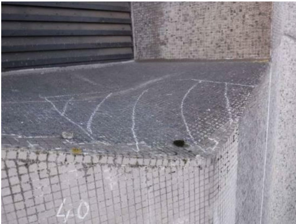
Photo B.25: A view showing an area of hollow sounding cladding with a vertical and horizontal crack in the east elevation (row D storey 2)
