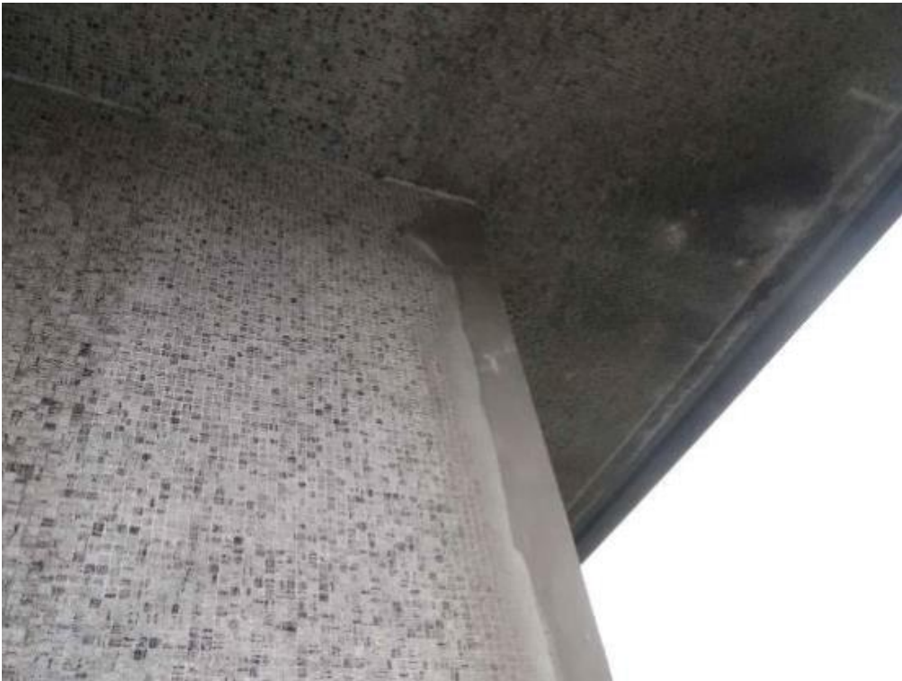
Photo B.47: A view showing a repaired vertical crack to the elevation (West machine hall north elevation)
