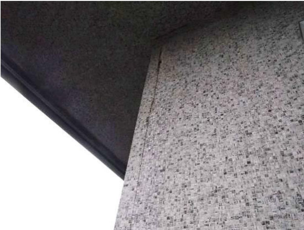
Photo B.87: A view showing a vertical crack in the east elevation of the East Machine Hall
