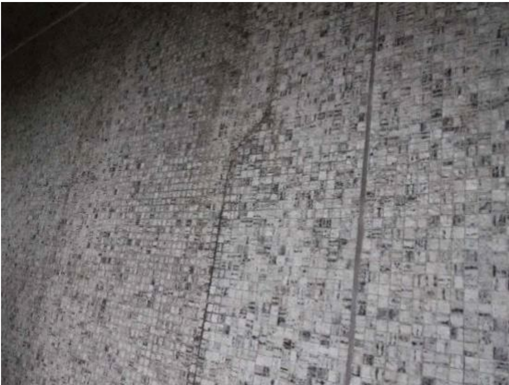
Photo B.48: A view showing a vertical crack in the north elevation of the West machine hall
