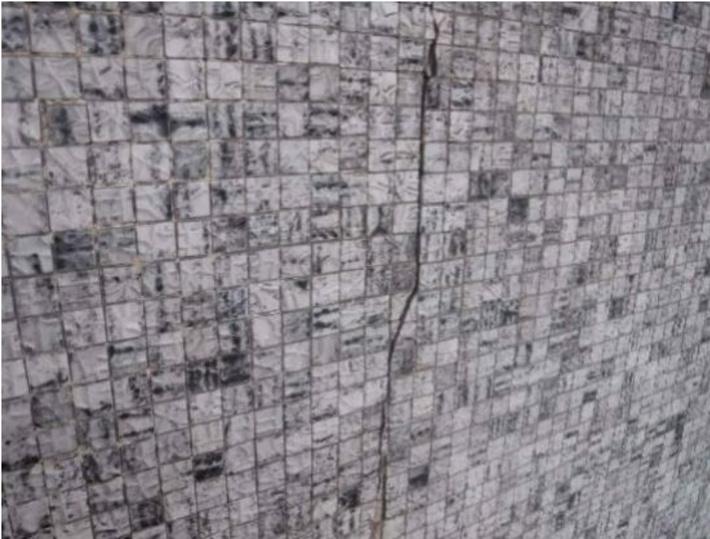
Photo B.17: A view showing a vertical crack in the internal face of the south entrance
