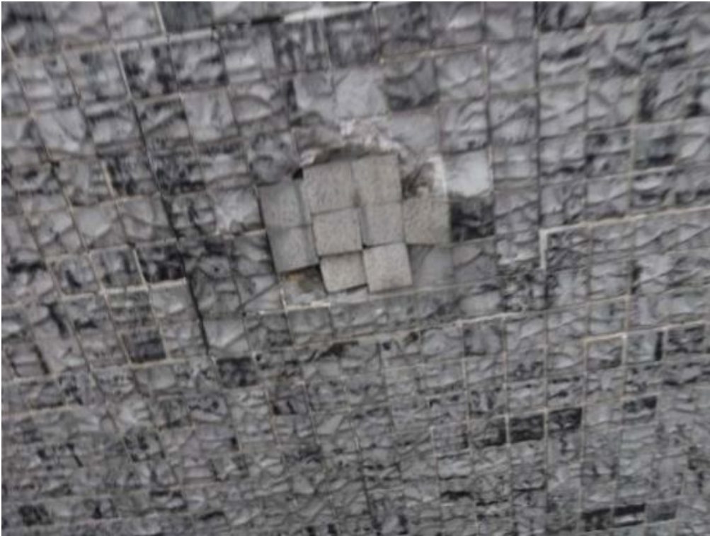
Photo B.13: A view showing a poor repair to the 6th storey of the south elevation
