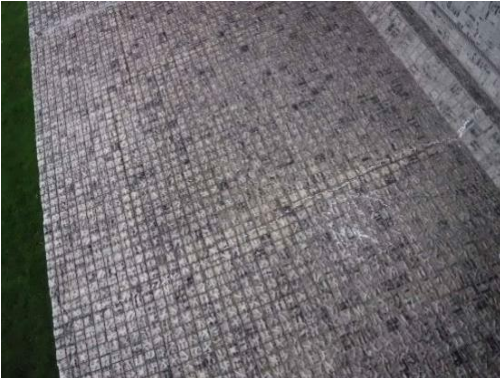
Photo B.59: A view showing a crack to the top face of the lower cantilever (West machine hall, south elevation)
