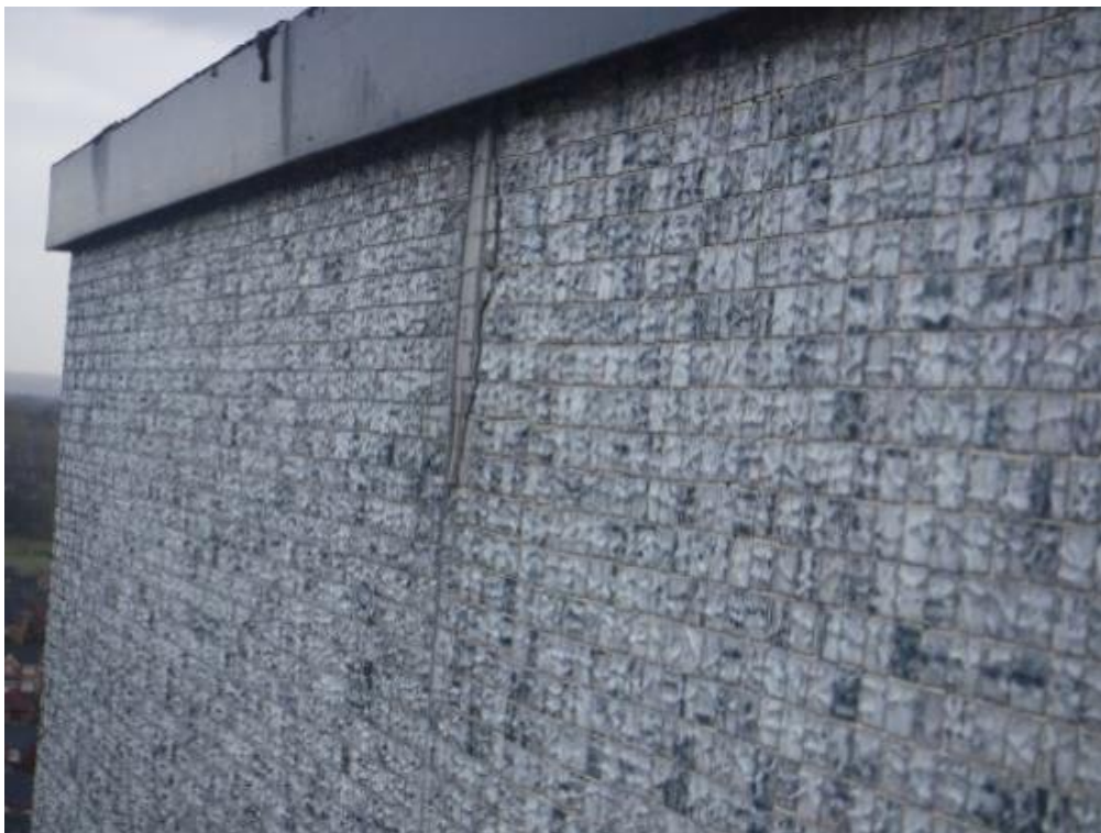
Photo B.6: A view showing a new vertical crack in the 12th storey of the north elevation
