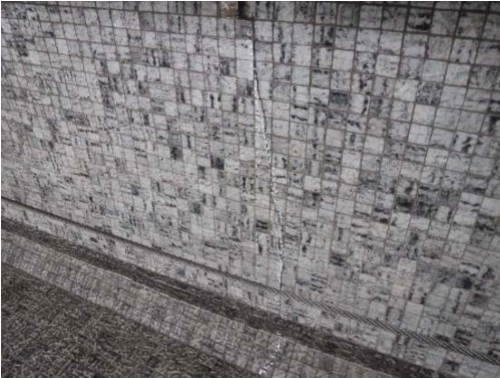
Photo B.69: A view showing a vertical crack in the west elevation (West Machine Hall)
