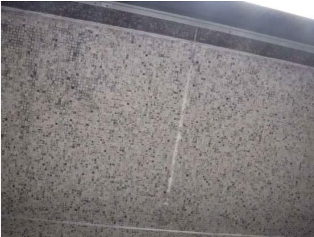
Photo B.46: A view showing a crack in the soffit of the upper cantilever (West machine hall north elevation)
