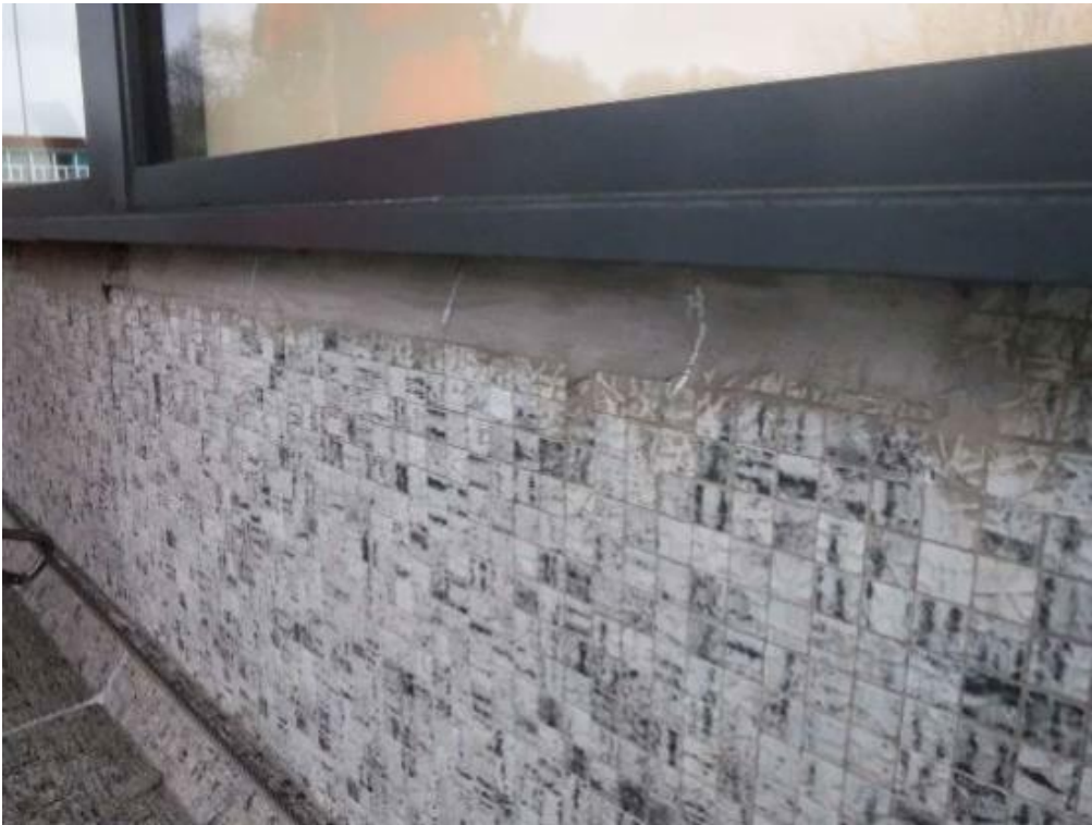
Photo B.61: A view showing vertical cracks in a repair below the window sill (West machine hall south elevation)
