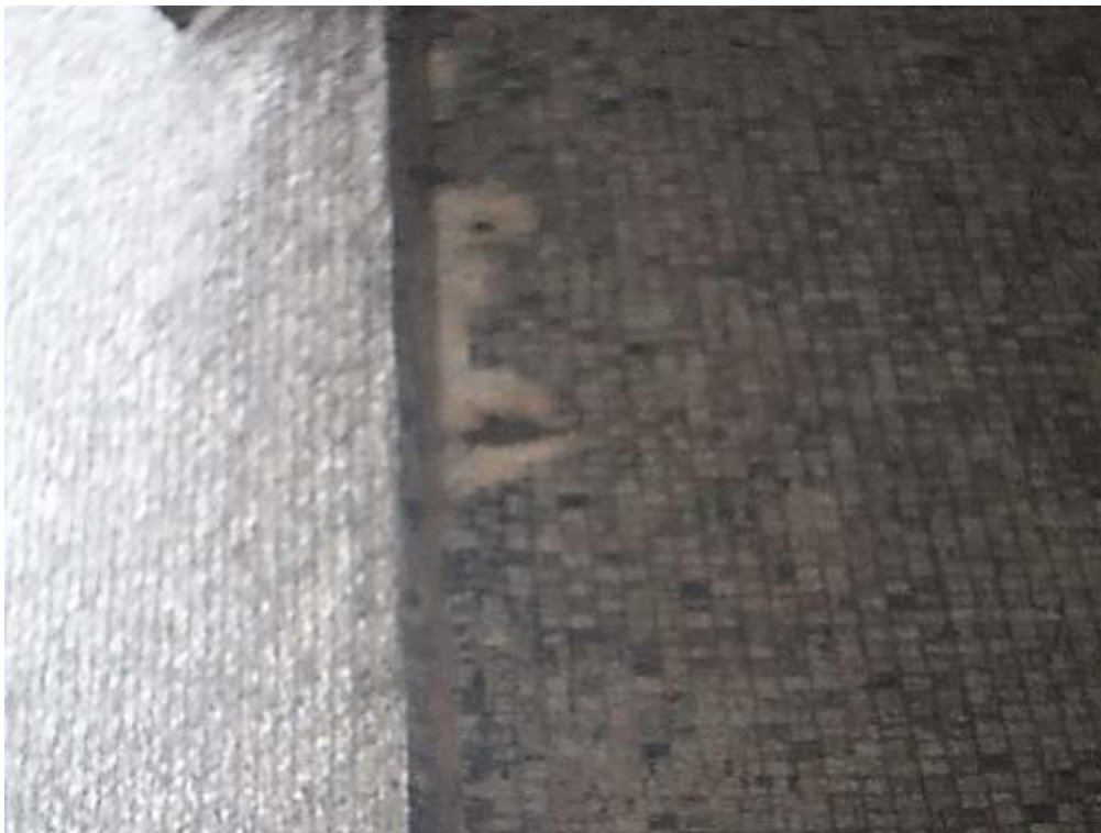
Photo B.21: A view showing an area of spalling with exposed reinforcement to the south entrance
