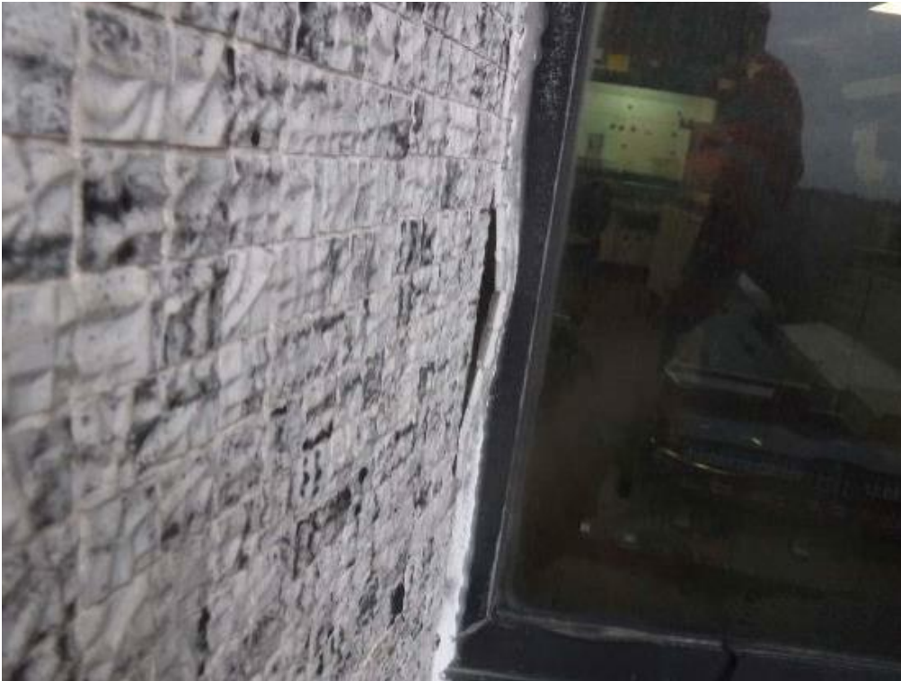
Photo B.43: A view showing loose tiles to the west elevation (row BQ storey 10)
