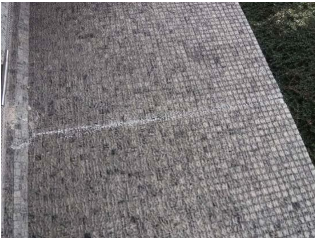
Photo B.82: A view showing a crack in the top face of the lower cantilever (East Machine Hall, south elevation)
