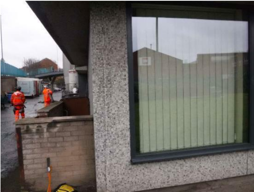
Photo B.71: A view showing a vertical crack to the elevation (West machine hall west elevation)
