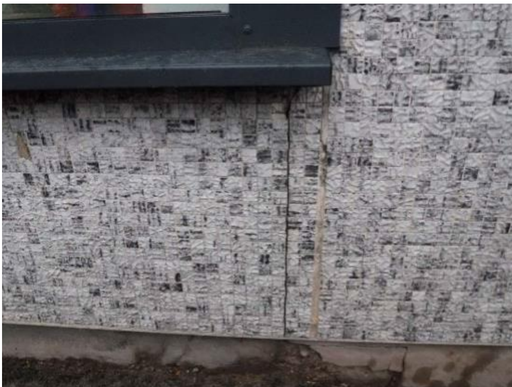
Photo B.81: A view showing a vertical crack in the south elevation of the East Machine Hall
