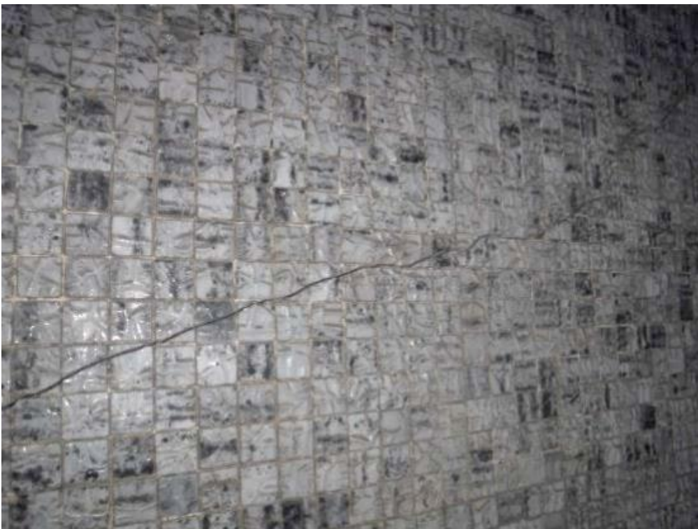
Photo B.20: A view showing a diagonal crack in the internal face of the south entrance
