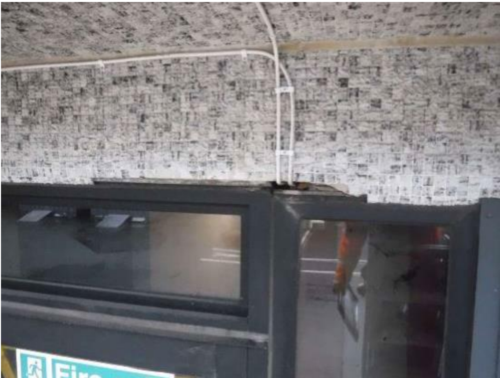
Photo B.76: A view showing an area of spalling above a window in the north elevation of the East Machine Hall
