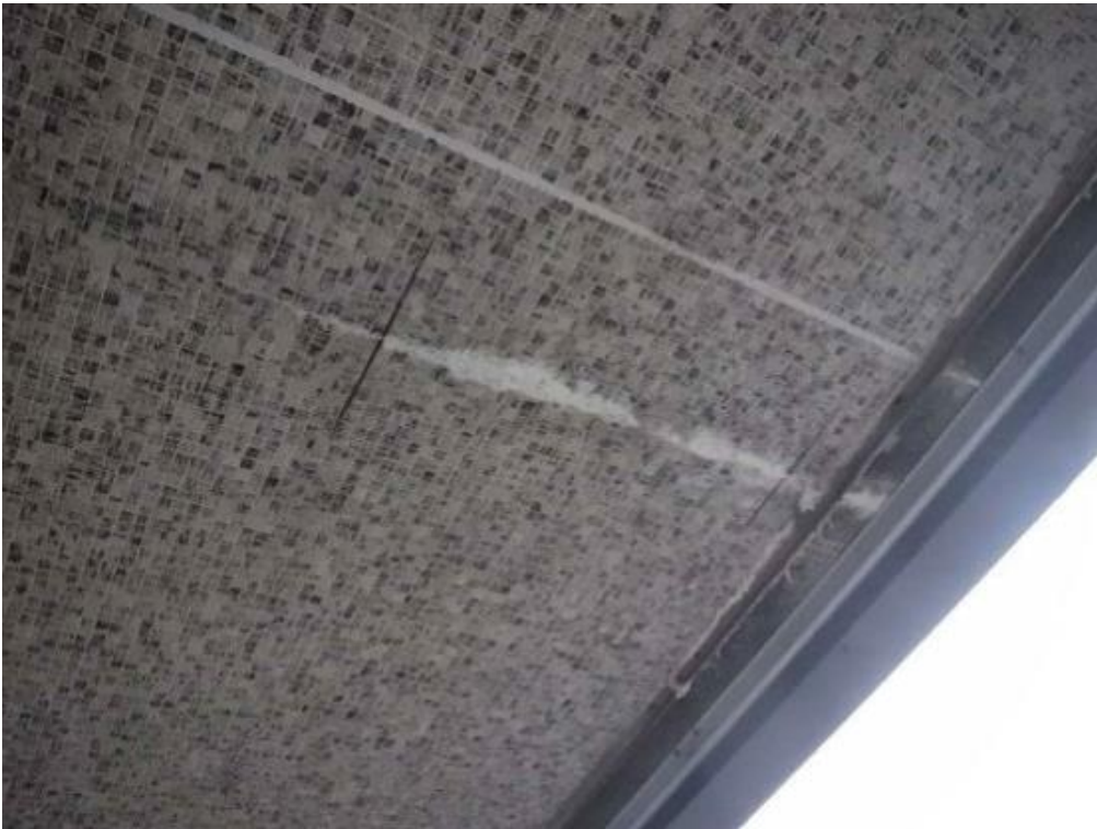
Photo B.85: A view showing a crack in the soffit of the upper cantilever of the East Machine Hall
