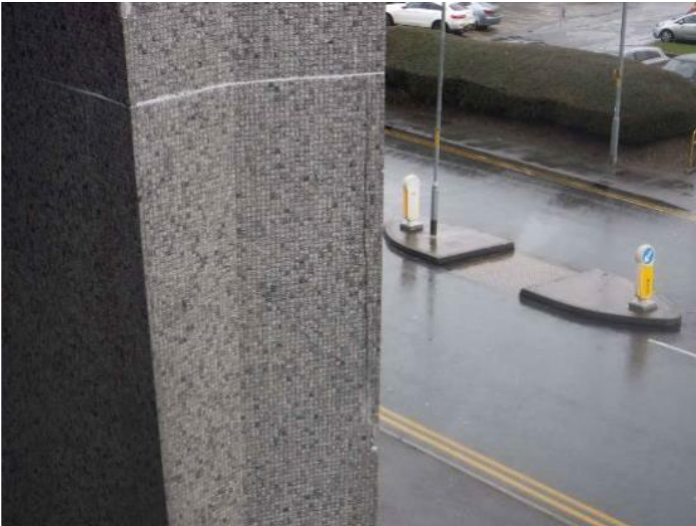
Photo B.40: A view showing a vertical crack in the west elevation (row BA storey 2)
