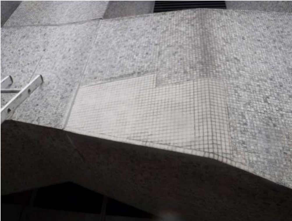
Photo B.39: A view showing hollow sounding repaired cladding (row BJ storey 2)
