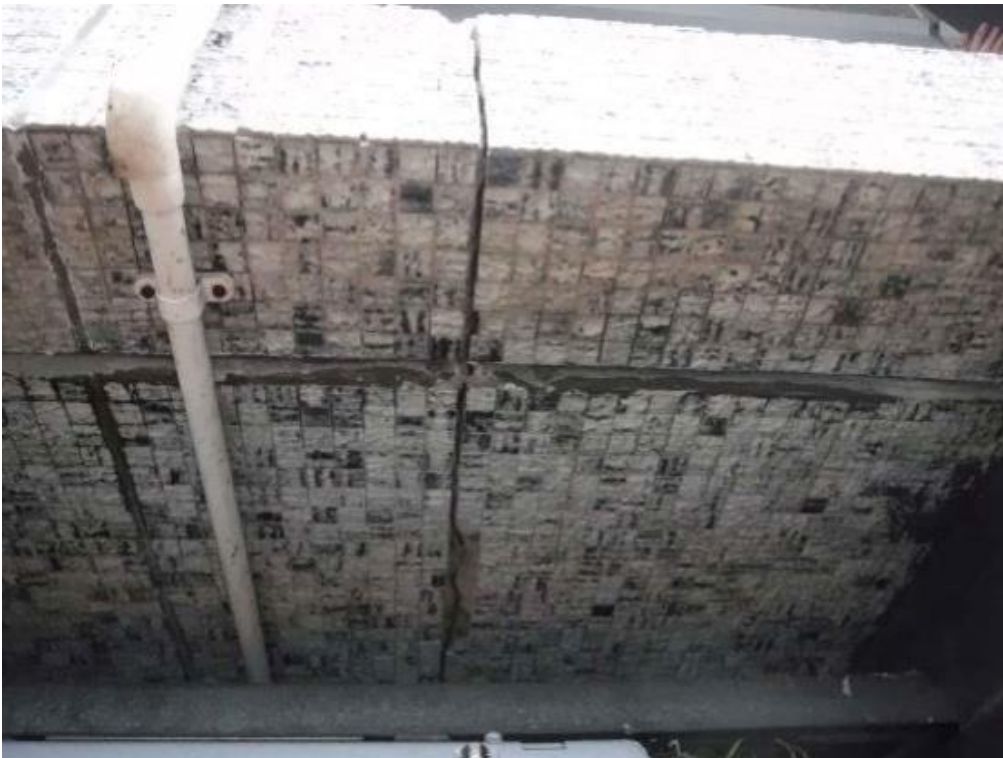
Photo B.52: A view showing a crack in the soffit of the lower cantilever (West machine hall north elevation)
