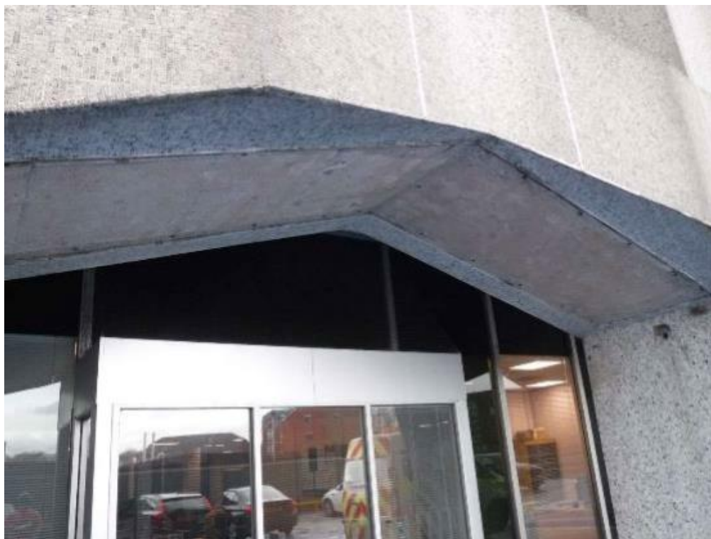
Photo B.30: A view showing missing cladding to the east elevation (row K storey 2)
