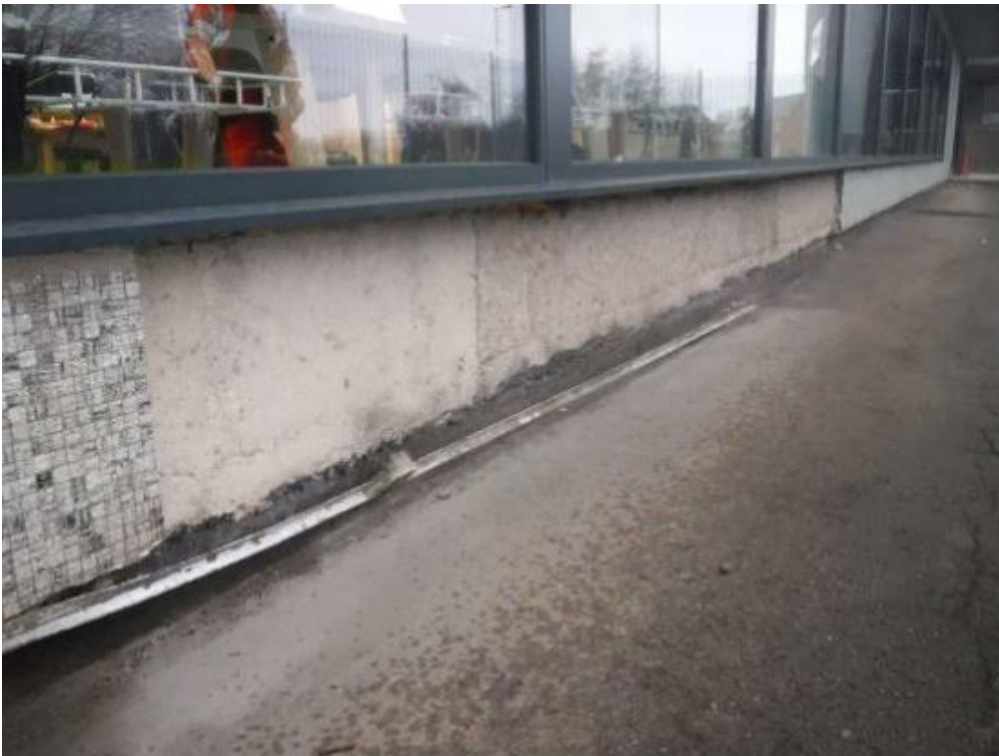
Photo B.64: A view showing a section of missing cladding to the south elevation of the West machine hall
