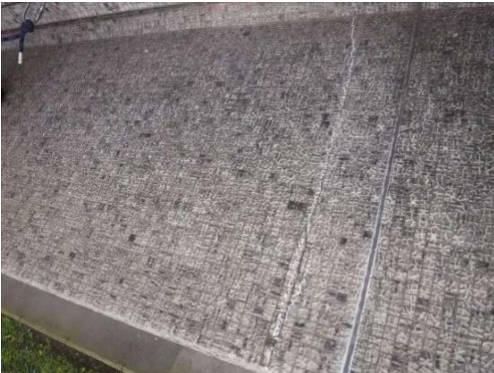
Photo B.68: A view showing a crack in the top face of the lower cantilever (West Machine Hall)
