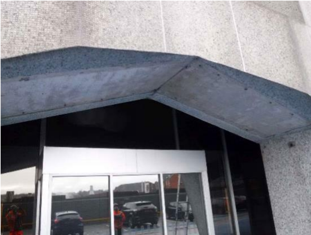
Photo B.31: A view showing missing cladding to the east elevation (row O storey 2)
