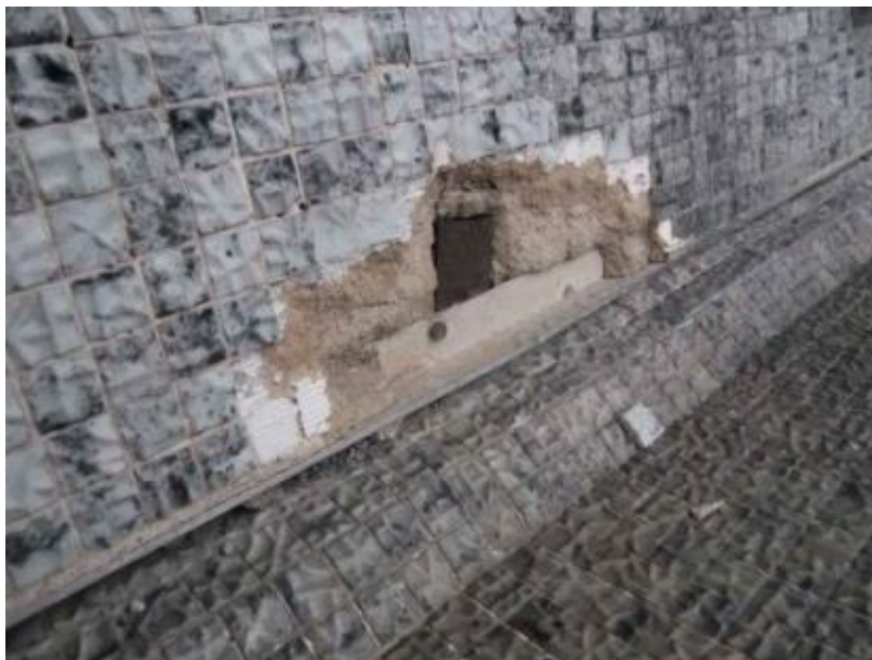
Figure 2.4: Area of spalling due to corrosion of an embedded steel object
