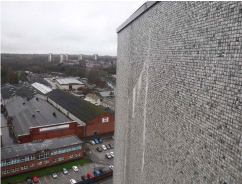
Photo B.14: A view showing a diagonal crack with leachate deposits to the 12th storey of the south elevation
