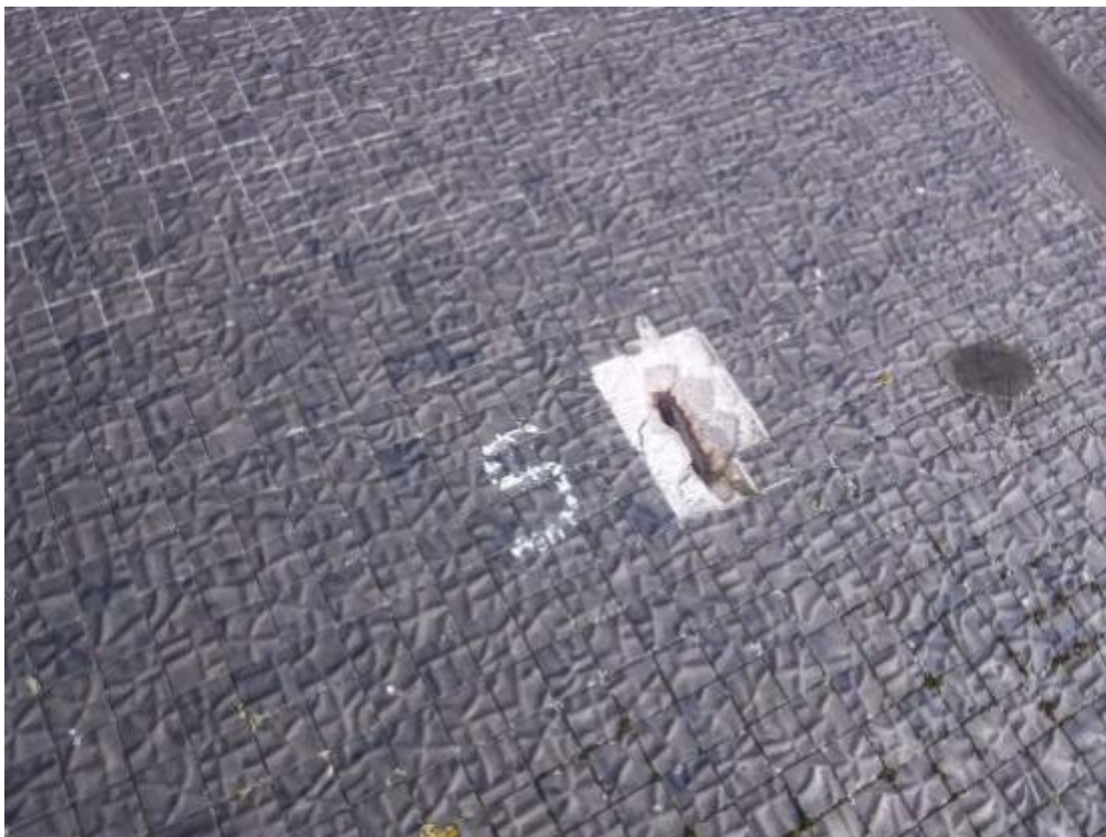
Photo B.22: A view showing an area of spalling with exposed reinforcement to the east elevation (row D storey 11)
