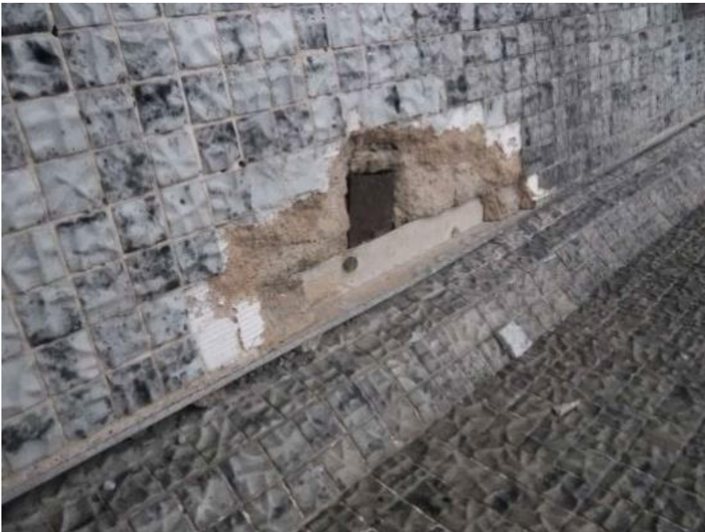
Photo B.84: A view showing a spall to the base of the mosaic panel (East Machine Hall, south elevation)
