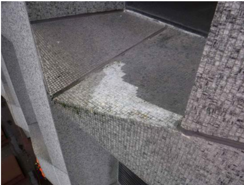
Photo B.34: A view showing missing tiles to the west elevation (row BL storey 4)
