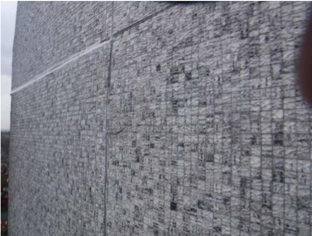
Photo B.7: A view showing a new horizontal crack to the 11th storey of the north elevation
