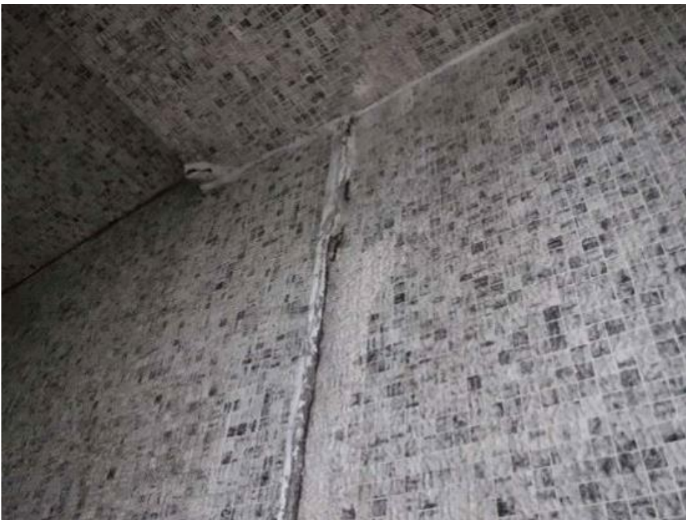
Photo B.78: A view showing de-bonded sealant in the south elevation of the East Machine Hall
