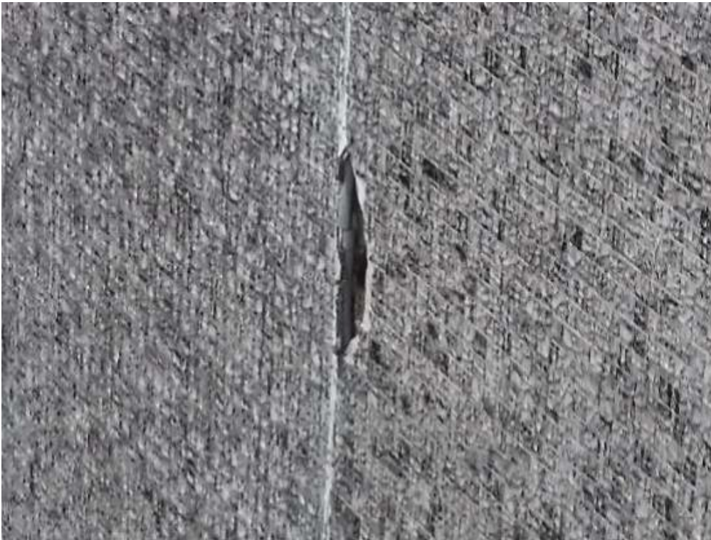
Photo B.15: A view showing an area of spalling with exposed reinforcement at a joint in the 7th storey of the south elevation
