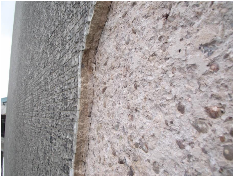
Figure 2.3: Failure of the cladding at the concrete-adhesive render interface
