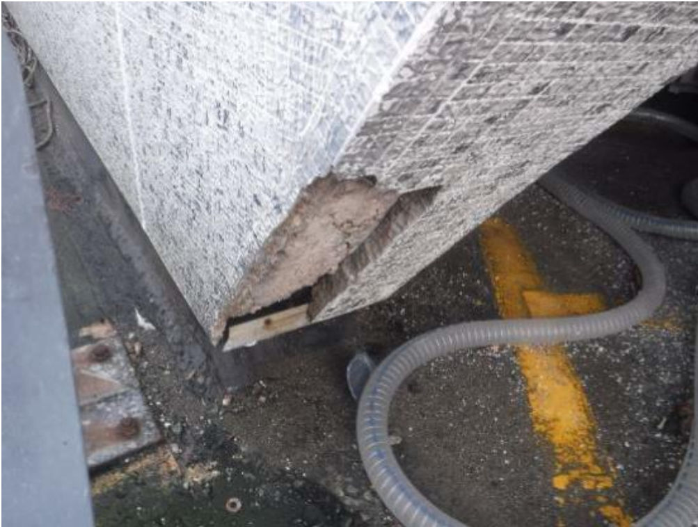
Photo B.9: A view showing a 'new' area of spalling at ground level in the north elevation
