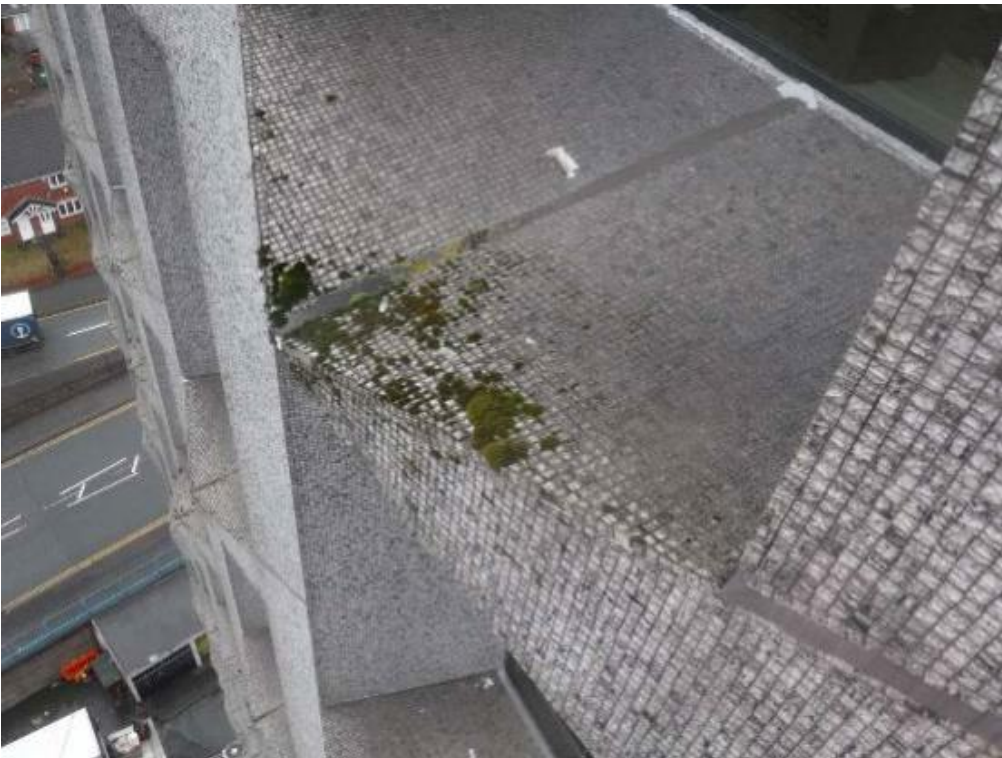
Photo B.42: A view showing moss growth to the west elevation (row BR storey 11)
