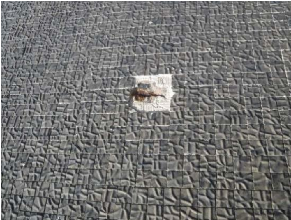
Photo B.28: A view showing spalling with exposed reinforcement to the east elevation (row S storey 6)
