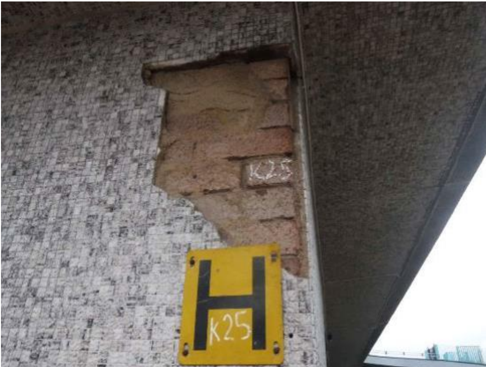
Photo B.89: A view showing spalled cladding on the east elevation of the East Machine Hall
