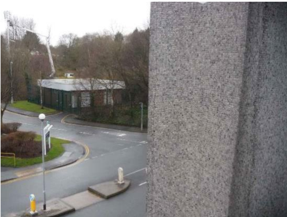
Photo B.24: A view showing a vertical crack with hollow sounding cladding to the east elevation (row X storey 2)
