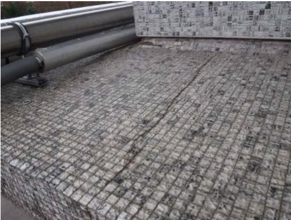
Photo B.74: A view showing a crack in the top of the lower cantilever (East Machine Hall, north elevation)
