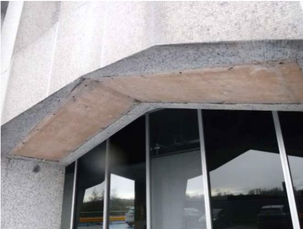
Photo B.32: A view showing missing cladding to the east elevation (row Q storey 2)
