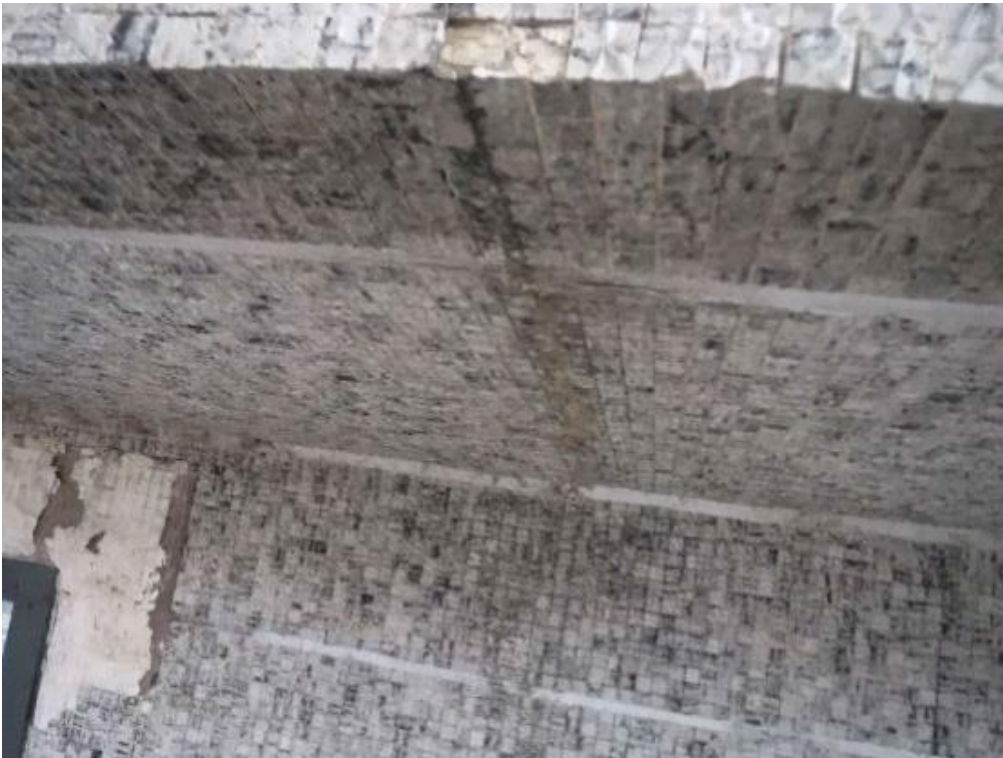
Photo B.75: A view showing a crack in the soffit of the lower cantilever (East Machine Hall, north elevation)
