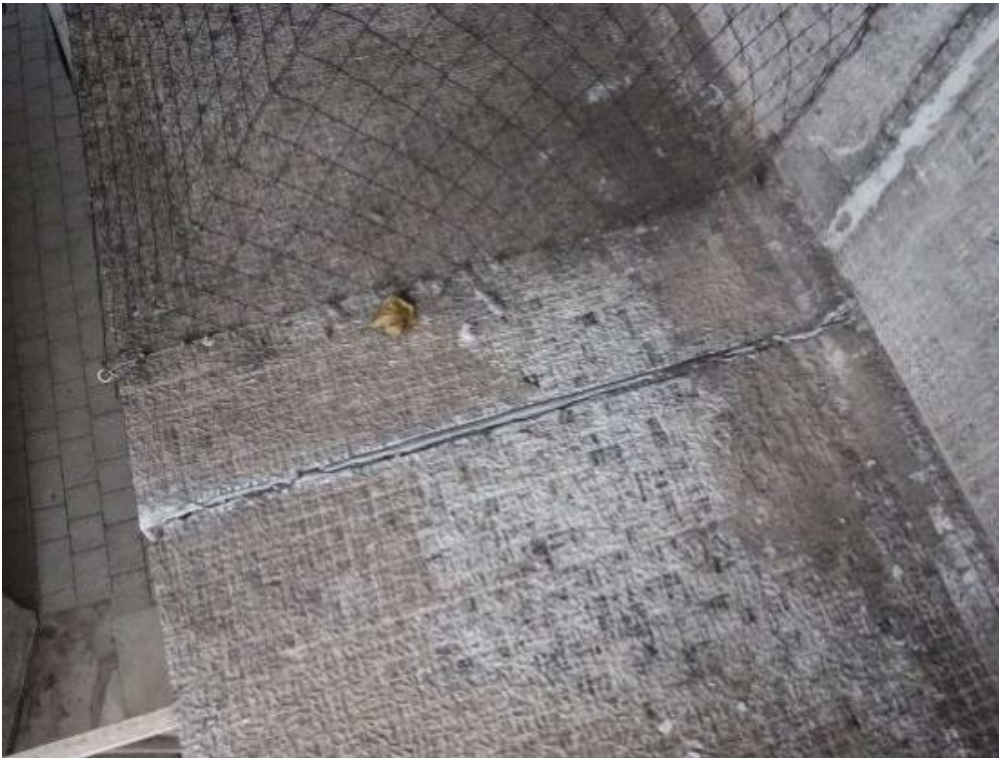
Photo B.79: A view showing de-bonded sealant in the top of the lower cantilever (East Machine Hall, south elevation)
