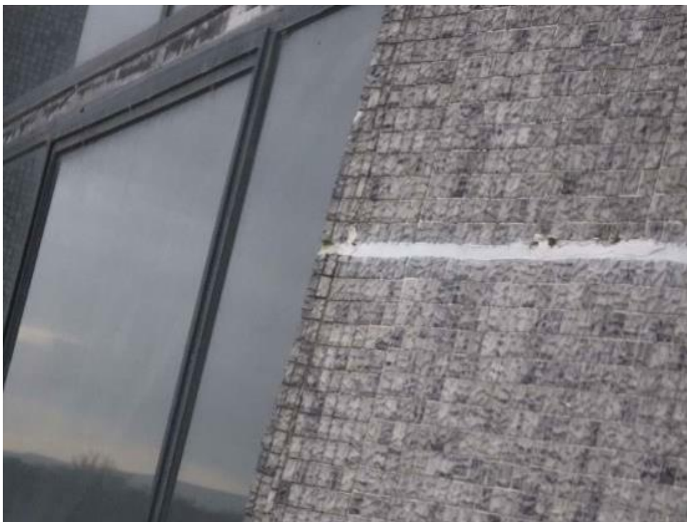
Photo B.5: A view showing a vertical crack to the 10th storey of the north elevation
