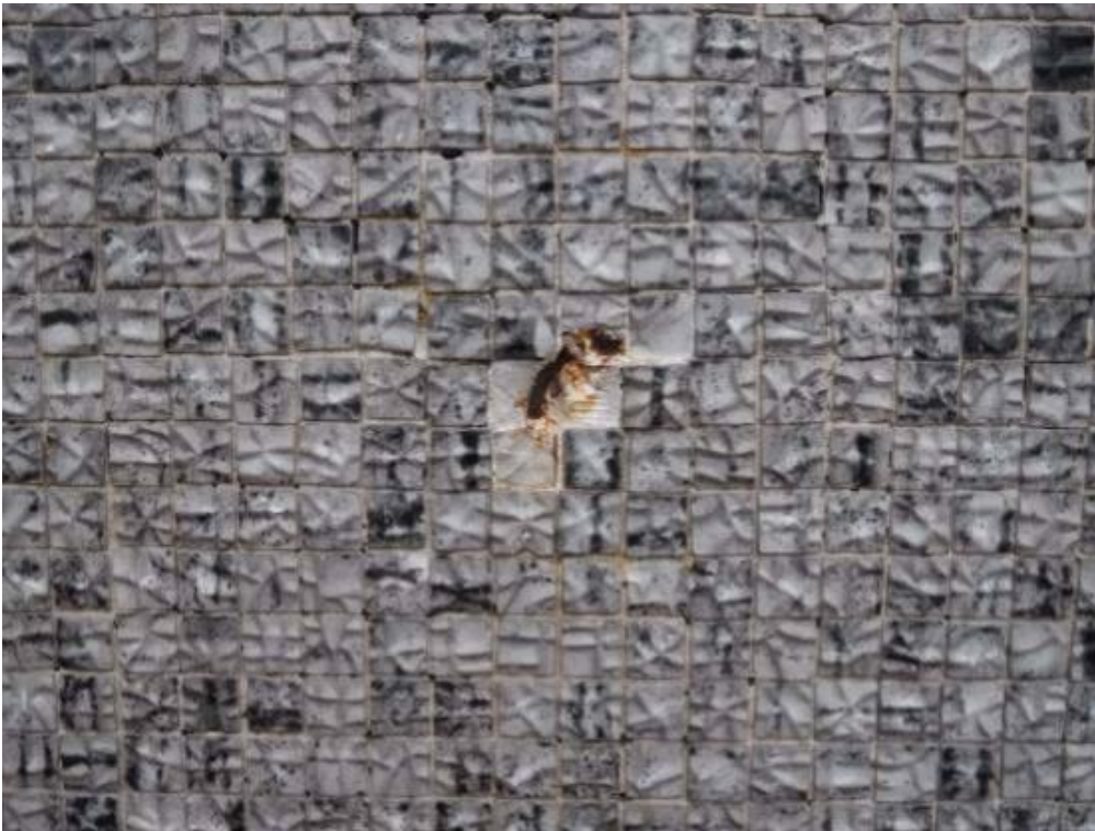
Photo B.11: A view showing an area of spalling with exposed steel in the 11th storey of the south elevation
