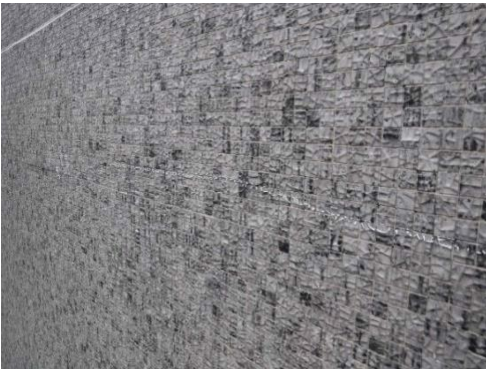
Photo B.18: A view showing a full width horizontal crack in the 10th storey of the south elevation
