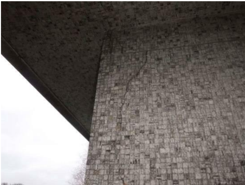
Photo B.55: A view showing a diagonal crack in the south elevation (West machine hall)
