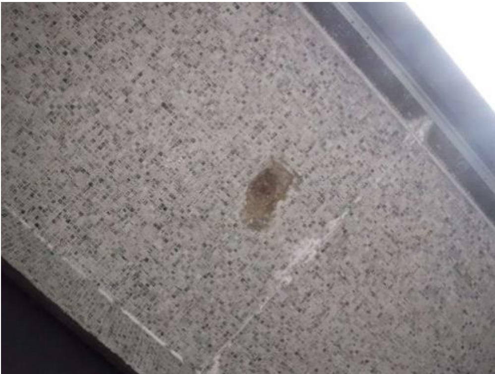
Photo B.50: A view showing spalling to the soffit of the upper cantilever (West machine hall north elevation)
