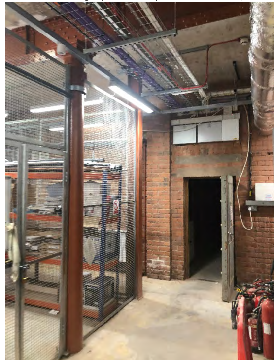
Figure 3.39 Photo of Room B1.01 Basement Storage area (Source : Photograph taken by author, 21/03/21)
