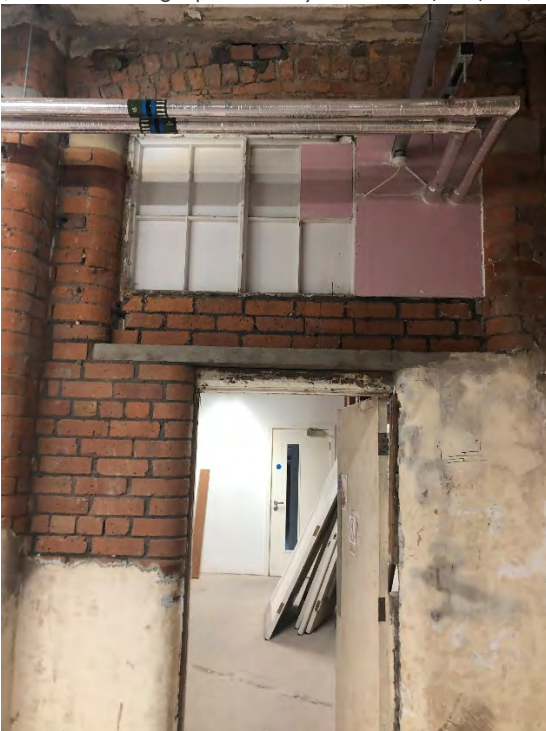
Figure 3.38 Photo of Room B1.01 Basement Storage area (Source : Photograph taken by author, 21/03/21)
