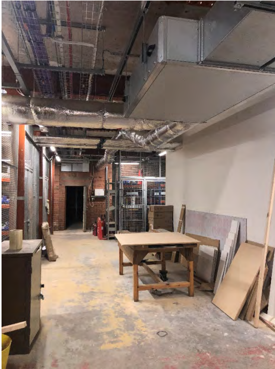
Figure 3.36 Photo of Room B1.01 Basement Storage area (Source : Photograph taken by author, 21/03/21)
