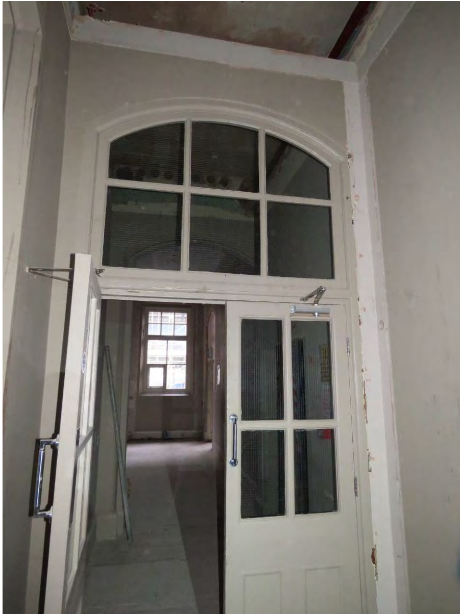
Figure 120: An example of an original pair of glazed timber corridor doors and fanlight which have been removed from their original location and repositioned. The doors and fanlight will be retained and redecorated as part of the consented scheme.
