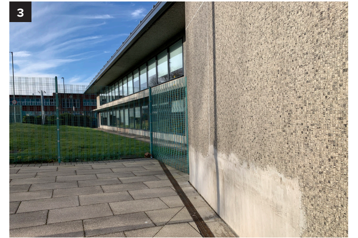
Existing condition of mini-mosaic tiles to south elevation at ground level
